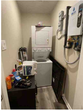
Unit B Utility
