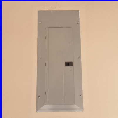
Main panel in garage
