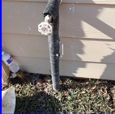
Main water shutoff
