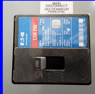
200 amp main service disconnect in garage
