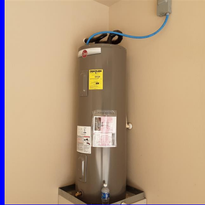
Water heater in garage
