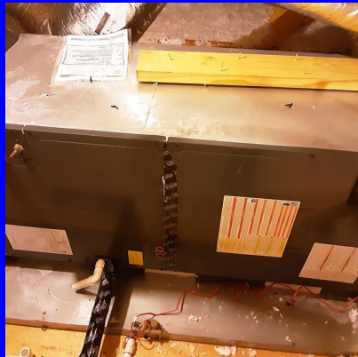
Goodman furnace in attic
