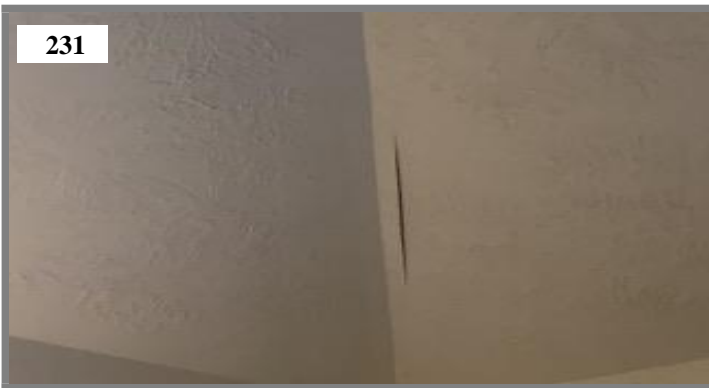
loose ceiling seam upstairs left
