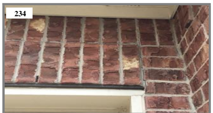
mortar crack over garage
