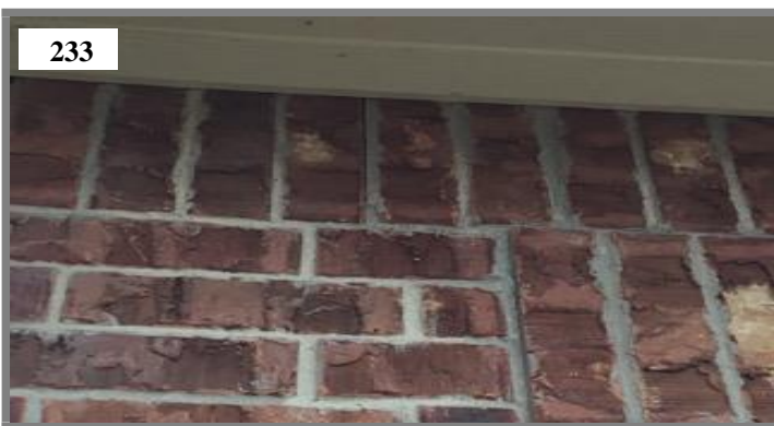
mortar crack over garage
