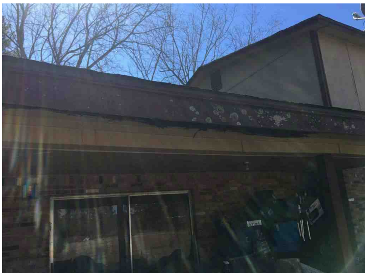
Rotten Fascia and Cornice
