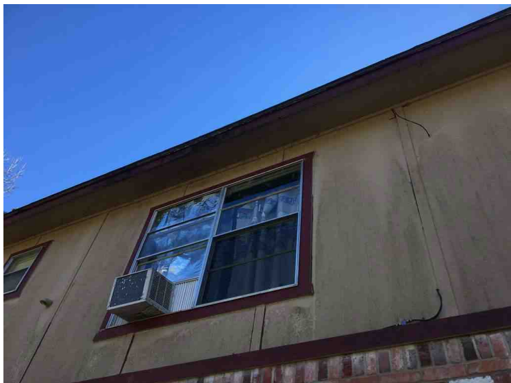
Rotten Fascia Board
