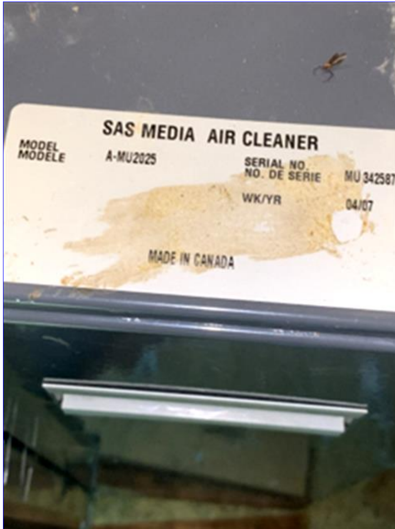
C. Photo 3(Picture) The filter location is in the attic.
