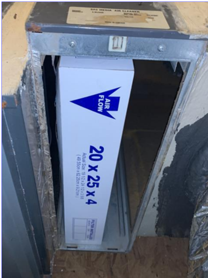
C. Photo 4(Picture) The currently installed filter is under-sized. Recommend correction.
