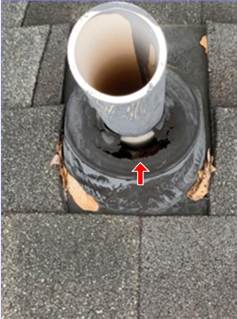
C. Photo 4(Picture) Damage was observed on one of the plumbing vent pipe boots. Recommend all vent pipe boots be resealed and/or replaced to prevent water intrusion and damage.
