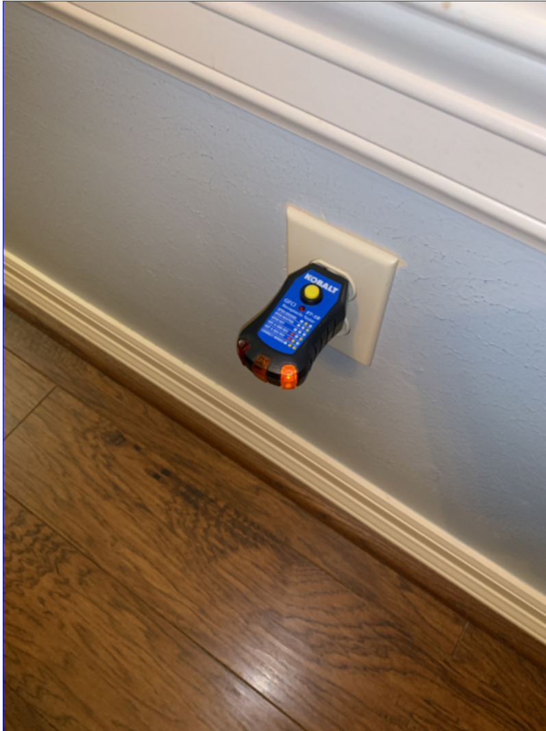
B. Photo 2(Picture) In the front bedroom, on the exterior wall, the outlet has a bad top receptacle. Recommend replacement.
