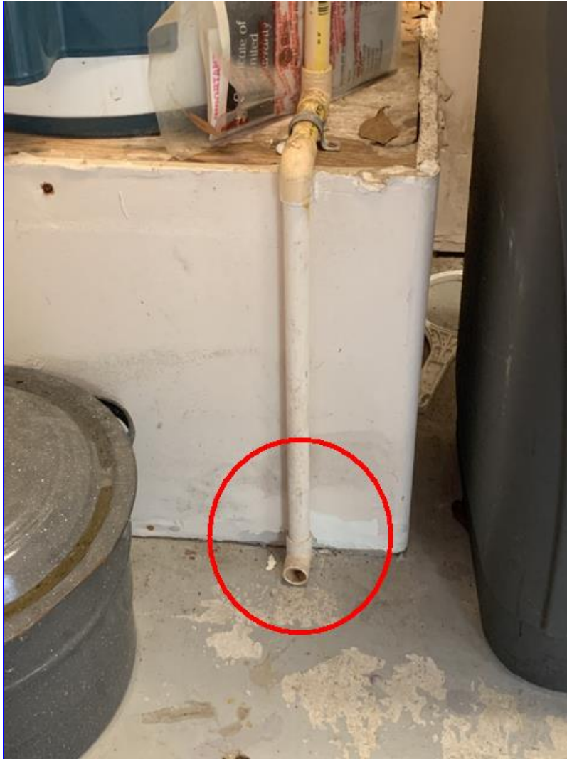
C. Photo 2(Picture) The T&P (Temperature and Pressure) relief valve piping on water heater, should extend to within 6 inches of the floor and should be pointed downward for safety.
