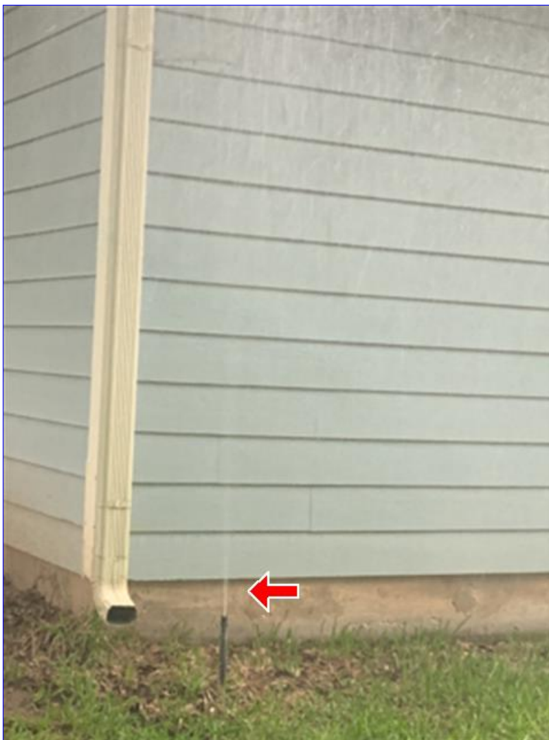
E. Photo 1(Picture) A damaged sprinkler head nozzle was observed in Zone 3.
