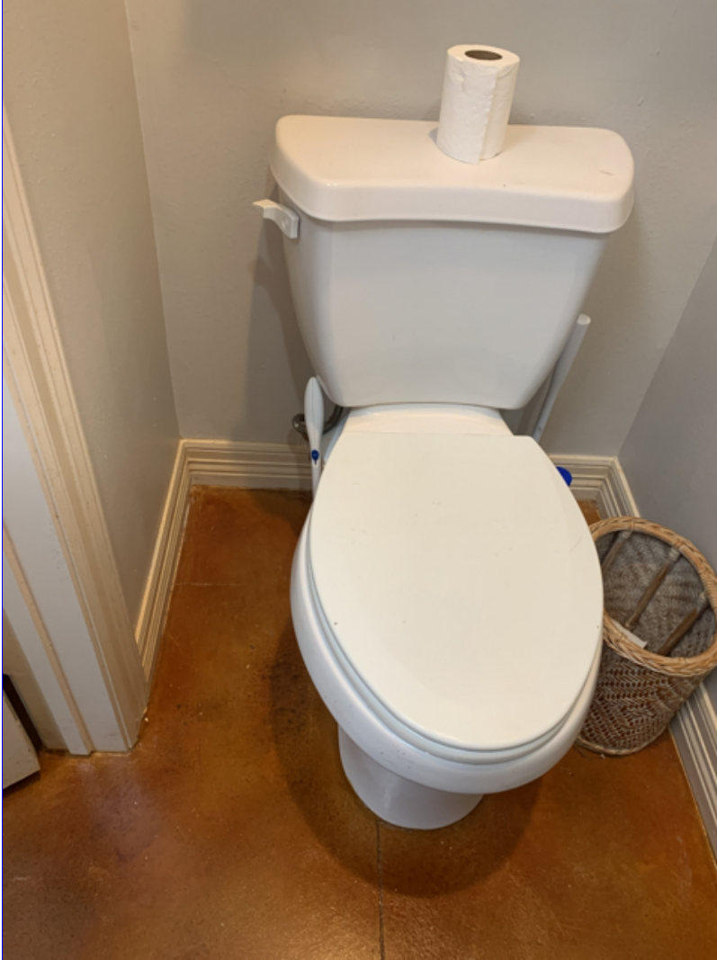
A. Photo 1(Picture) Two toilets are loose at floor. Repairs may involve re-setting the toilet on a new wax seal. I recommend a qualified licensed plumber repair or correct as needed.
