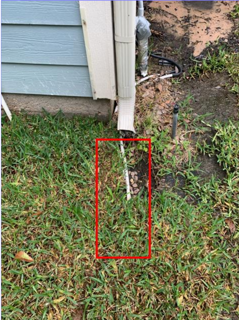
B. Photo 1(Picture) Concrete splash blocks or downspout extensions, are absent at some gutter downspouts. Gutter downspouts should discharge a minimum of 18" away from the foundation.
