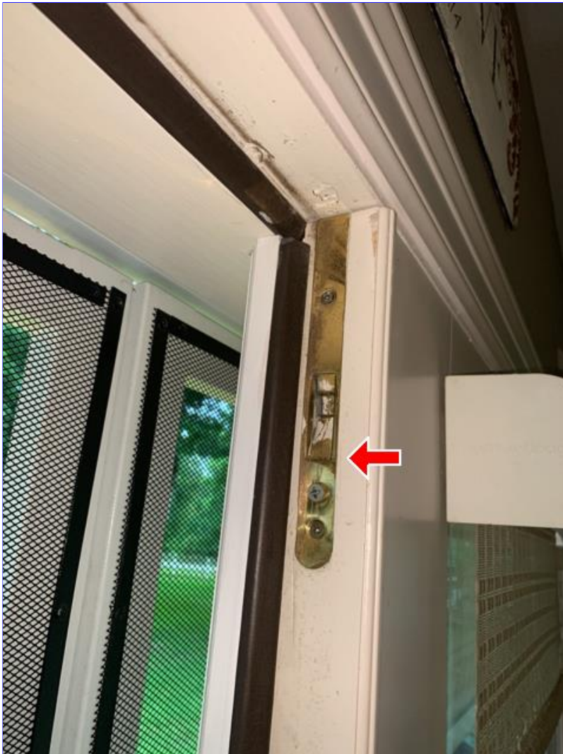
G. Photo 2(Picture) The back exterior double door slide latches are damaged and inoperable.
