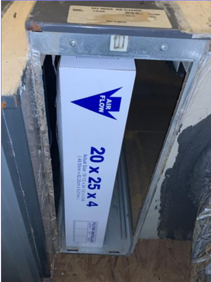
C. Photo 2(Picture) The filter location is in the attic.
