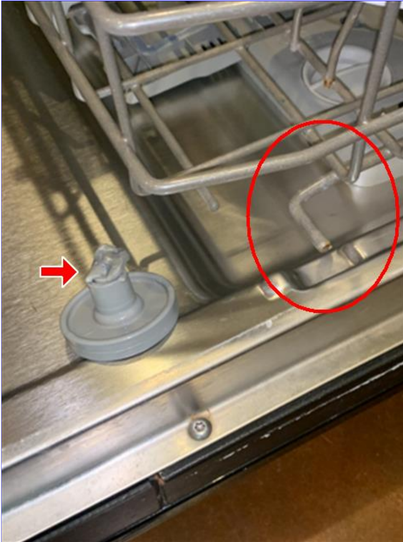
A. Photo 1(Picture) The bottom rack front right wheel is damaged. Recommend replacement as needed.
