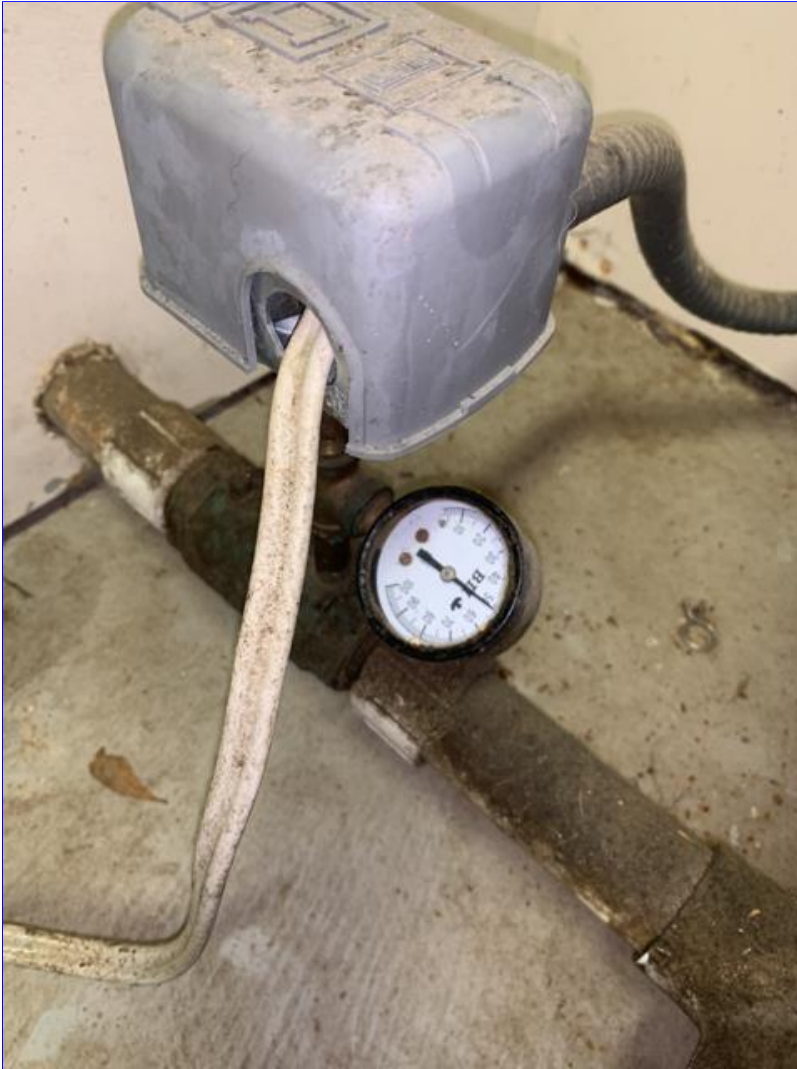
B. Photo 2(Picture) The pressure gauge near the pressure switch is not registering properly. Recommend replacement.
