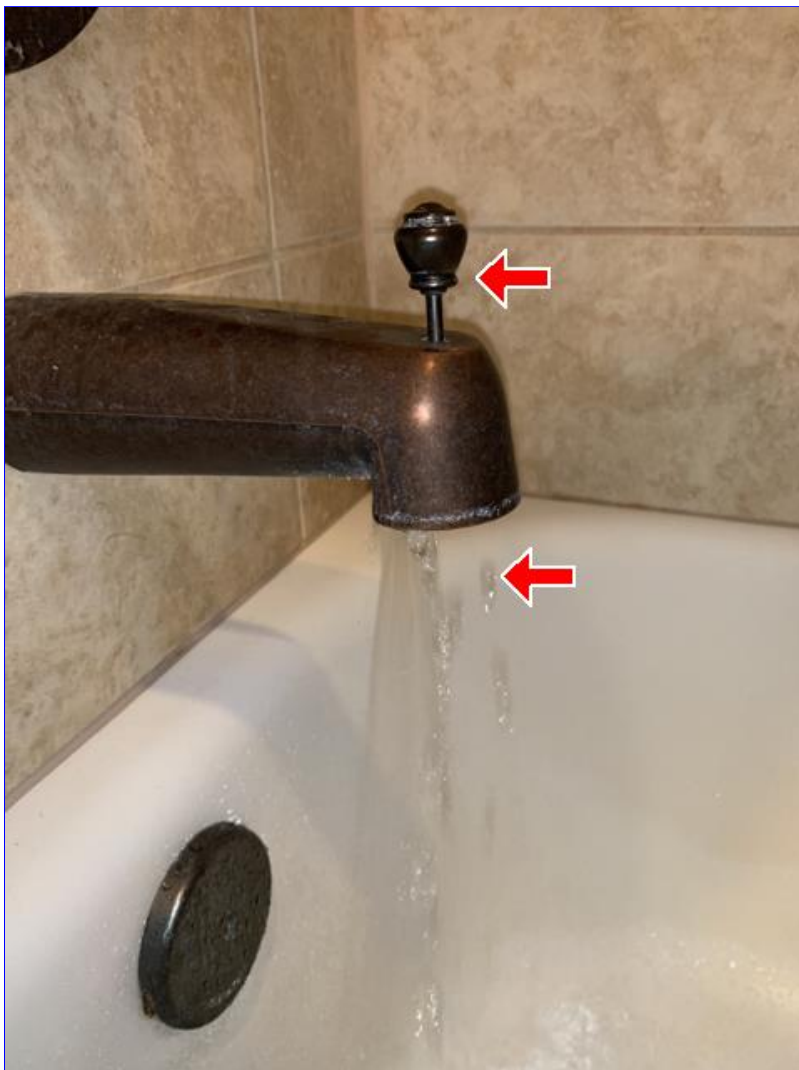
A. Photo 4(Picture) Water does not fully divert from tub spigot to shower head in some bathrooms. Recommend correction.
