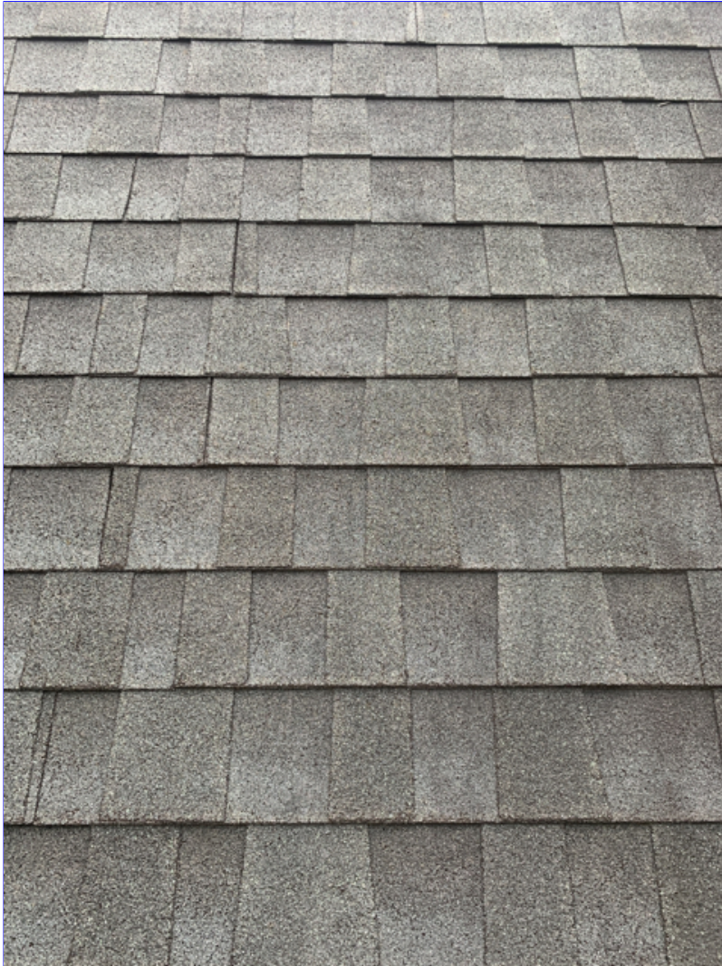
C. Photo 1(Picture) This roof covering is probably around 14 years old. This type of architectural style composition shingles typically lasts about 20 years in this climate.
