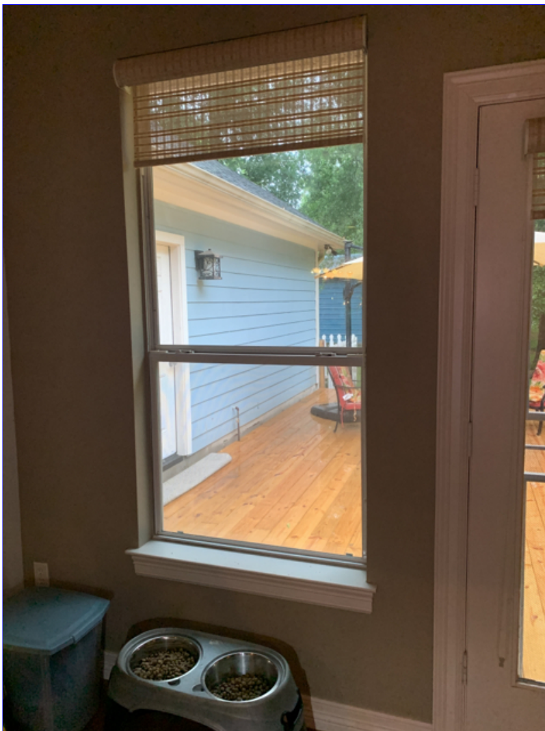
H. Photo 2(Picture) In the back enclosed sitting room/ office, the window springs on the left window have failed.
