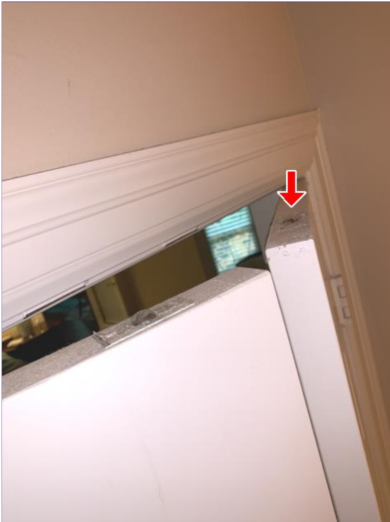
G. Photo 3(Picture) The ball catch hardware at the top of interior double doors are damaged, missing, or out of adjustment. Recommend correction.
