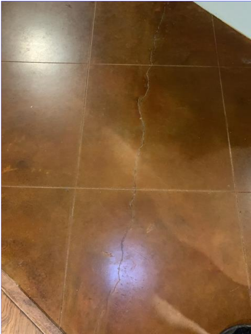
A. Photo 3(Picture) Some concrete surface cracks were observed in the interior stained concrete floors. There is little to no deflection across the cracks. This type of flexural crack is generally the result of seasonal variations in soil moisture causing the soils to shrink and/or swell exerting pressure on the foundation. This type of crack is not structurally significant.
