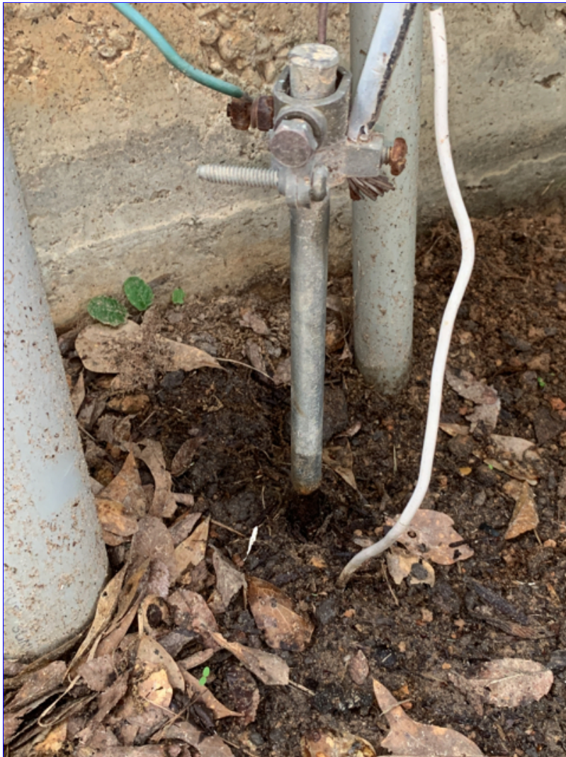
A. Photo 1(Picture) The system ground rod (electrode), is corroded. Recommend replacement.
