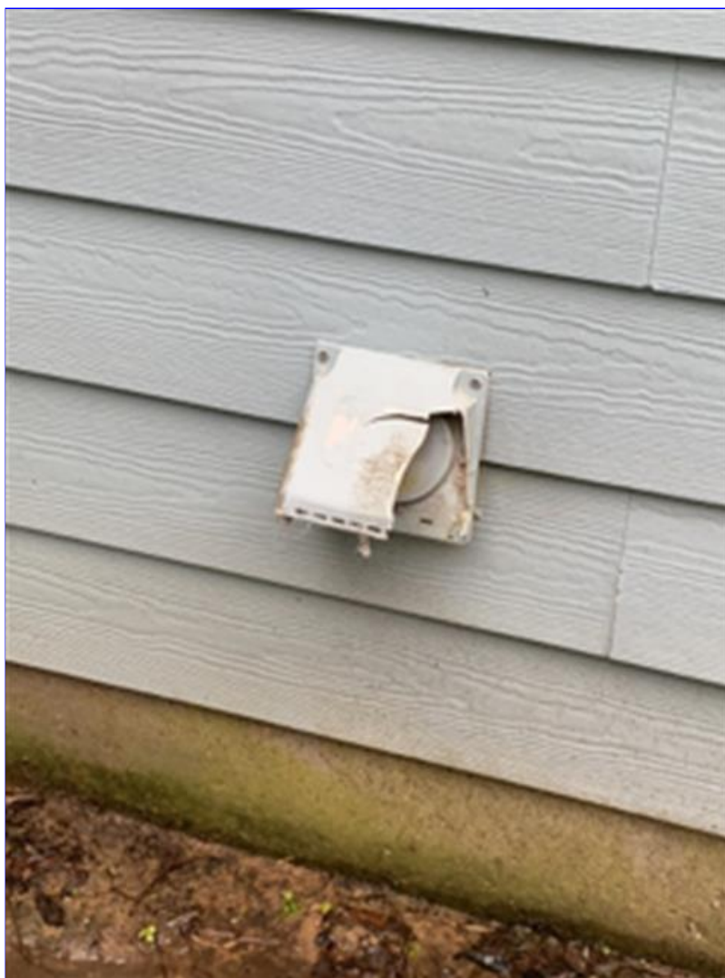
H. Photo 1(Picture) The dryer exhaust exterior cover is damaged. Recommend correction as needed.
