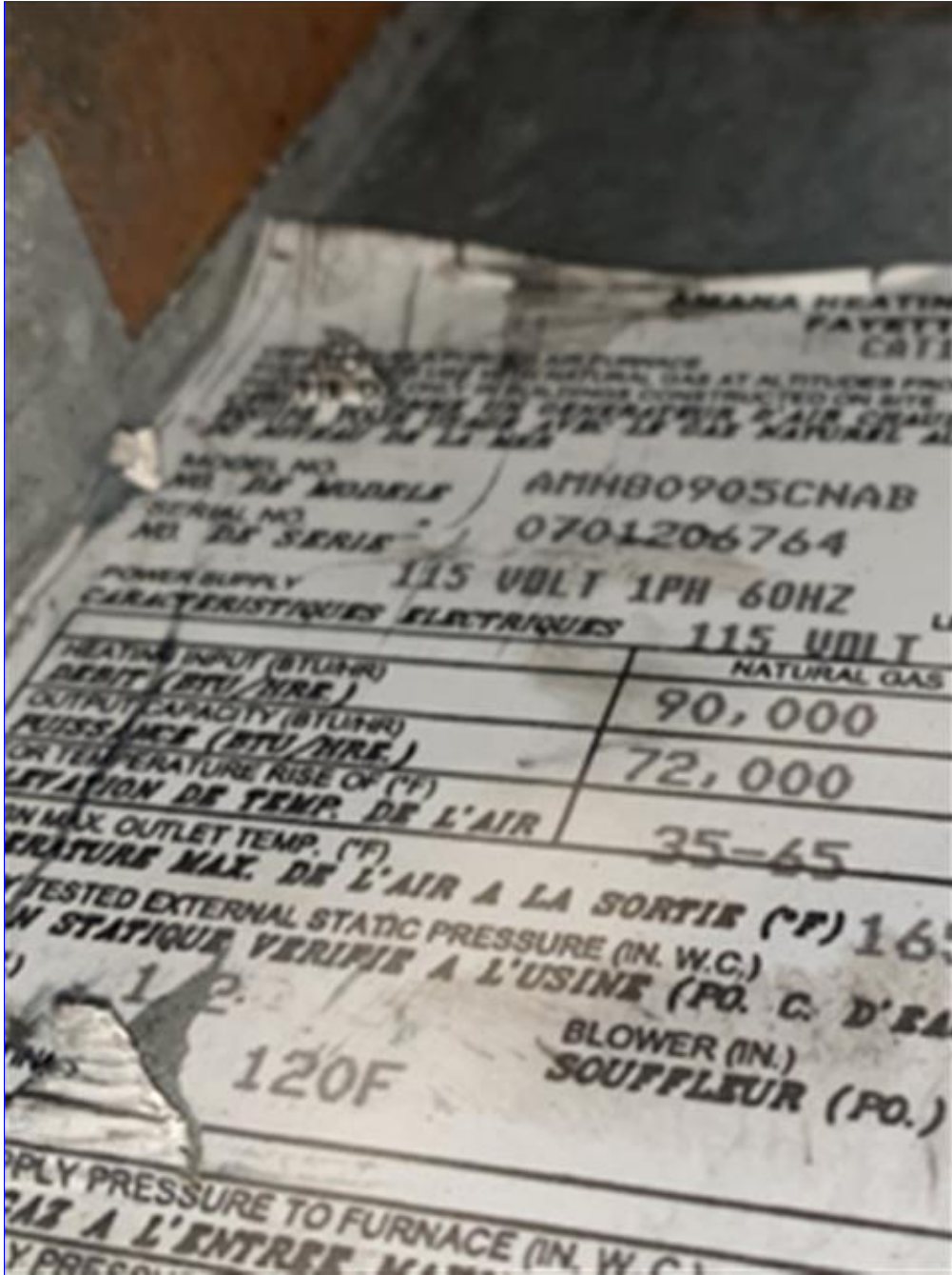
A. Photo 2(Picture) Furnace service tag.
