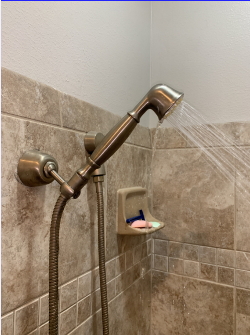
A. Photo 3(Picture) Shower head leaks were observed in some bathrooms.
