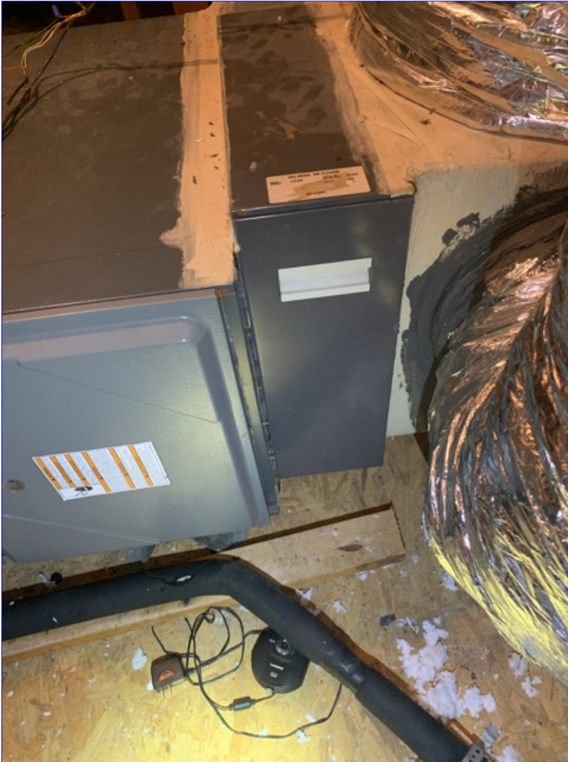
C. Photo 1(Picture) The filter location is in the attic.
