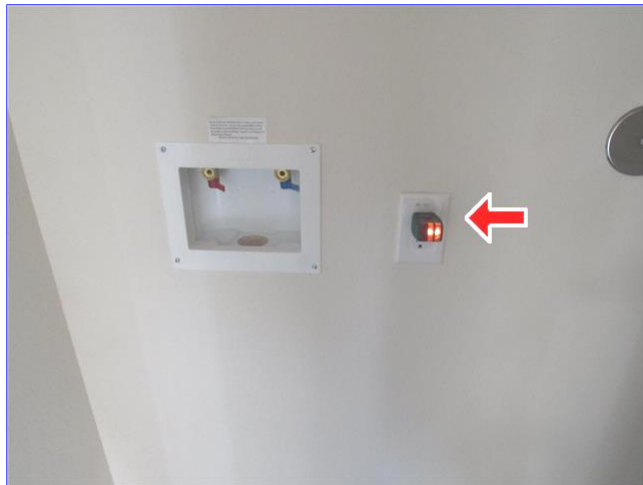
B. Item 1(Picture) no GFCI for plugs in utility room - recommend adding for safety - required by present code
