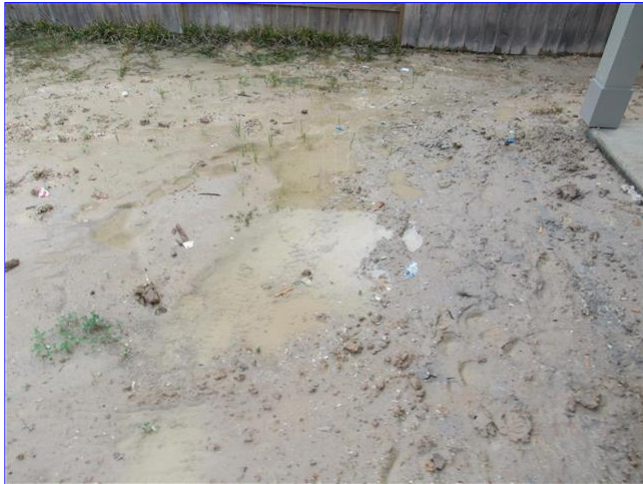
B. Item 3(Picture) grade appeared to be holding water in some places on January 25 - recommend evaluation by professional contractor/landscaper to drain properly in swales to street
