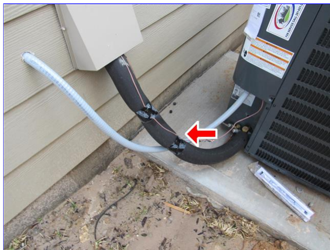
B. Item 1(Picture) no UV wrap for insulation for suction line at exterior ac unit - recommend adding to prevent damage to insulation
