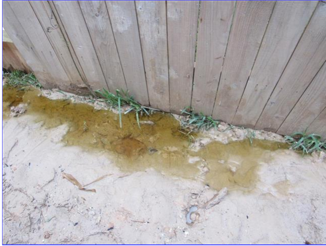
B. Item 1(Picture) grade appeared to be holding water in some places on January 25 - recommend evaluation by professional contractor/landscaper to drain properly in swales to street
