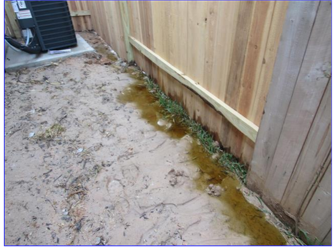
B. Item 2(Picture) grade appeared to be holding water in some places on January 25 - recommend evaluation by professional contractor/landscaper to drain properly in swales to street
