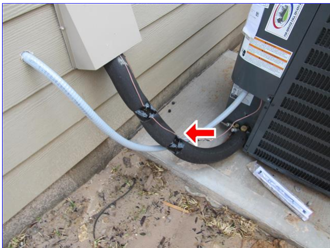
B. Item 1(Picture) no UV wrap for insulation for suction line at exterior ac unit - recommend adding to prevent damage to insulation
