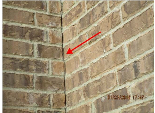
Corner area along front wall not sealed
