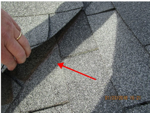
Lack of adhesion at the front valley
