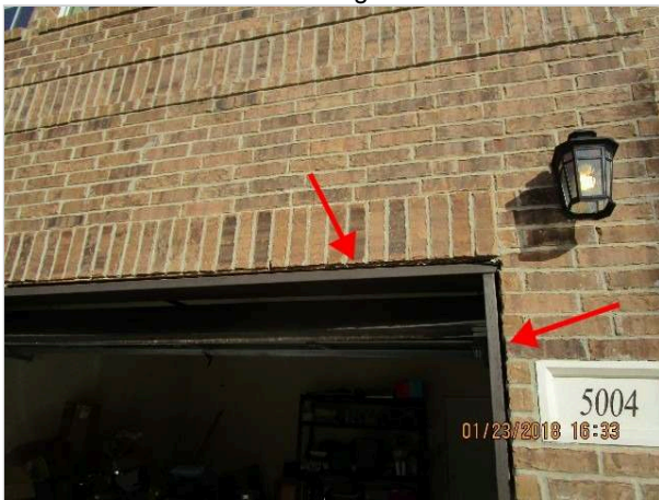
Area between the garage trim board and brick wall not sealed
