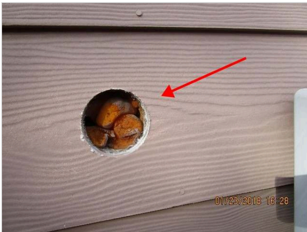
Hole in right exterior wall
