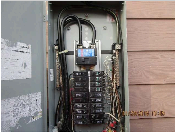
Cover removed for inspection
