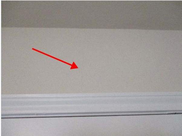
Sheetrock crack in left rear bedroom
