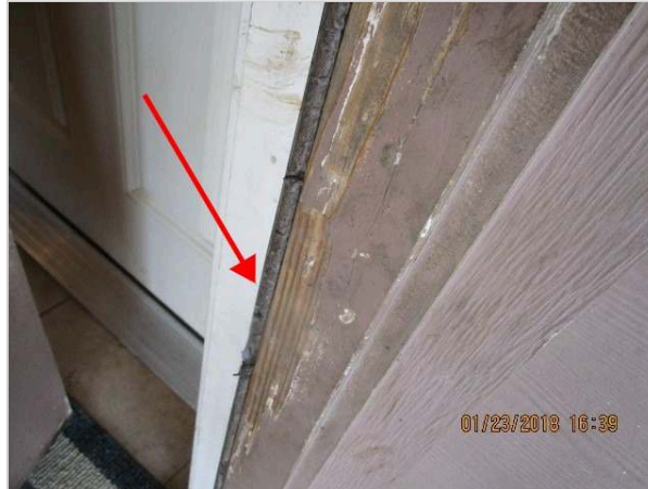
Damaged weather stripping
