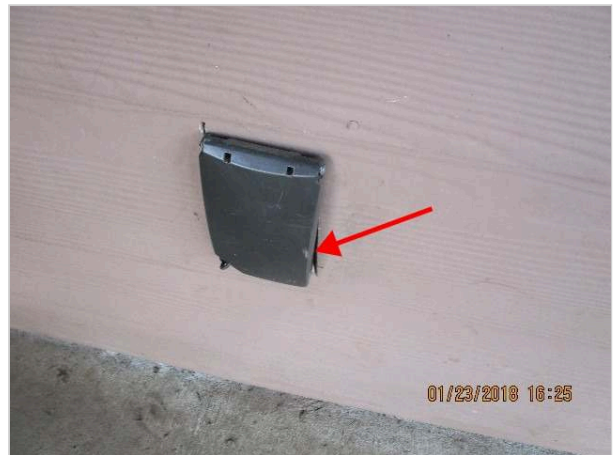
Gap in wall / Needed sealed
