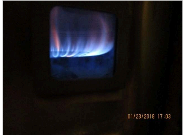
water heater burner viewed
