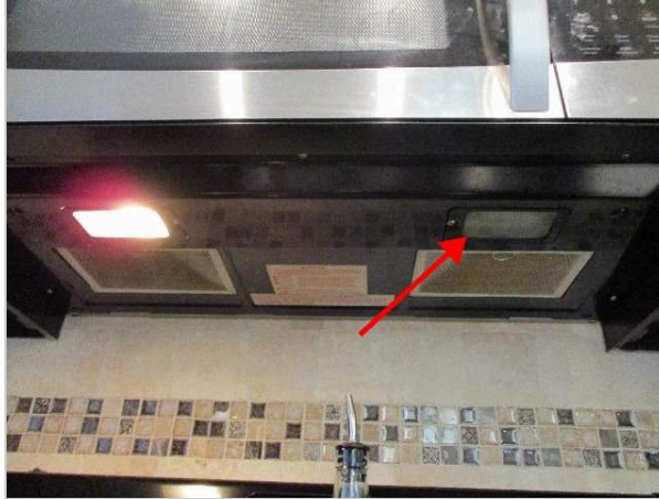
Light not functioning
