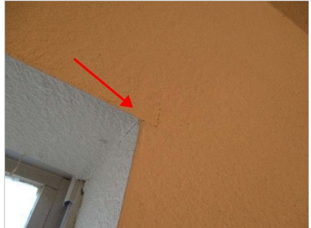
Sheetrock crack in master bathroom window
