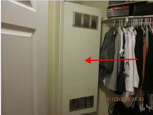
Water heater closet
