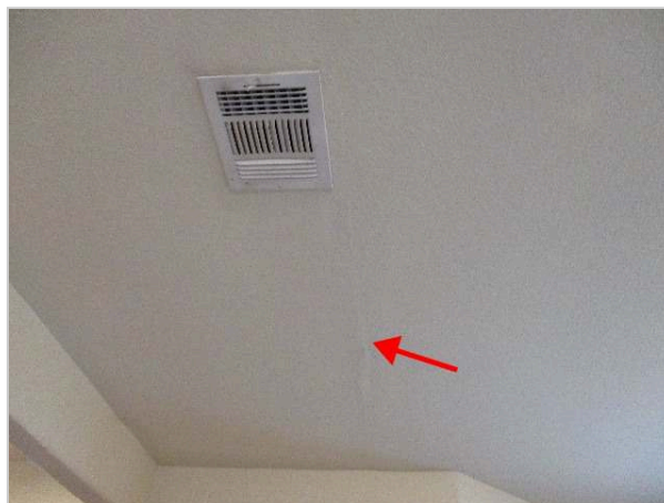
Stain / crack in dining area Page 9 of 17
