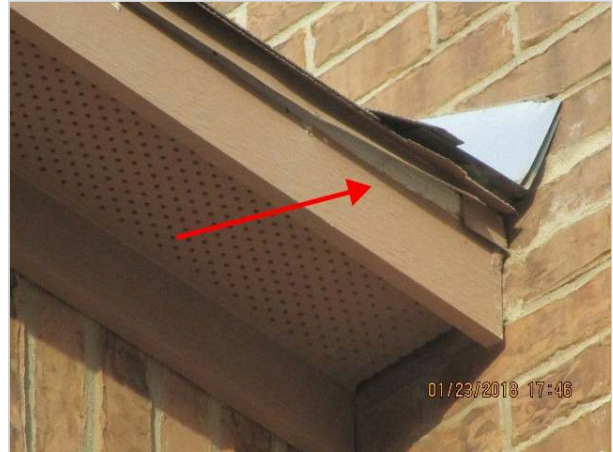
Damaged drip edge flashing
