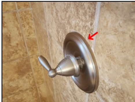
Fixture base not sealed
