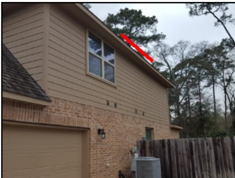
Recommend splash guard over condensing unit
