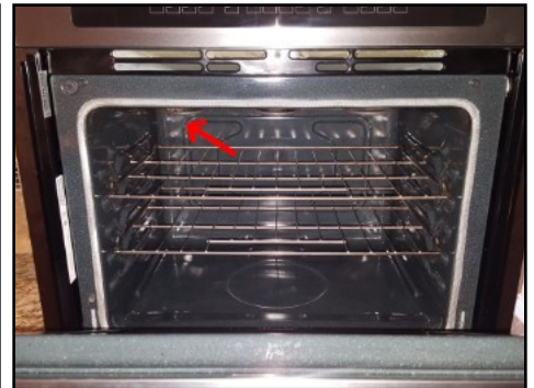
Oven light inoperable
