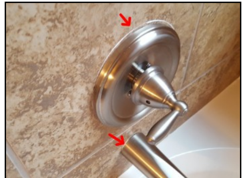
Fixture base not sealed
