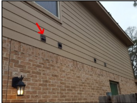
Dryer vent termination
