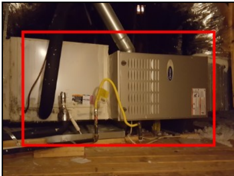
Furnace/Air handler located in attic space
