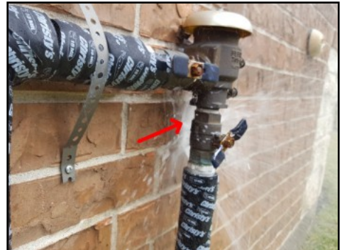
Anti-siphon device cracked/leaking
