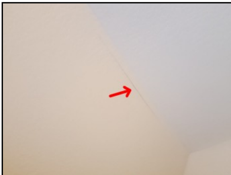
Settling crack at bedroom ceiling
