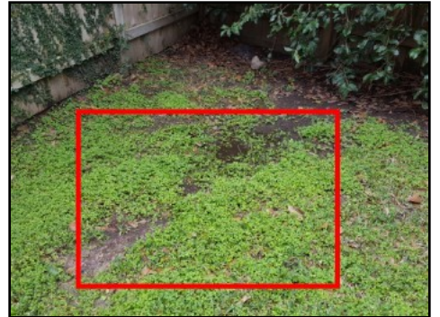
Excessive moisture at rear left elevation
