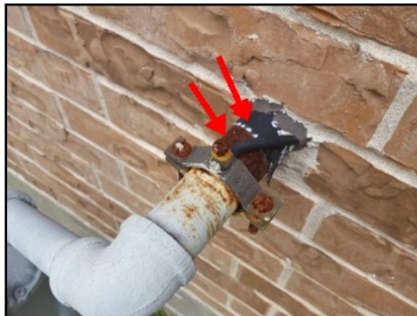
Gas line not protected/wrapped
