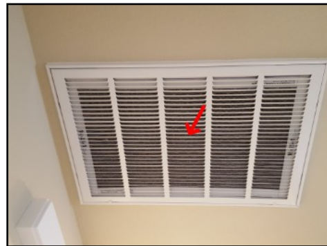
HVAC filter dirty
