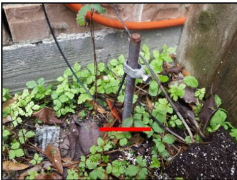
Ground rod not flush with grade
