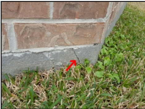
Wedge crack at rear right corner
