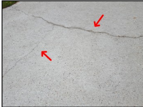
Cracks in driveway flatwork
