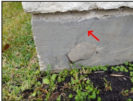
Wedge crack at front left corner
