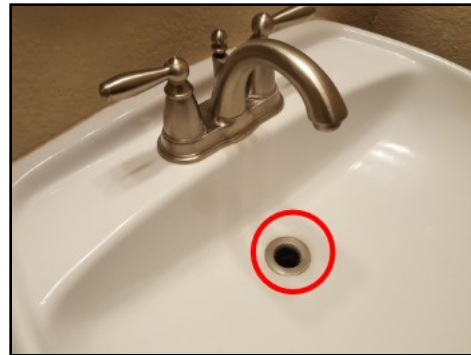
Drain-stop not present
