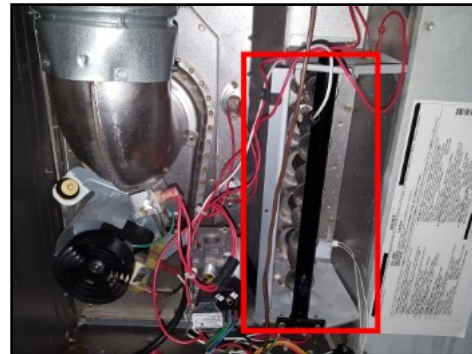
Furnace burner ports
