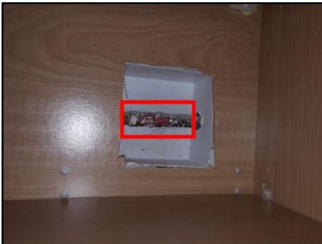
Gas line service valve within cabinet
