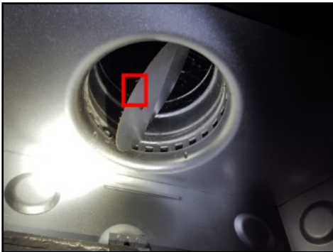
Recommend installing damper blocking clamp
