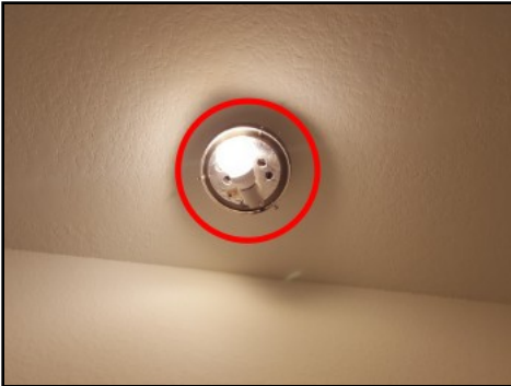
Missing light fixture protective globe
