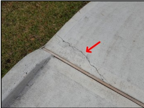
Crack in driveway flatwork
