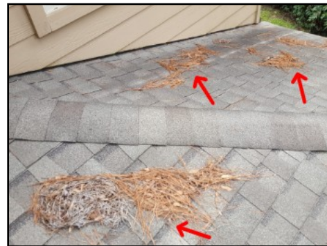
Debris on roof covering
