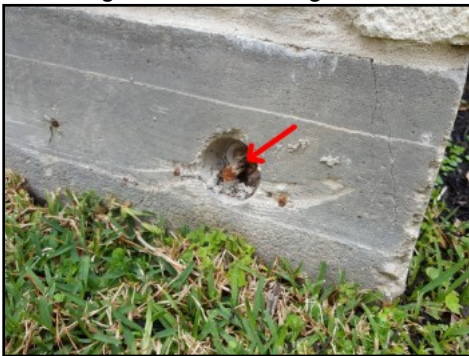
Exposed tension cable
