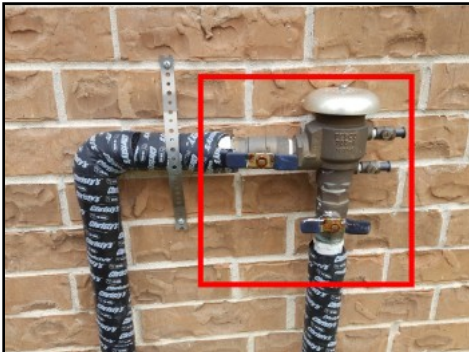
Main irrigation valves/anti-siphon device
