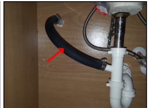
Primary A/C drain line
