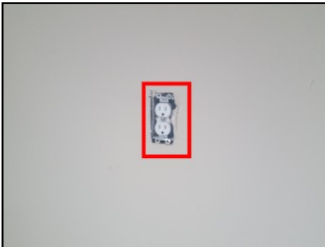
Missing receptacle cover plate
