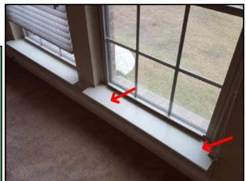
Window sill not secure in place
