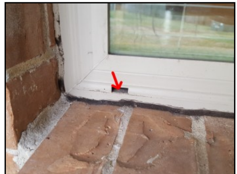
Weep hole cover missing at rear elevation
