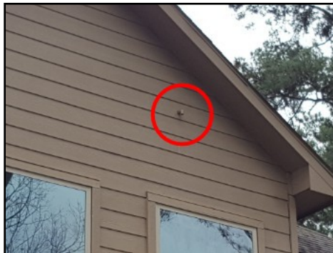
Secondary A/C drain line at rear elevation
