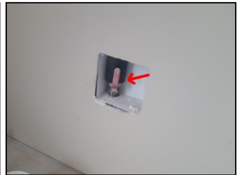
Main water shut off valve
