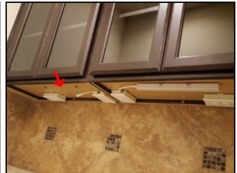
Light fixture not present
