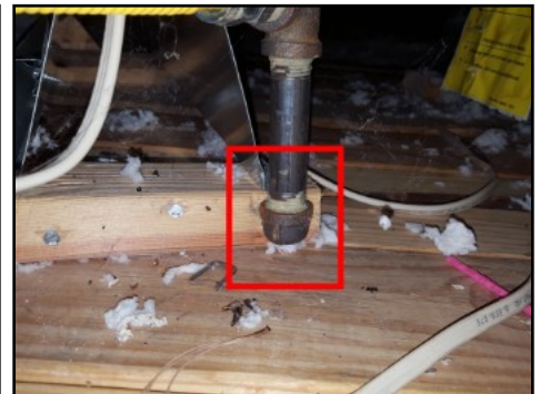
Sediment trap cap blocked
