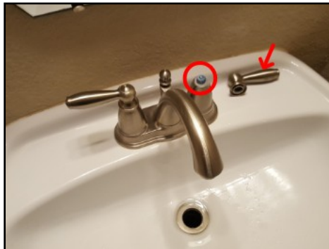
Fixture handle not secure in place
