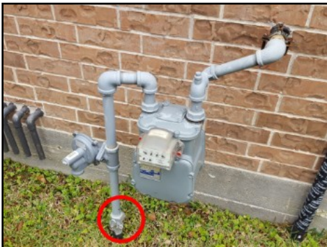
Gas meter and main shut off valve
