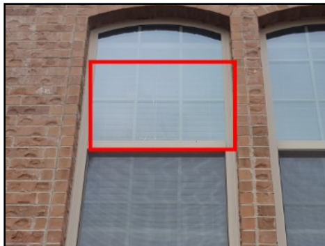
Seal failure at upper front left elevation
