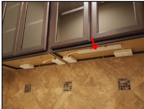
Light fixture inoperable
