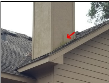
Mildew growth at chimney siding
