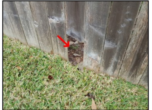
Fence picket damaged at rear elevation
