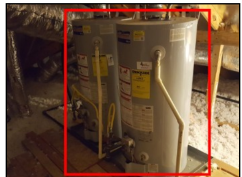
Water heaters located in attic space
