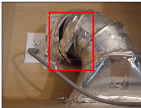
Vent duct not connected/sealed
