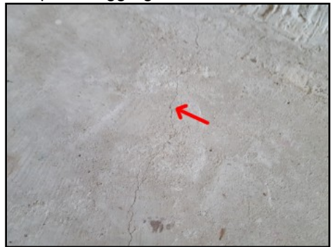
Hairline cracks in garage
