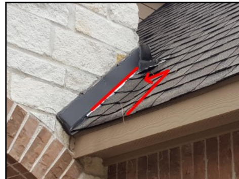
Roof deflection at front elevation
