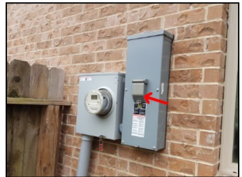
Homeowner main breaker location
