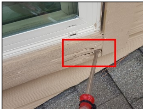
Deteriorated siding material at upper rear elevation
