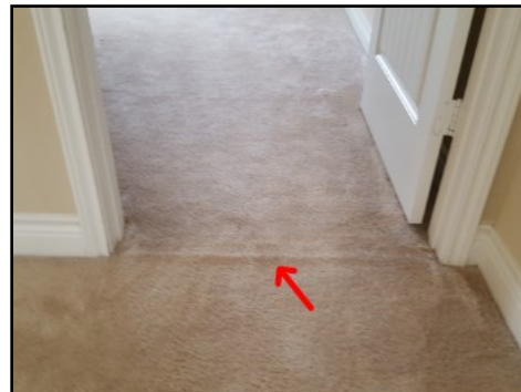
Carpet flooring loose
