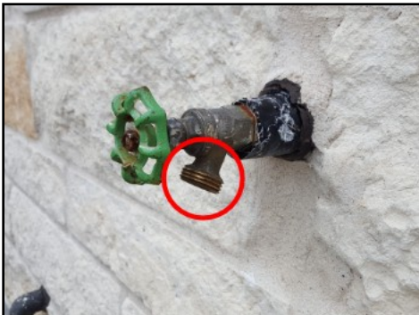
Missing back flow preventer at hose bibs
