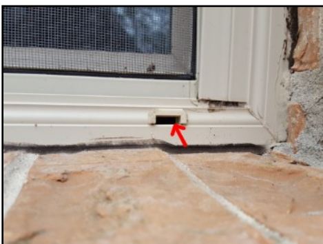
Damaged weep hole cover at rear elevation
