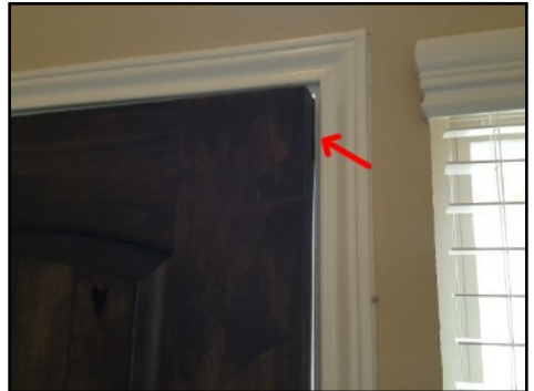
Door rubs on frame/jamb
