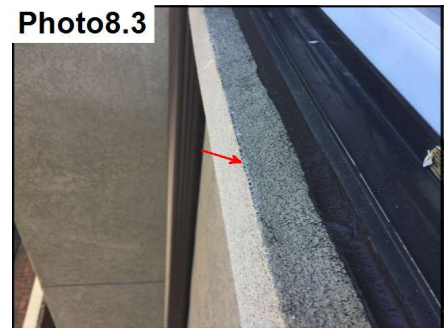
Impact damage noted at foam accent.
