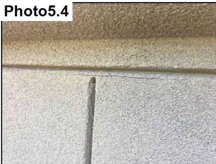
Cracked control joints noted. Seal / Repair as needed.
