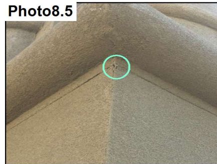
Cracked corner noted.
