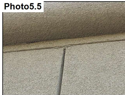
Cracked control joints noted. Seal / Repair as needed.
