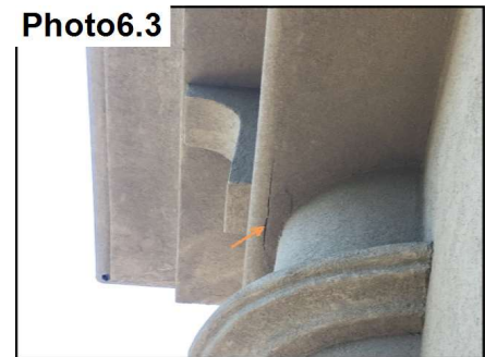
Seal / Repair crack as needed.
