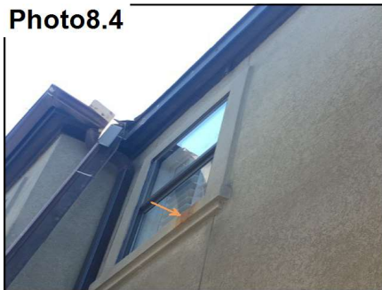
Rust staining from HVAC overflow noted.
