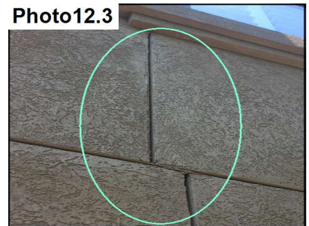
Cracked control joints noted.
