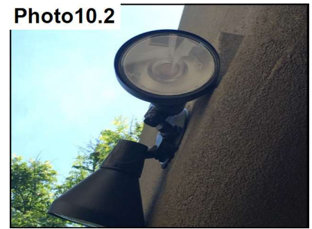
Light fixture lacks sealants.
