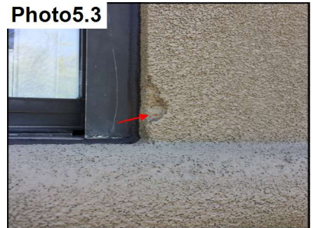
Impact damage is present. Seal / Repair as needed.
