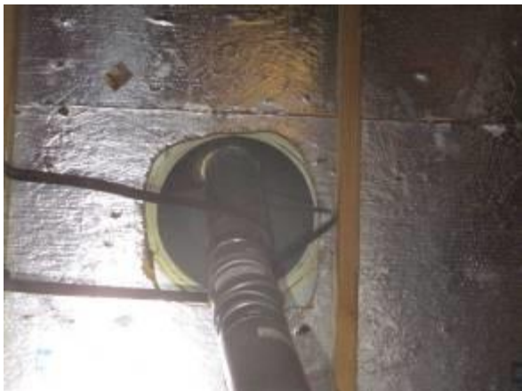
Visible daylight/Stained service decking
