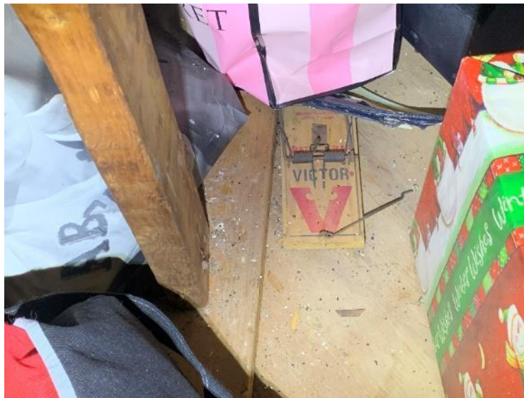
Rodent traps and droppings observed in the attic
