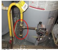
HEI file photo showing sediment trap
