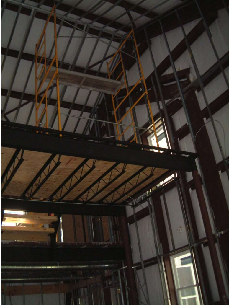
Exterior Wall and Ceiling ready to install batt insulation before sheetrock attachment to hat channels
