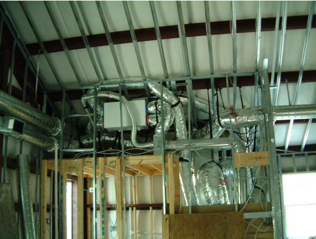
3 zone HVAC and bathroom(s) vent system.
