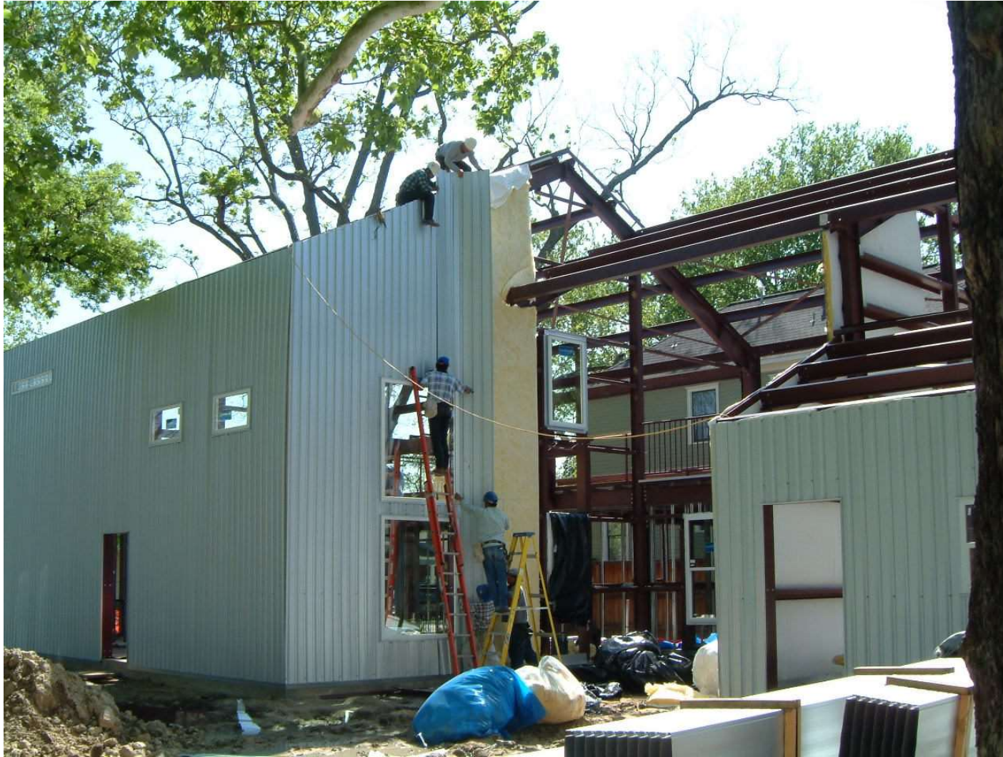
Exterior Sheathing Installed with Thin Layer of Insulation. Thicker Batt Insulation Installed Inside Prior to Sheetrock Installation.
