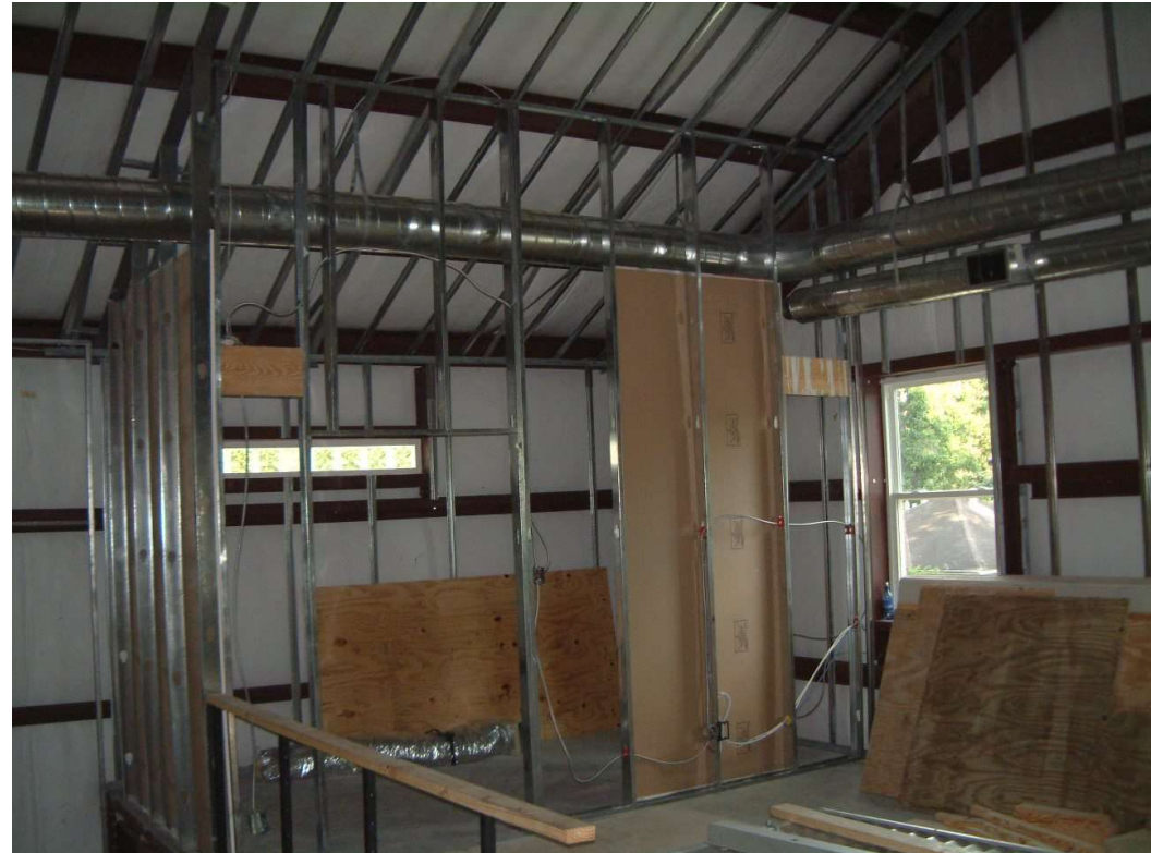
Typical interior room framing and exterior wall hat channels for sheetrock installation (batt insulation filled in behind hat channels that are attached to building girths and purlings).
