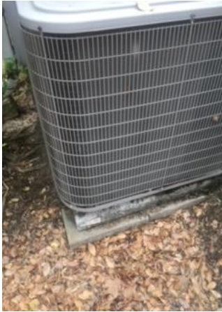
Clean condenser coil of dirt and debris.
