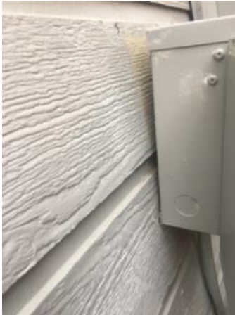
Secure disconnect box.
