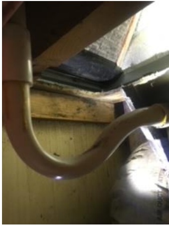
Insulate primary drain line per code and clear AC drain line.
