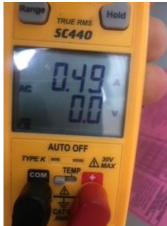
Condenser fan motor rated load amp.
