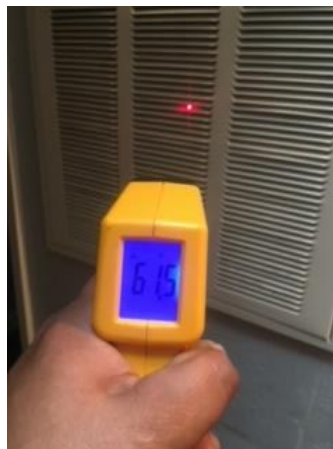
61° return air Evaporator coil split: 19° Normal split: 15 degrees and over
