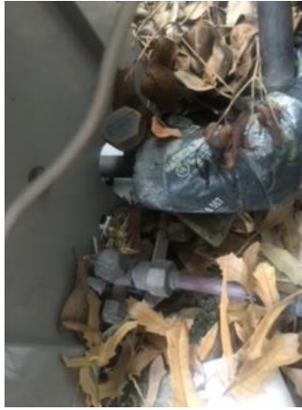
Install freon locking caps per code.
