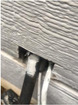
Seal gaps around copper line.
