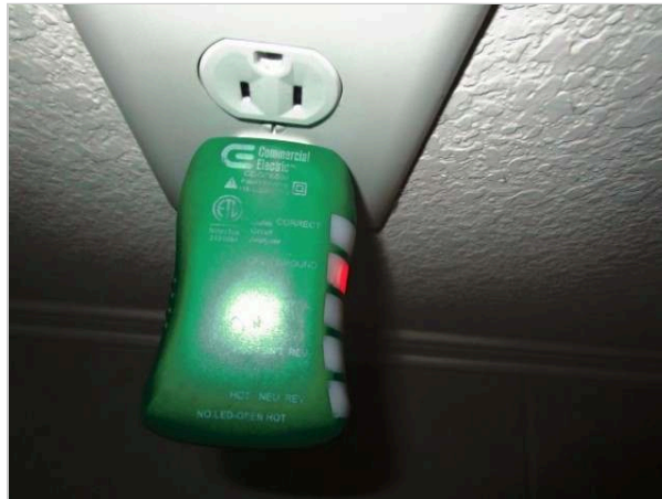
Open ground indication - rear receptacle, right wall
