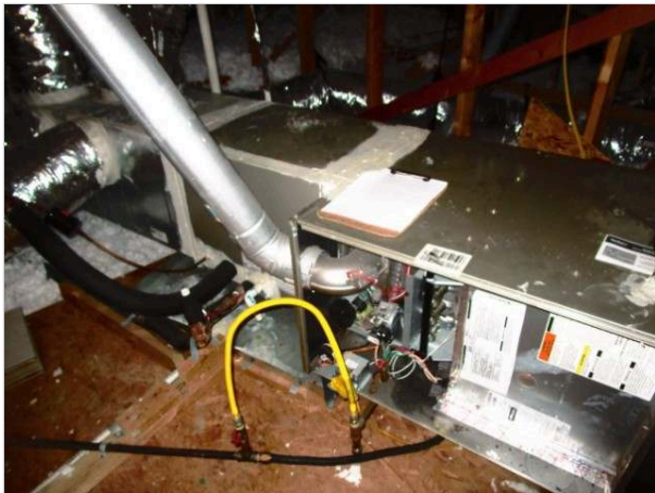
Furnace in attic
