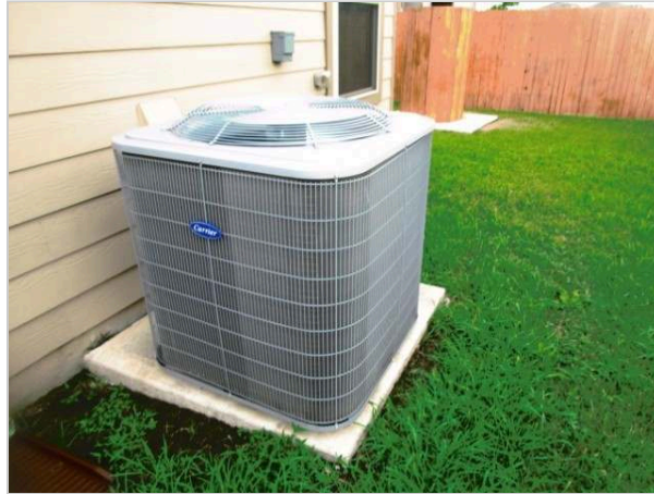
Outside condensing unit
