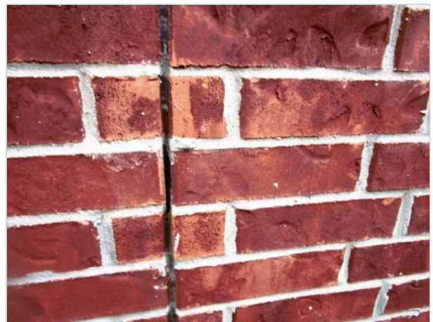
Expansion Joint needed sealant
