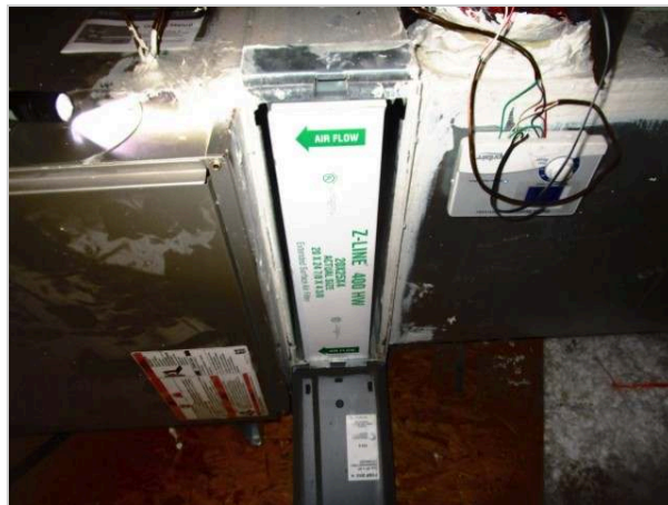
Filter in attic
