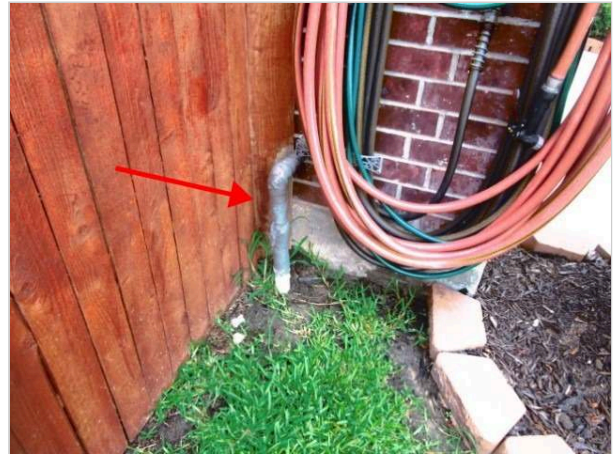
Main water valve
