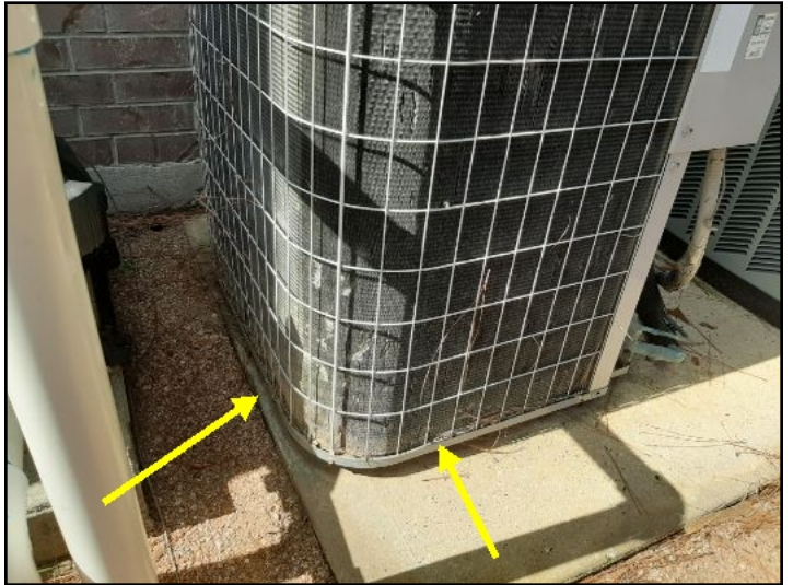
DIRTY / DAMAGED COILS
