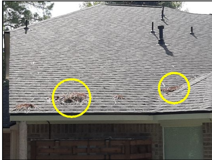
DEBRIS AT ROOFTOP
