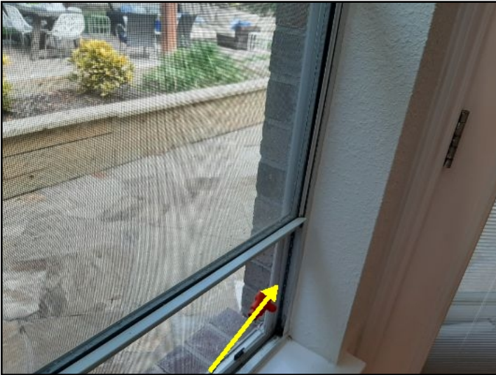
DAMAGED WINDOW HARDWARE
