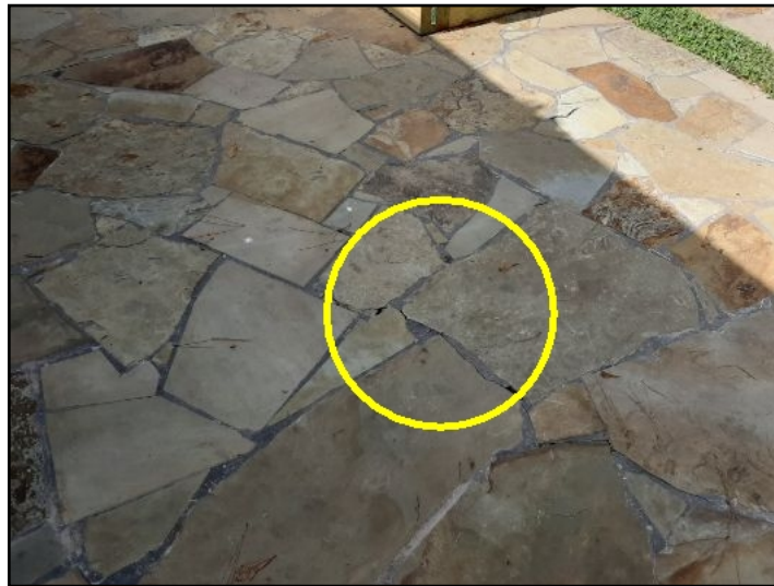
DAMAGE / VOIDS AT PATIO MORTAR
