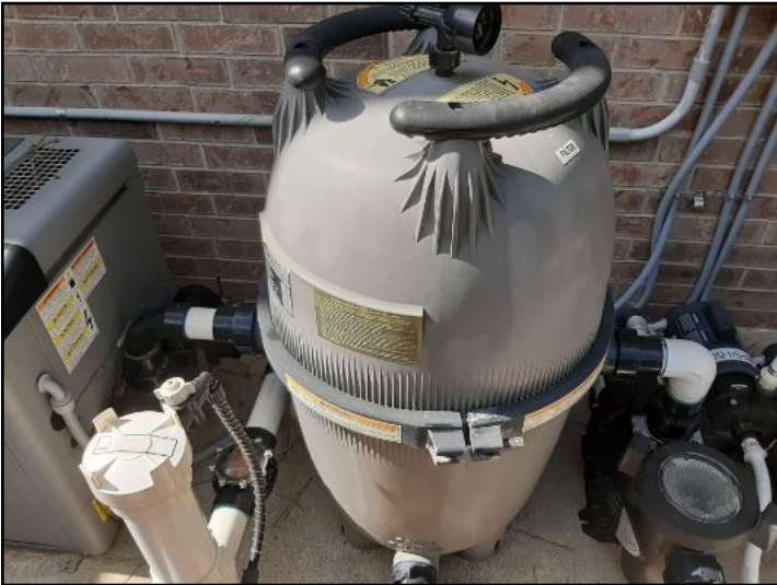
FILTER IN GOOD CONDITION
