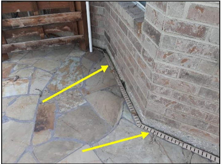
EVIDENCE OF CLOGGING AT DRAIN CHANNEL
