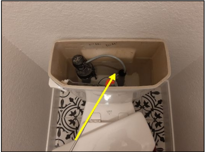
WATER LEVEL TOO HIGH; CONTINUES TO RUN
