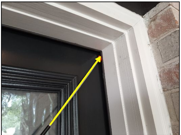
GAP AT DOOR AND WEATHERSTRIPPING
