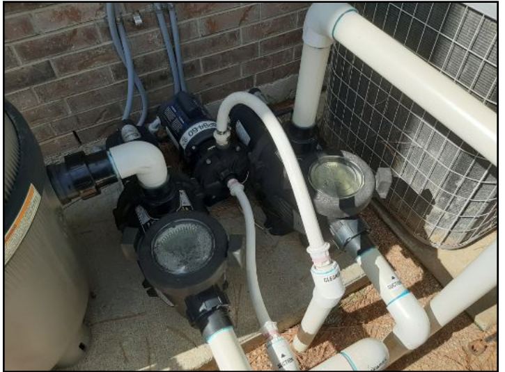
POOL PUMP OK
