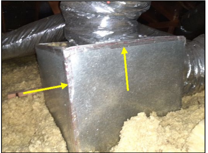
MISSING / NO FIBER PAINT
