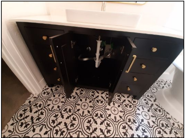
EVAPORATOR DRAINS INTO THIS SINK
