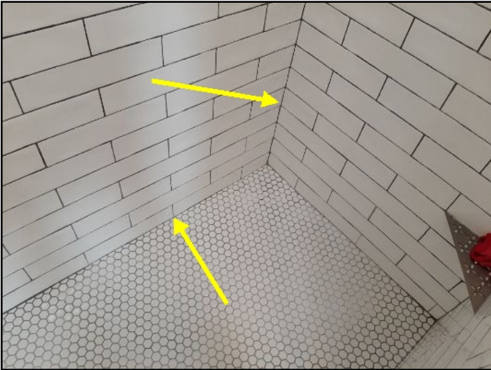
SEAL DETERIORATION / UNSEALED AREAS
