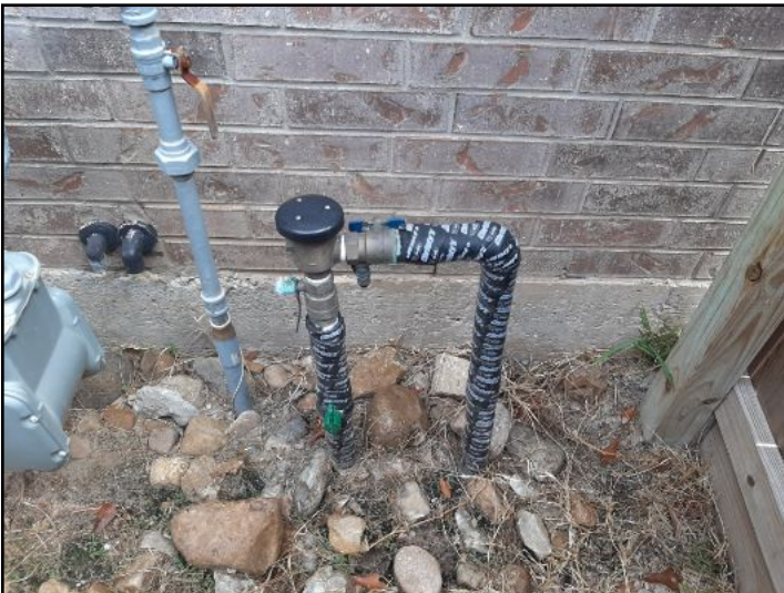
SPRINKLER BACKFLOW OK
