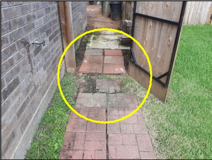
LOW AREAS; PRONE TO WATER PONDING
