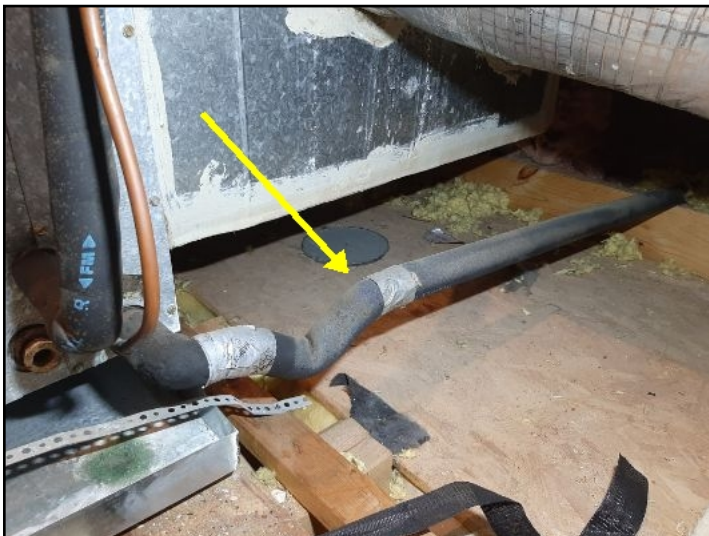
MISSING / NO ACCESS TO PIPE FOR CLEANING AND MAINTENANCE
