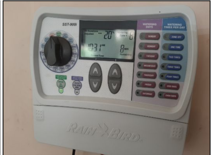
SPRINKLER CONTROL OPERATIONAL; 8 ZONES PRESENT
