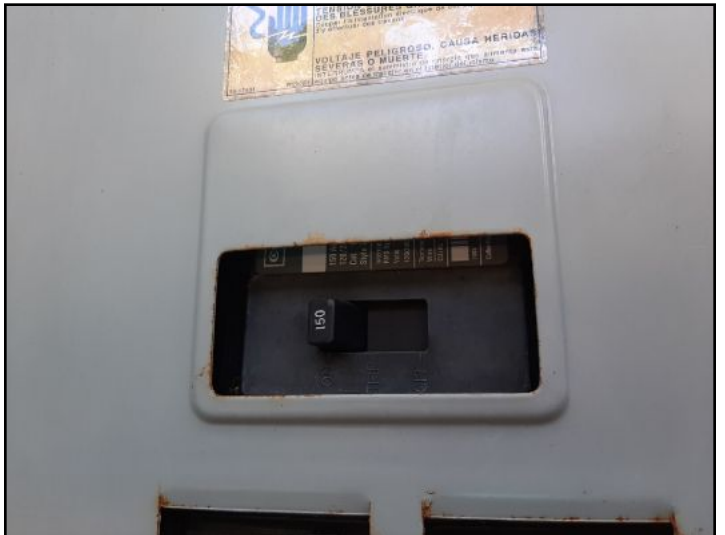
MAIN BREAKER OK
