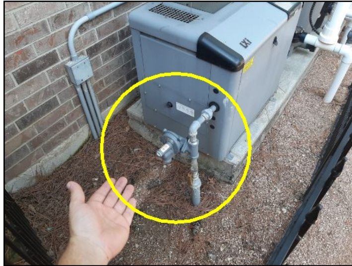
EVIDENCE OF GAS SMELL / LEAK
