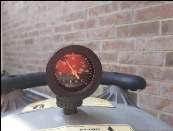
POOL WATER PRESSURE OK
