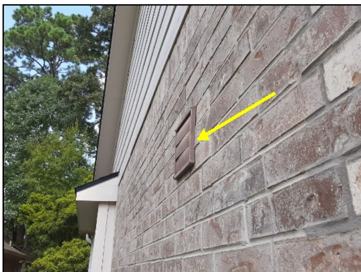
SEAL DETERIORATION AT EXTERIOR VENT
