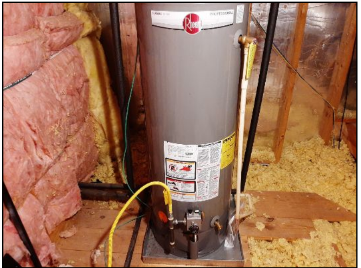
WATER HEATER OK
