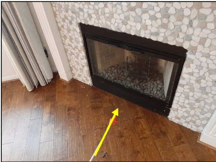
INSUFFICIENT CLEARANCE AT FRONT OF FIREPLACE
