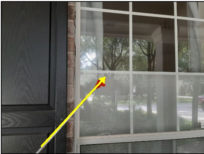
DAMAGED WINDOW PANE
