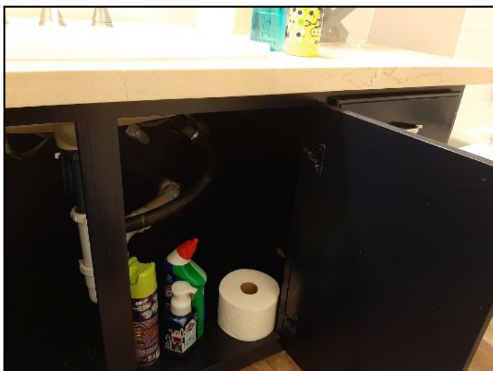
EVAPORATOR DRAINS INTO THIS SINK
