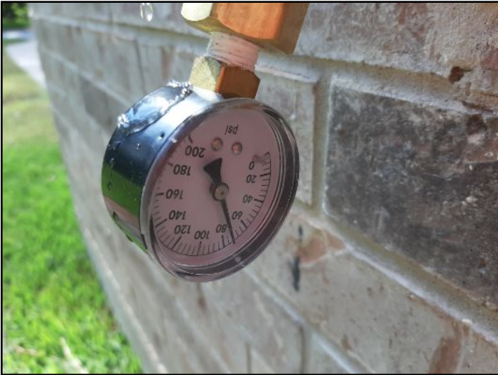
WATER PRESSURE OK; 75 PSI
