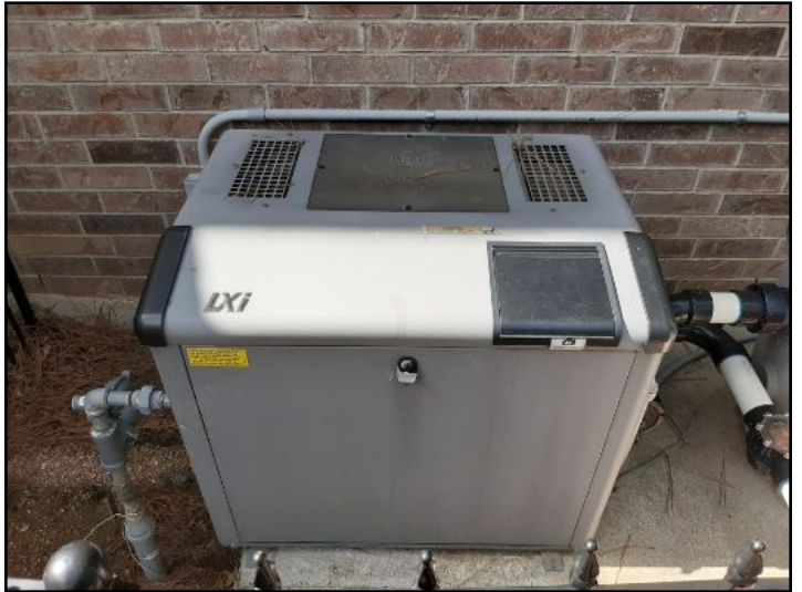
POOL HEATER OPERATIONAL
