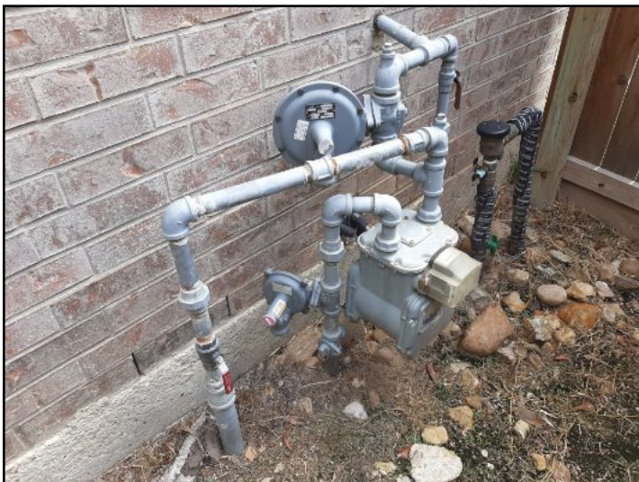
GAS METER OK
