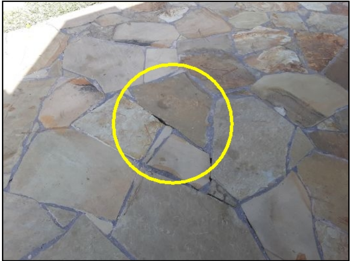
DAMAGE / VOIDS AT PATIO MORTAR
