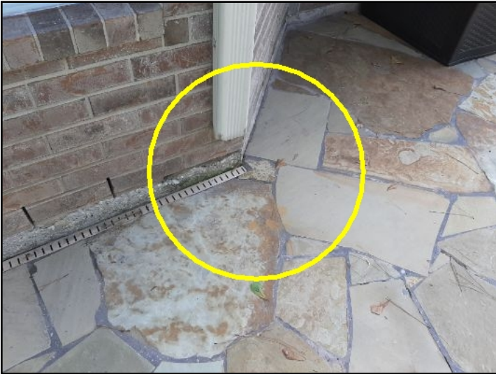
MISSING SPLASHBLOCK / EXTENSION
