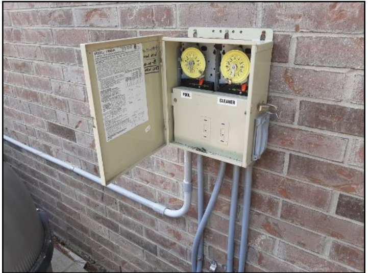
POOL CONTROL OPERATIONAL
