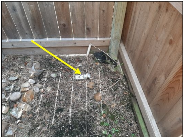
DAMAGED / UNSECURED SPRINKLER RAIN SENSOR
