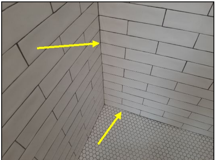
SEAL DETERIORATION / UNSEALED AREAS
