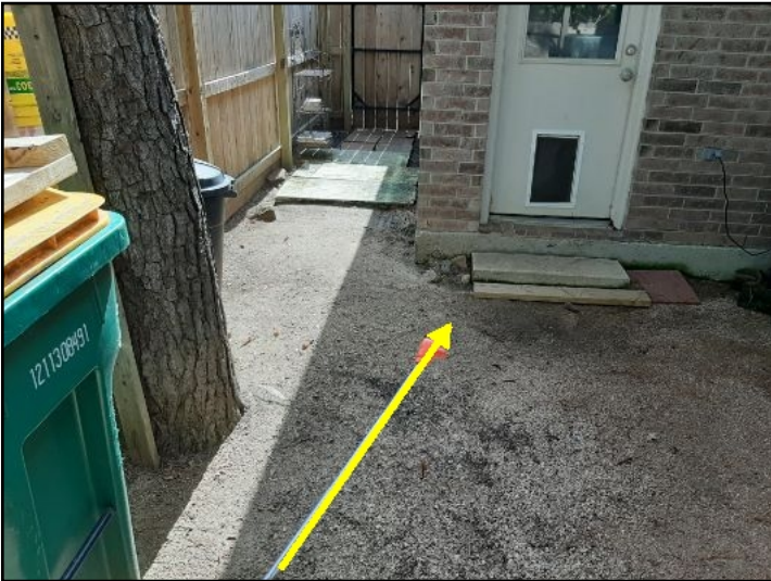
EVIDENCE OF STANDING WATER / PONDING
