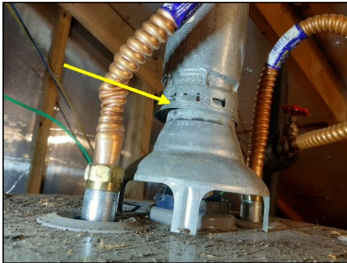
UNSECURED EXHAUST VENT
