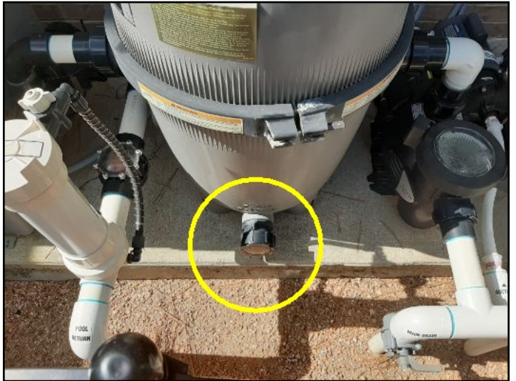
MISSING / NO BACKWASH SYSTEM PRESENT
