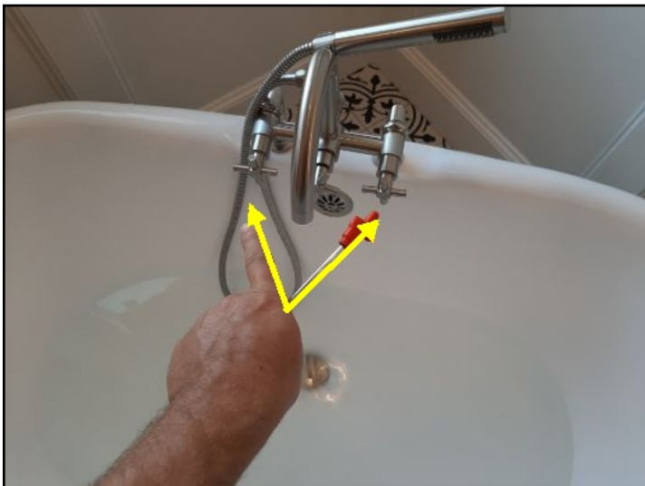
HOT AND COLD SUPPLY REVERSED
