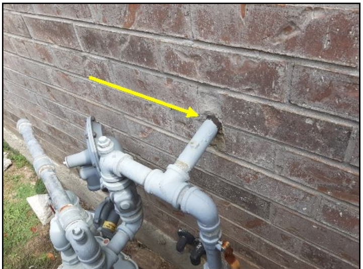
MISSING BONDING AND PROPER WALL TRANSITION
