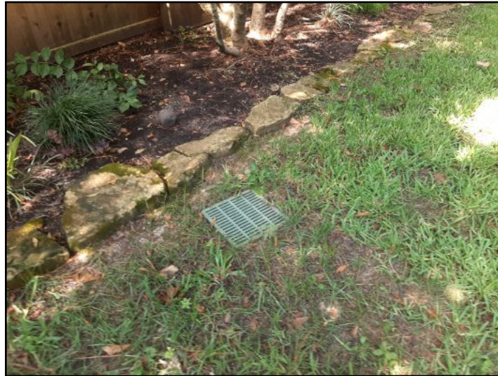
FRENCH DRAINS PRESENT OK
