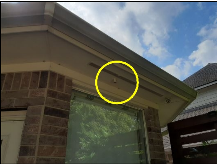
EVAPORATOR SECONDARY DRAIN PIPE ROUTED HERE
