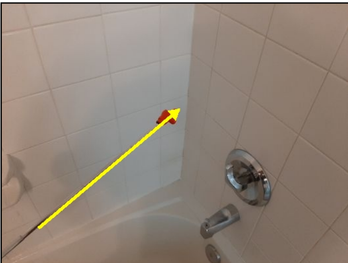
SEAL DETERIORATION / UNSEALED AREAS
