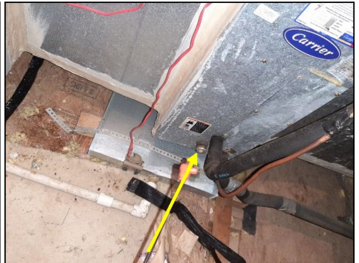
MISSING OVERFLOW DRAIN PIPE
