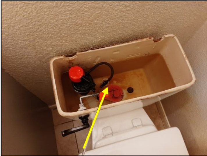
WATER LEVEL TOO HIGH; CONTINUES TO RUN
