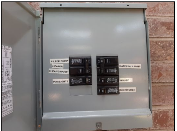
SUB PANEL OK
