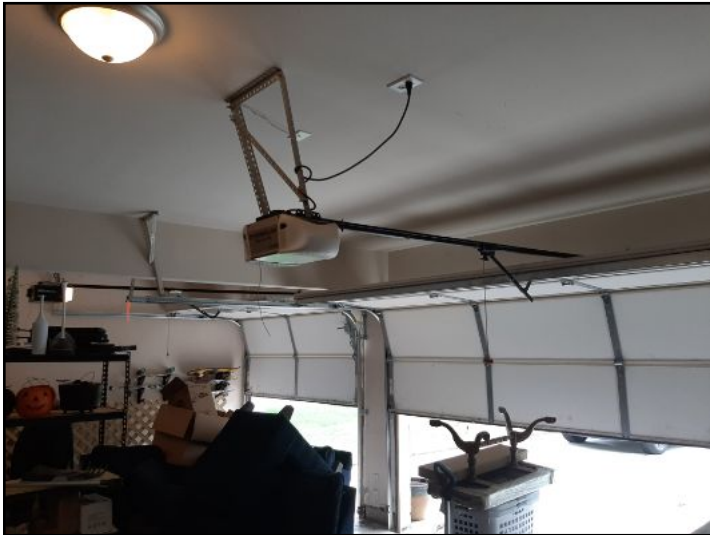
GARAGE DOOR OPENER OK
