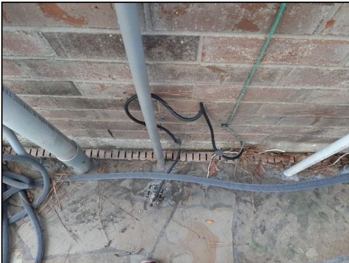
MAIN GROUNDING OK
