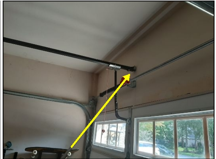
LOOSE / UNSECURED GARAGE DOOR RAIL
