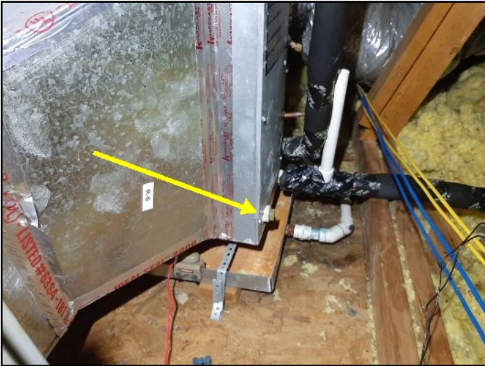
MISSING OVERFLOW DRAIN
