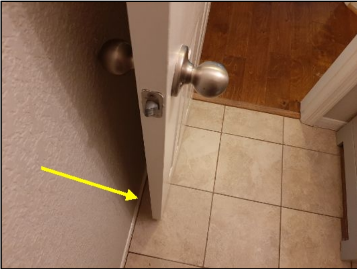
MISSING DOOR STOPPER
