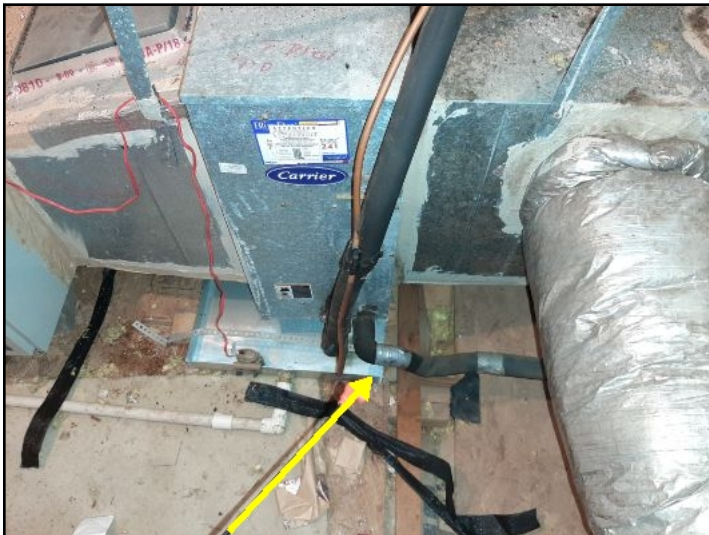
DRAIN PAN DOES NOT FULLY COVER EVAPORATOR
