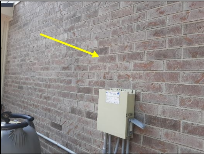
MISSING LIGHT FIXTURE AT POOL EQUIPMENT AREA
