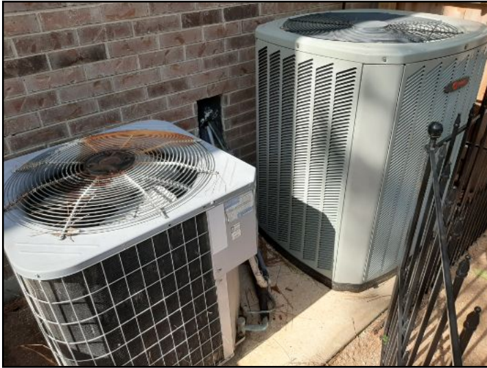
CONDENSING UNIT OK
