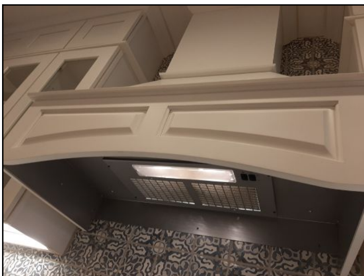
VENT HOOD OK
