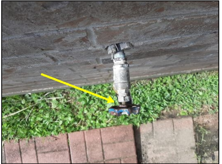
LEAKING VALVE WHEN IN THE OPEN POSITION
