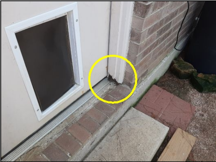
WOOD ROT AT FRAME
