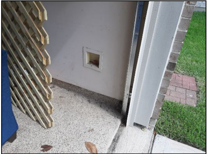
MAIN WATER VALVE OK
