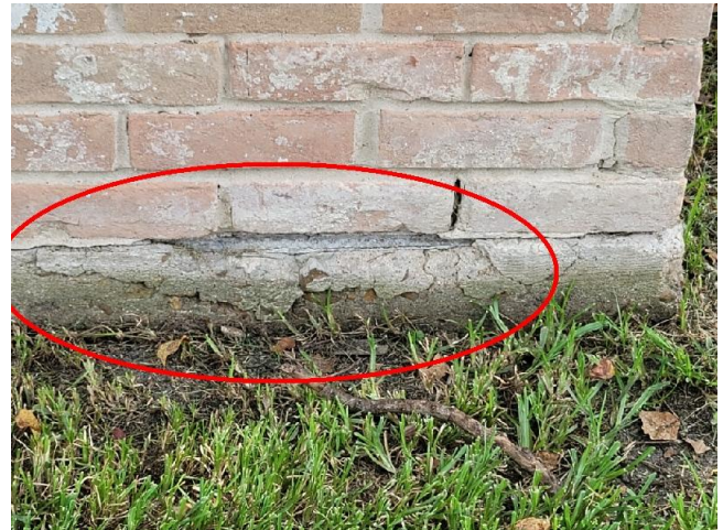
Another example of the multiple locations of spalling on the foundation.
