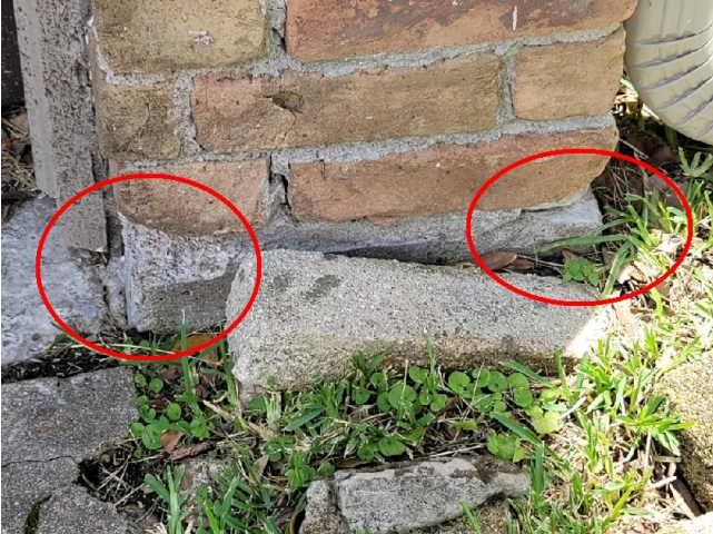
Corner pops/corner cracks were observed on the foundation.
