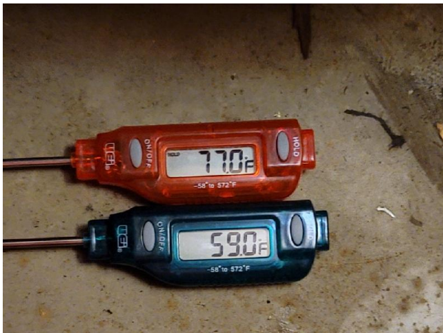
The temperature drop across the coil of the AC unit at the time of this inspection was 18 degrees. This is considered acceptable.
