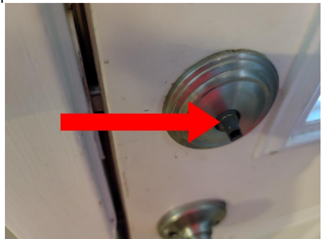
Damage or missing door hardware was observed and needs to be repaired.
