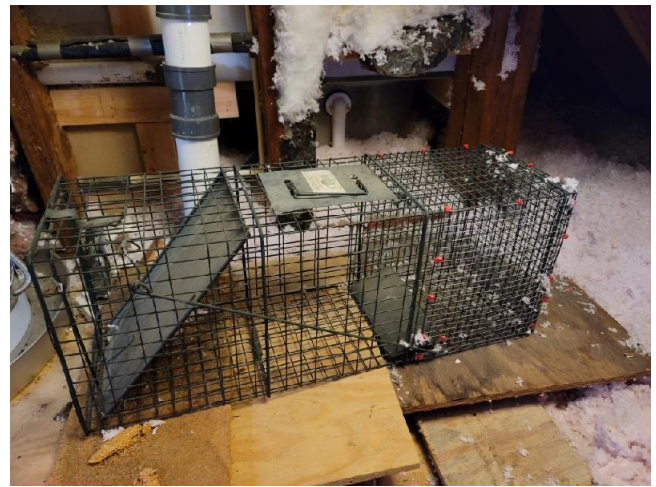
A live catch trap was observed in the attic and is an indication that rodents were or are present in the structure.
