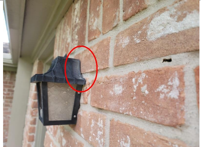
All exterior light fixtures need to be caulked at their base to prevent water penetration into the fixture or structure.
