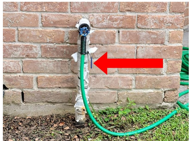
This Photograph shows the location of the main water supply shut off valve located on the exterior wall at the northeast corner of the home.
