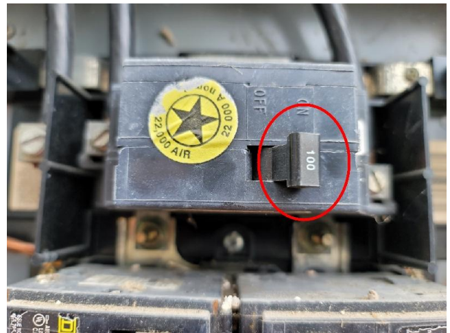
This Photograph confirms the statement above that this is a 100-amp service.
