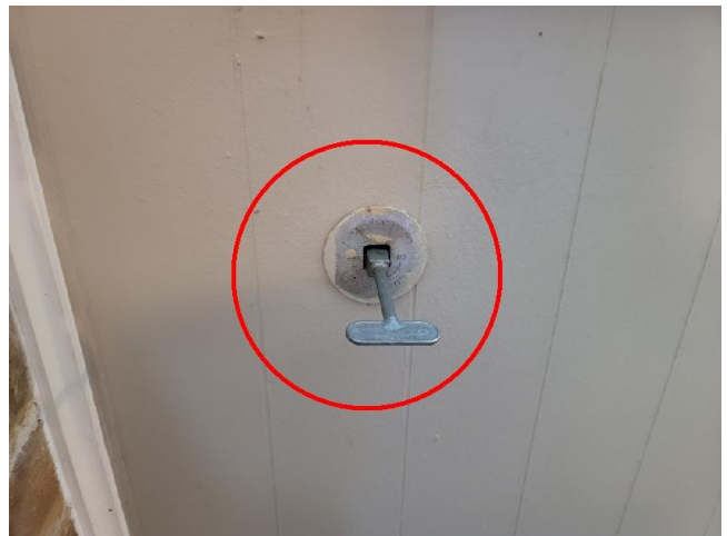
Inoperative gas valve. The gas control valve for the fireplace will not turn; therefore, it cannot be determined whether it is stuck in the on or off position.
