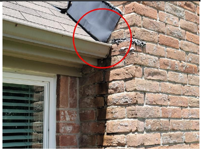
Missing kickout flashing around the chimney were observed. See the comments above and the following illustration.
