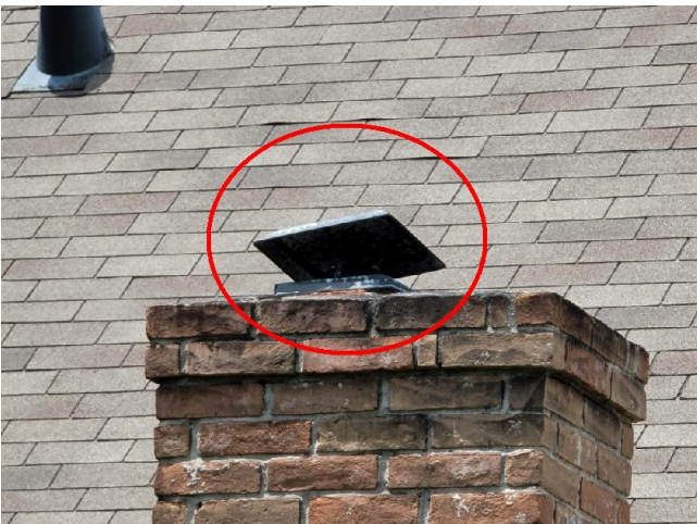
The chimney cap on top of the chimney was observed to be loose and there is no spark arrestor installed.
