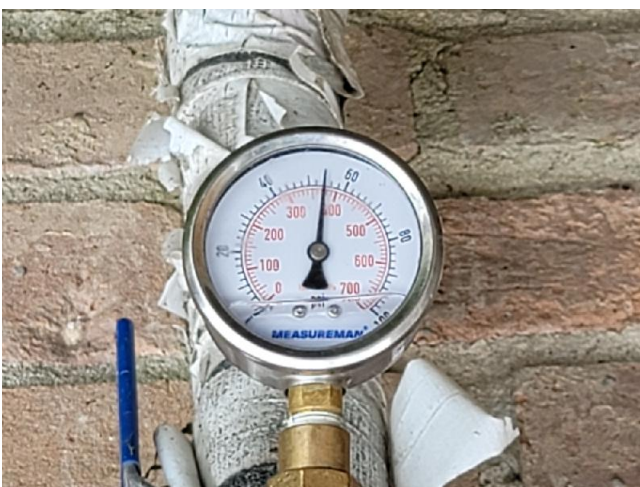
54 PSI main water supply pressure is considered acceptable.
