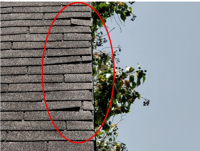
Another example of deficient shingles that were observed on the roof.
