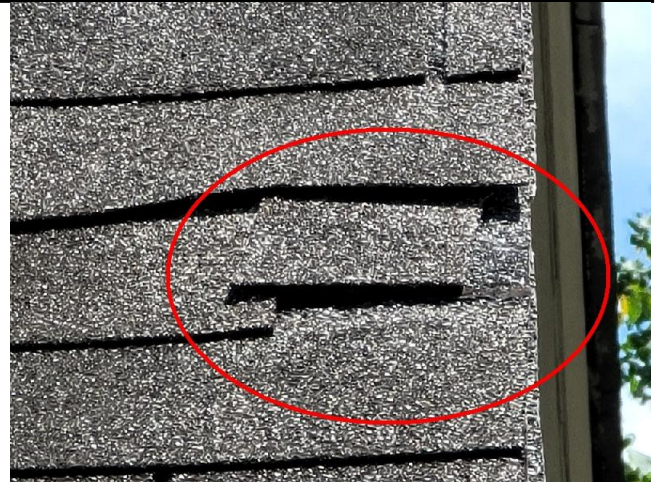
Torn shingles were observed.
