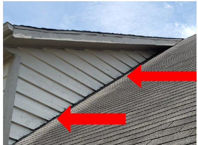
Multiple locations of siding were observed to be in contact with the shingles. See the comments above and the following illustration about the 2" rule.
