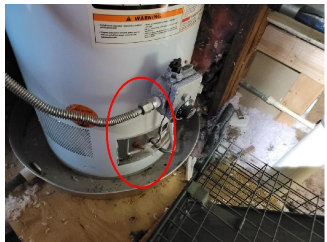
There is no sediment trap installed on a gas supply line to the water heater. See the comments above and the following illustration.
