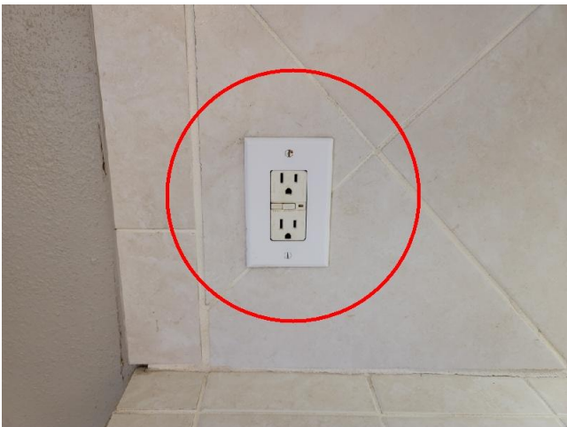
The GFCI outlet beside the kitchen sink is improperly wired. It will not trip when tested and even when manually tripped it still functions. This is a safety hazard. See the comments above.
