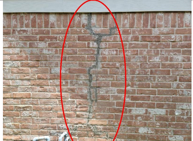
Multiple locations of various types, sizes and degrees of cracks that both have and have not been patched were observed on the exterior walls.
