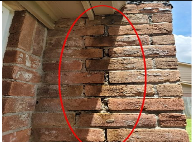
Deteriorated mortar was observed on the chimney below a missing kickout flashing on the roof. See the comments above.
