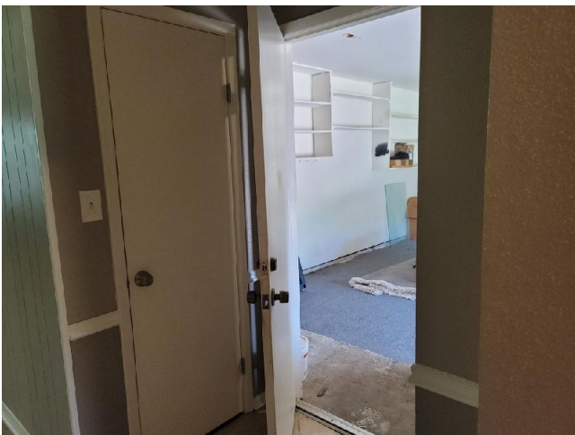
The garage door to the house is not self-closing. This is considered to be a safety hazard. See the comments above.
