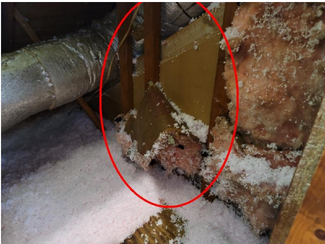
Insulation in the attic was observed to be falling off the sidewalls. See the comments above.
