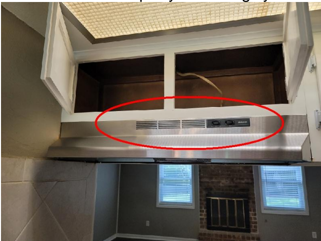
The range hood exhaust vent does not exhaust to the exterior as required by today's standards. See the comments above.
