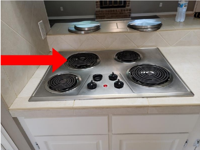
Using normal operating controls the right rear burner on the electrica cooktop would not operate.
