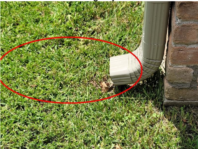
Multiple locations of missing splash blocks were observed. See the comments above.
