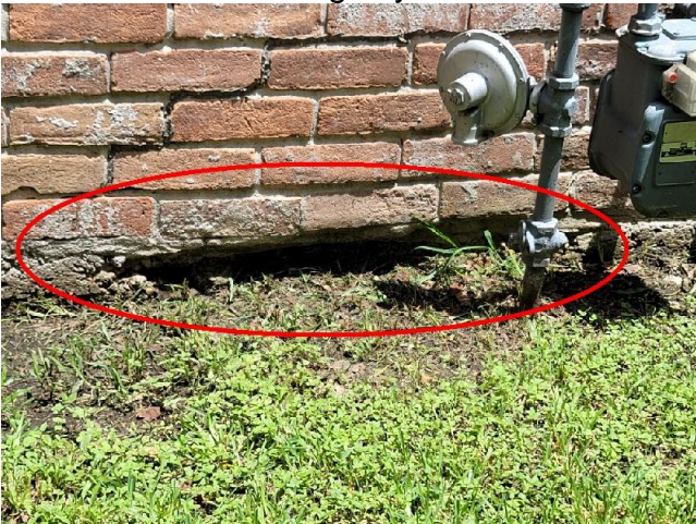
Exposed and corroding rebar on the foundation may be the cause of the spalling in the concrete at this location and other locations.
