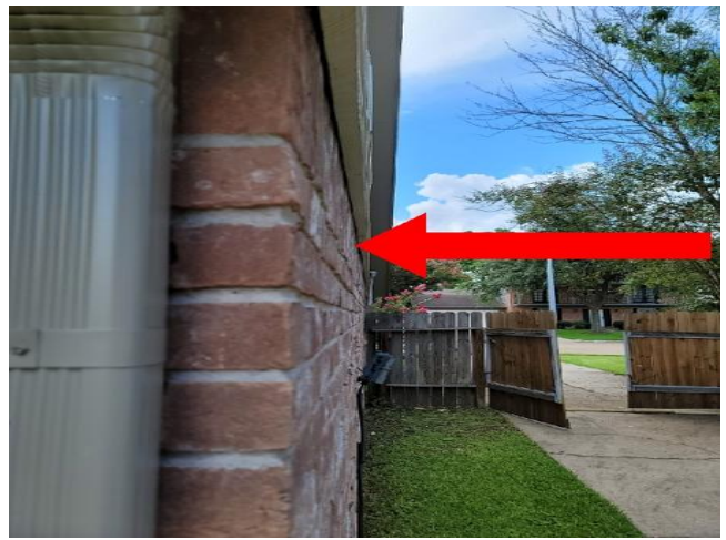
This east facing exterior wall was observed to be bowing.
