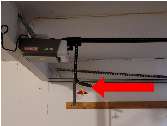
Both automatic garage door operators have been disconnected.
