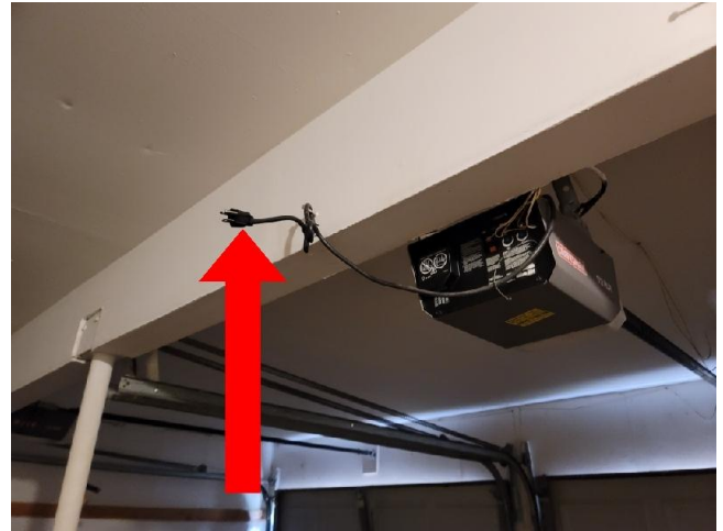
Both automatic garage door openers were unplugged at the time of this inspection.
