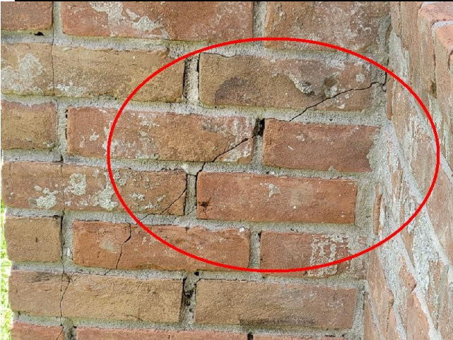
Cracks were observed on the exterior of the chimney. See the comments above.
