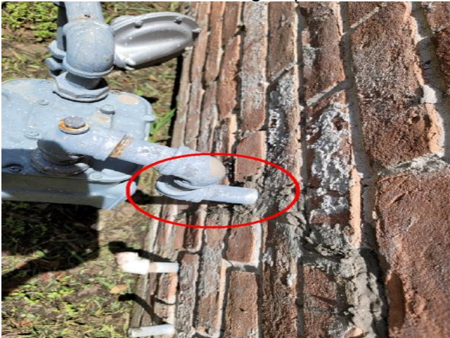
This photograph confirms the statement above that the gas meter was not bonded at the time of this inspection.
