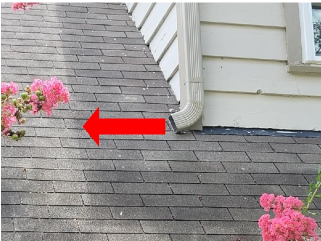
A downspout was observed to be discharging stormwater runoff at a 90-degree angle to the lay of the shingles. See the comments above.
