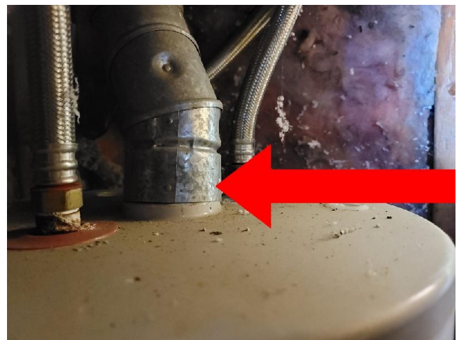
There is no draft hood installed on the exhaust vent on top of the water heater.
