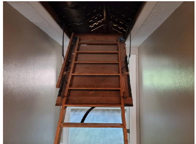
The attic access ladder should be insulated for increased energy efficiency.
