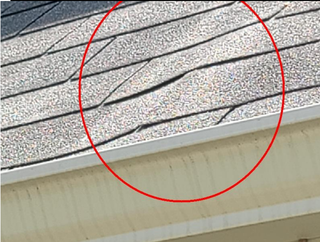
Buckled shingles were observed.
