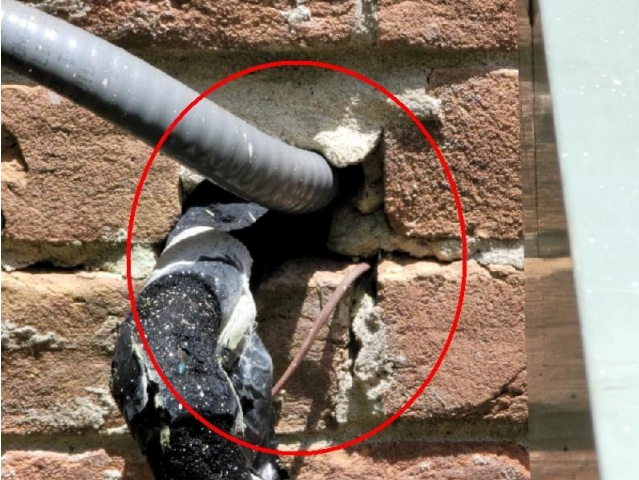
All holes and access points on the exterior walls need to be sealed/repared to reduce the risk of rodent and water penetration into the structure.
