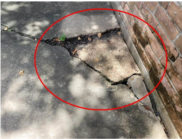
Multiple locations of trip hazards were observed on the back patio.
