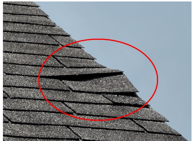
Multiple locations of buckled, uplifted or deficient shingles were observed.
