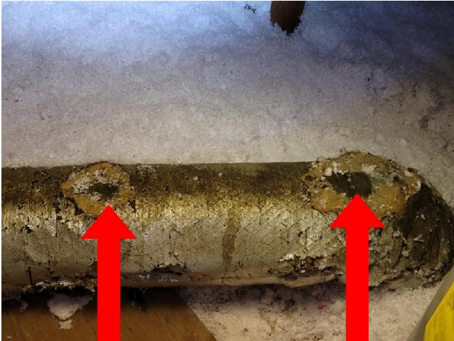
The insulation on the HVAC ducts in the Attic appears to have been chewed away by rodents to access moisture / condensation to drink.
