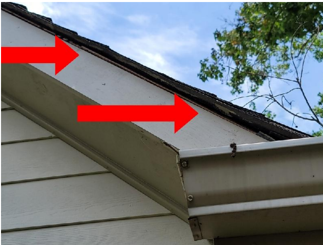
There is no drip / rake edge flashing installed around the west side of the roofs edge. See the comments above and the following illustration.
