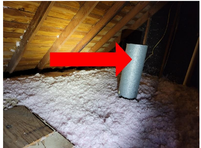
The exhaust fan in the ceiling of the kitchen was observed to be discharging directly into the attic. See the comments above.
