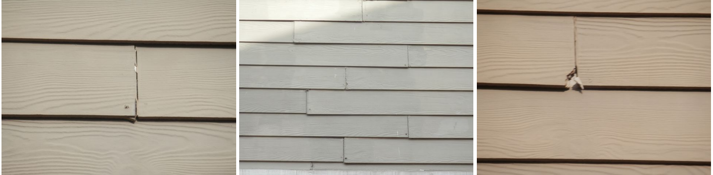
sample of siding end joints that are recommended to be caulked or sealed
