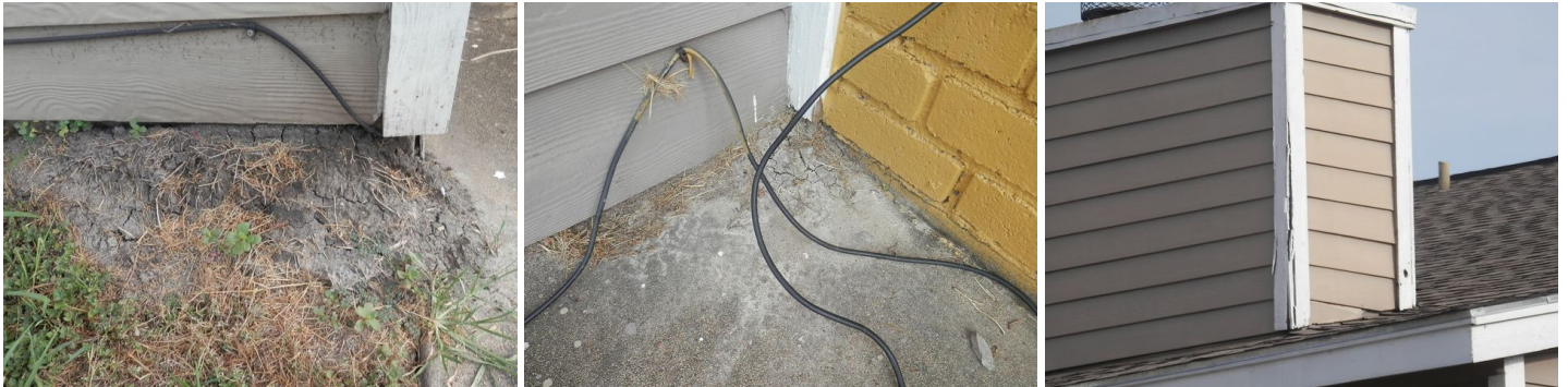
sample of ant beds at the back of unit C - void in trim at fireplace chimney housing
