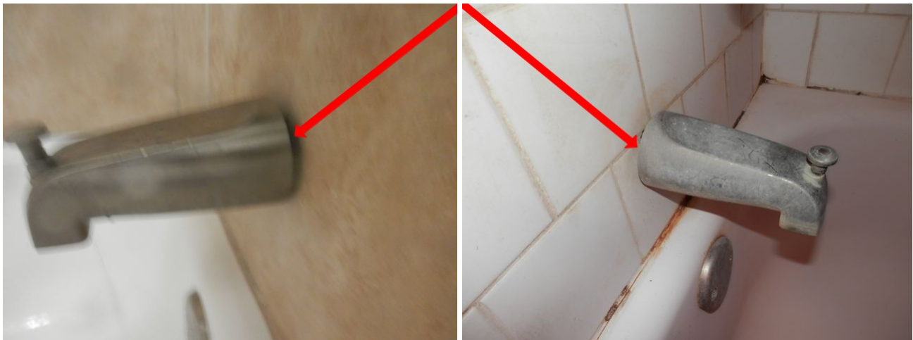
sample of faucet not sealed at the wall in unit A and C
