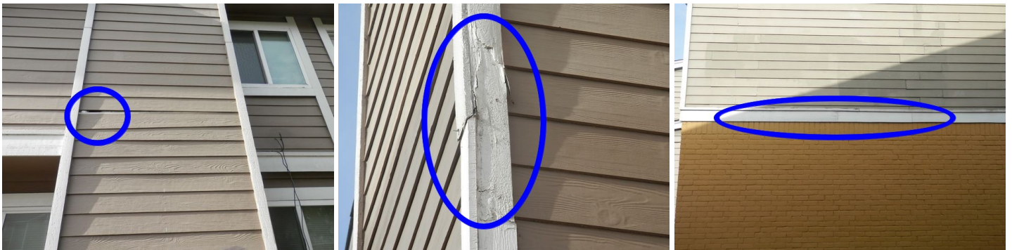
loose siding - deteriorated / soft wood
