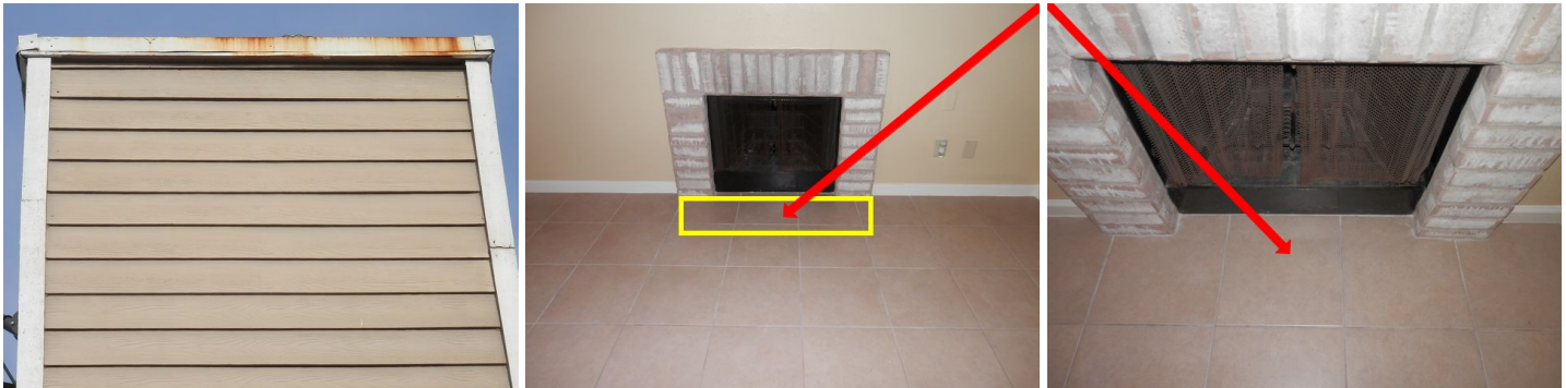
chimney cap appeared to be rusted - no discernable hearth at front of the fireplace firebox at unit A
