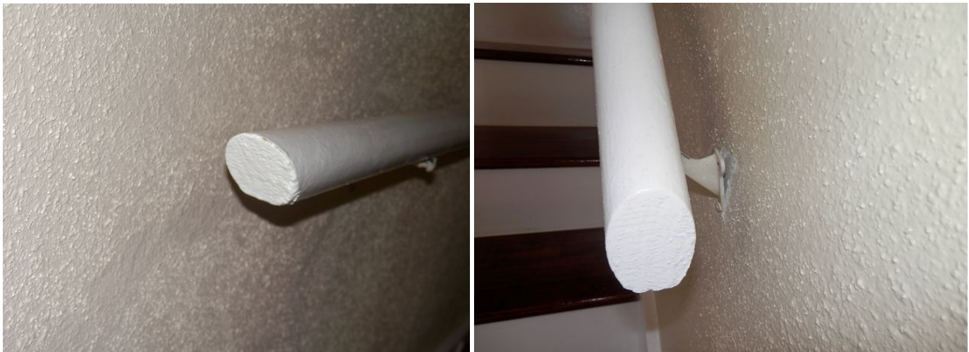
sample of hand rail not terminated to the wall (safety note) - hand rail was loose at wall in unit A
