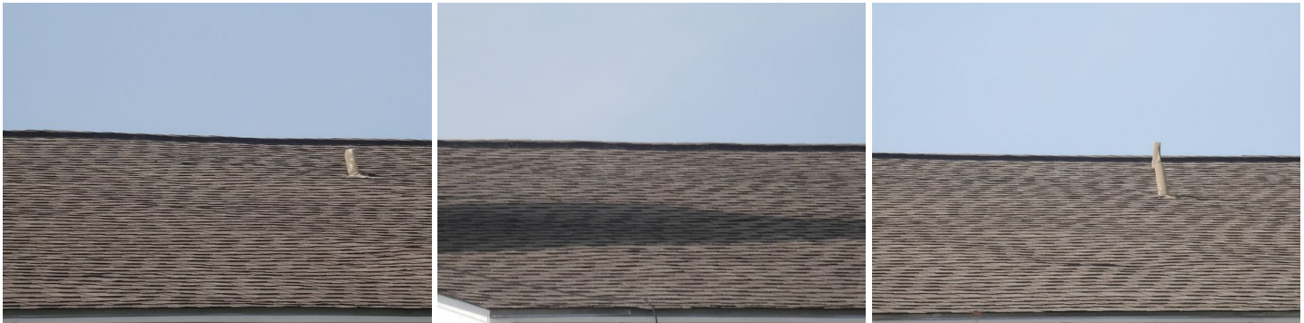
general view of the roof covering as seen from the ground at the front of the property
