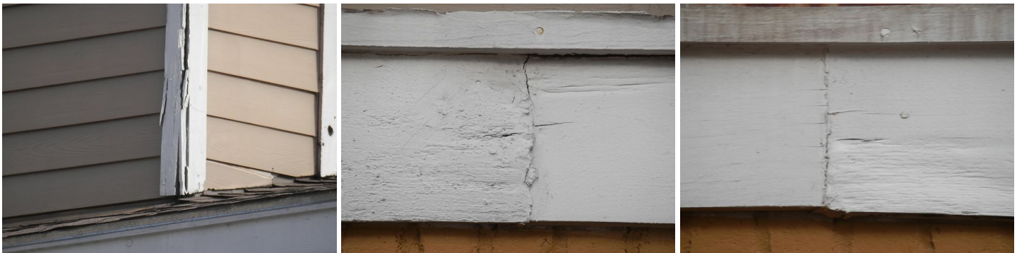
sample of loose trim and/or soft, deteriorated wood
