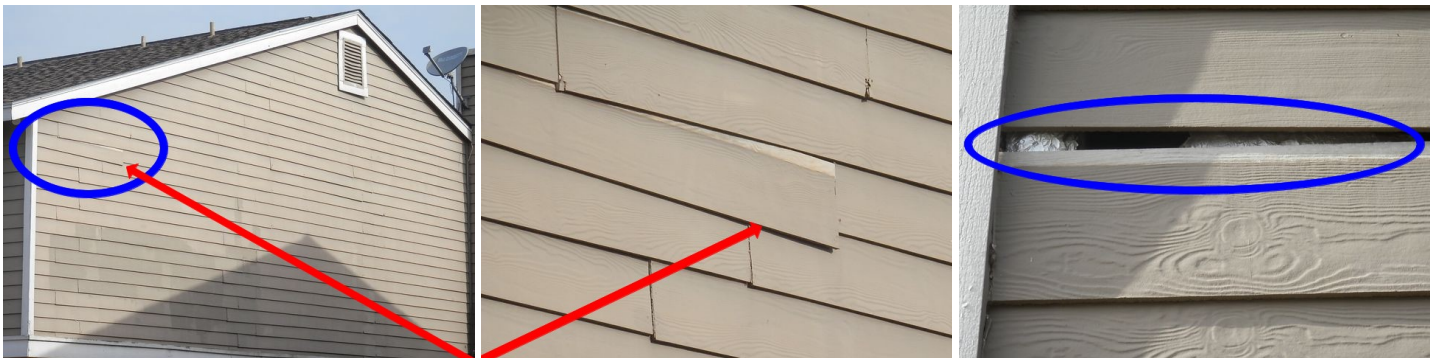
sample of loose siding and voids in the exterior veneer
