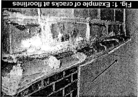
Fig. 1: Example of cracks at floorlines
