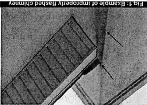
Fig. 1: Example of improperly flashed chimney
