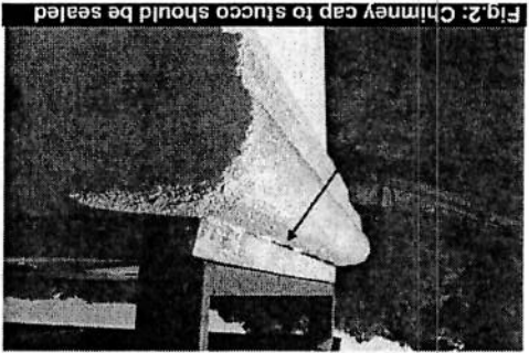
Fig. 2: Chimney cap to stucco should be sealed
