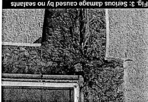
Fig. 3: Serious damage caused by no sealants
