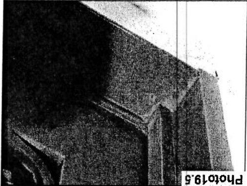
Door threshold, front elevation, no visible sealant
