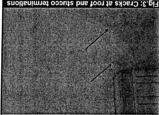
Fig. 3: Cracks at roof and stucco terminations
