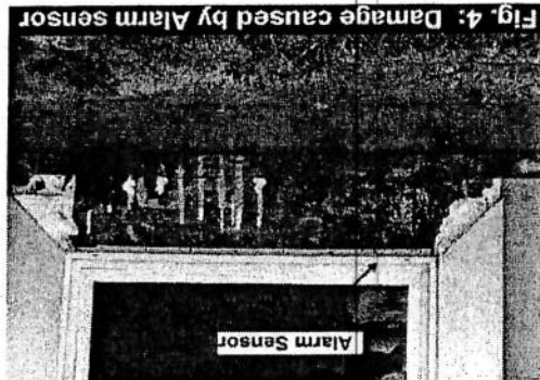
Fig. 4: Damage caused by Alarm sensor
