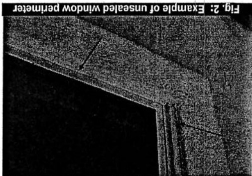
Fig. 2: Example of unsealed window perimeter
