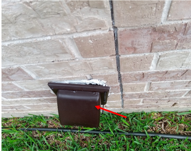
a. Loose dryer's louver vent cap (south wall) noted; recommend proper installation;
