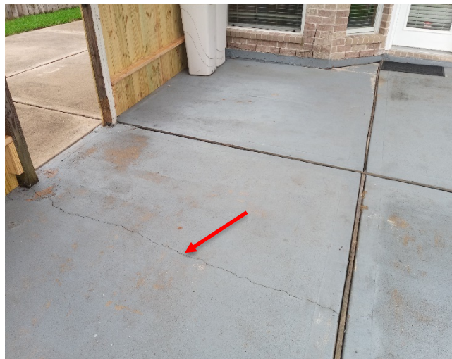
b. Observed concrete cracks at the back patio slab; this is common as concrete ages, and cracks observed are typical shrinkage/settlement cracks and not indicative of structural issue; it is recommended that this type of crack be sealed and monitored periodically to see if they increase in size, if it does, consult with a licensed structural engineer; Photo is representative of the issue and may not include all locations;
