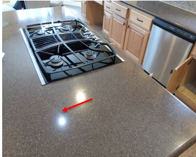
a. Noted a crack on kitchen granite countertop;
