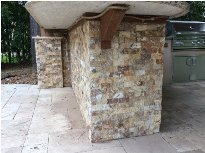
Outside kitchen counter appears to have excessive unsupported granite counter top
