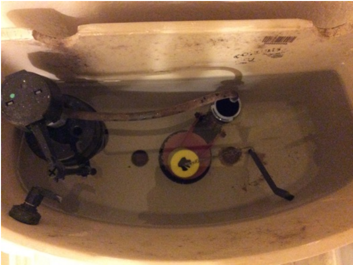
Broken toilet flush handle requires repair
