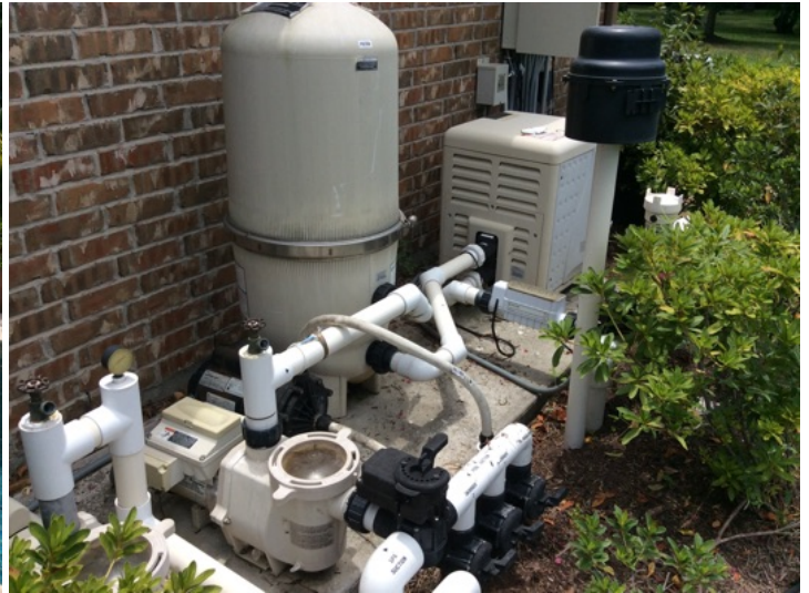
All three pumps and associated equipment are properly electrically bonded
