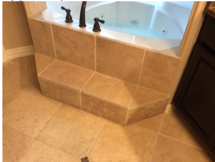
Observed there is no available access panel to service the jetted tub equipment
