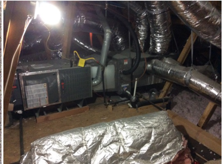
Downstairs furnace and air handling unit
