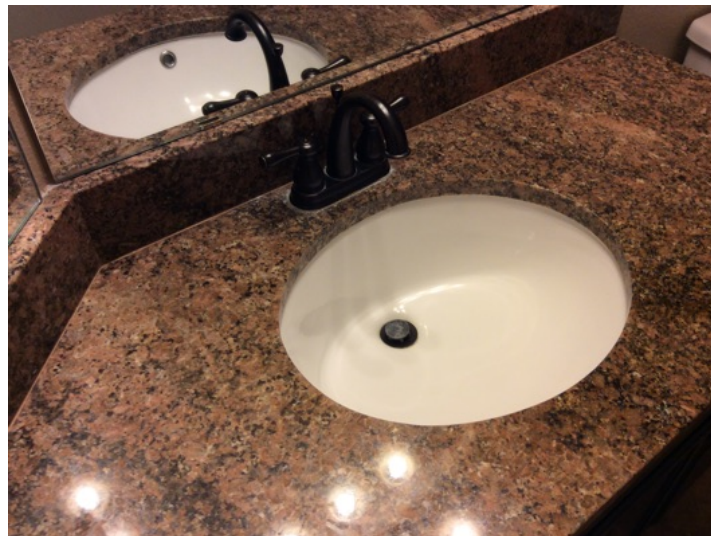
Upstairs back hall bath sink basin stopper requires repair
