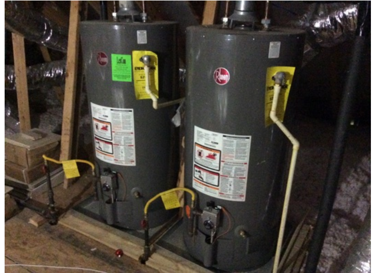
Twin Rheem water heaters piped in series
