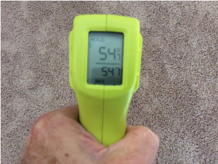
Upstairs cooling supply temperature 54°
