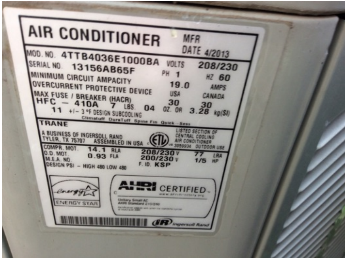
Trane air conditioner, 3 ton, manufactured April 2013, 14 SEER
