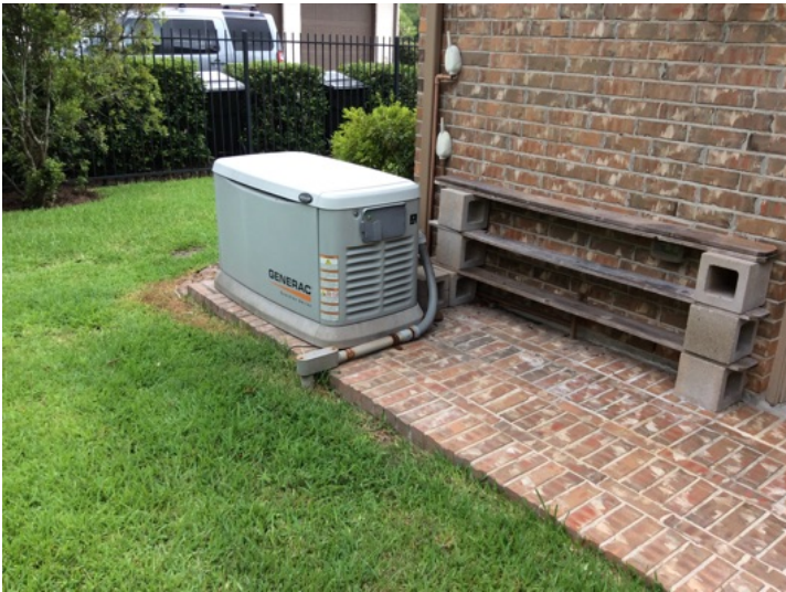
Auxiliary generator located behind the small garage
