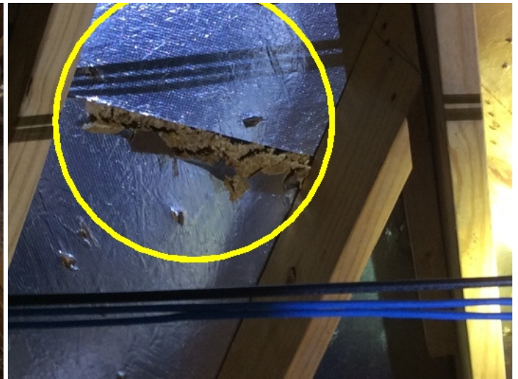
One area of OSB roof sheathing appears to be compromised as viewed from the attic
