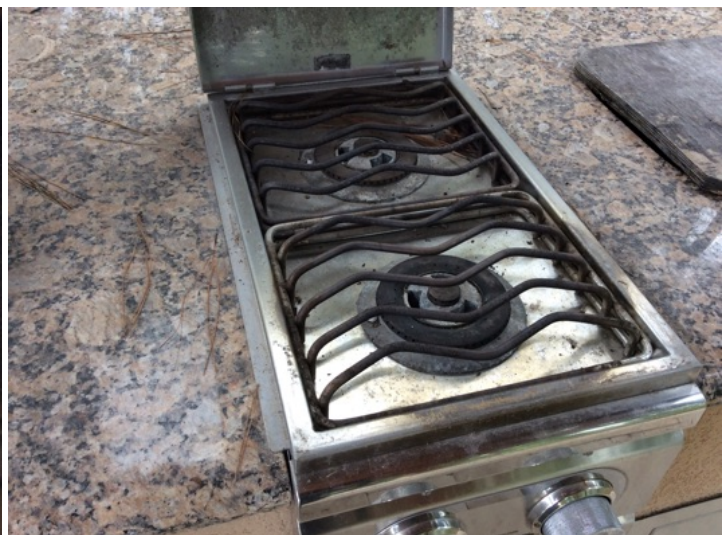
Was unable to light the burners in the outside kitchen
