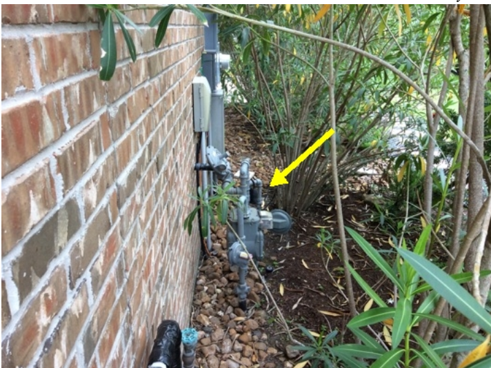
Gas meter on the east exterior wall
