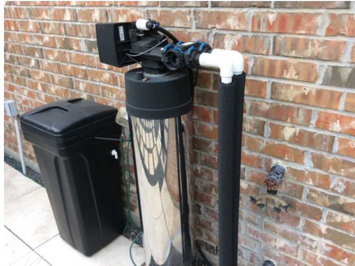
Water treatment system
