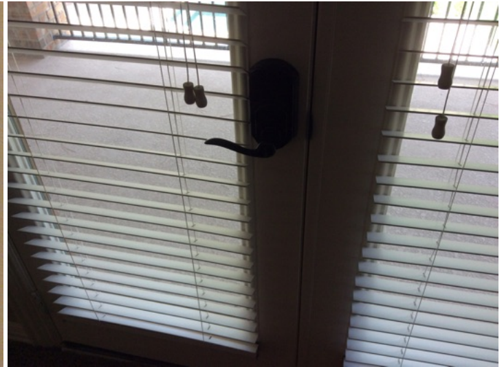
Back balcony door does not lock
