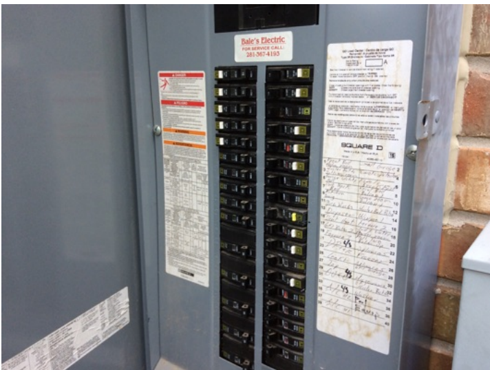
Main service panel, 200 amp, Square D
