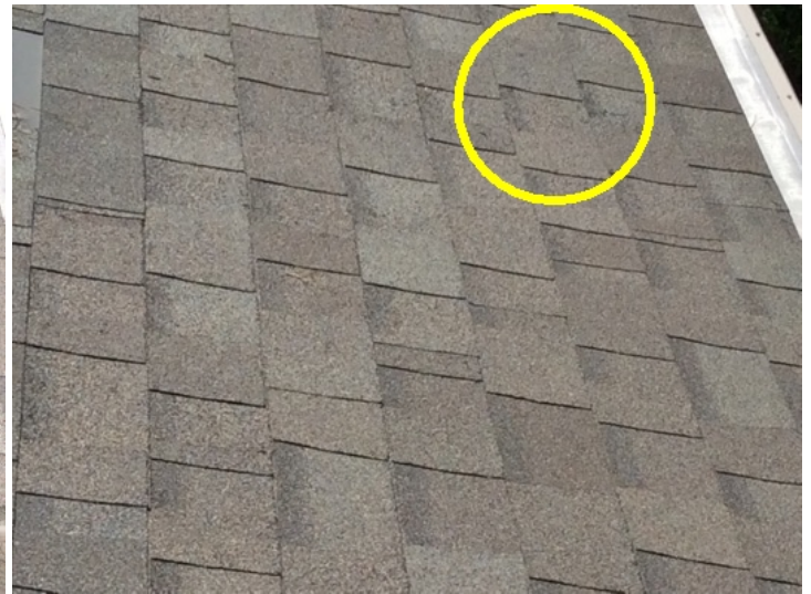
Apparent roof damage
