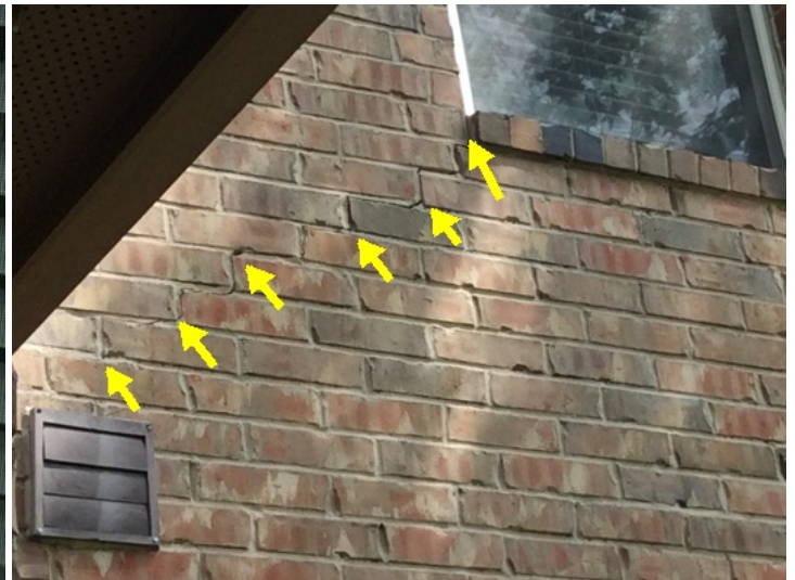
Mortar crack east wall
