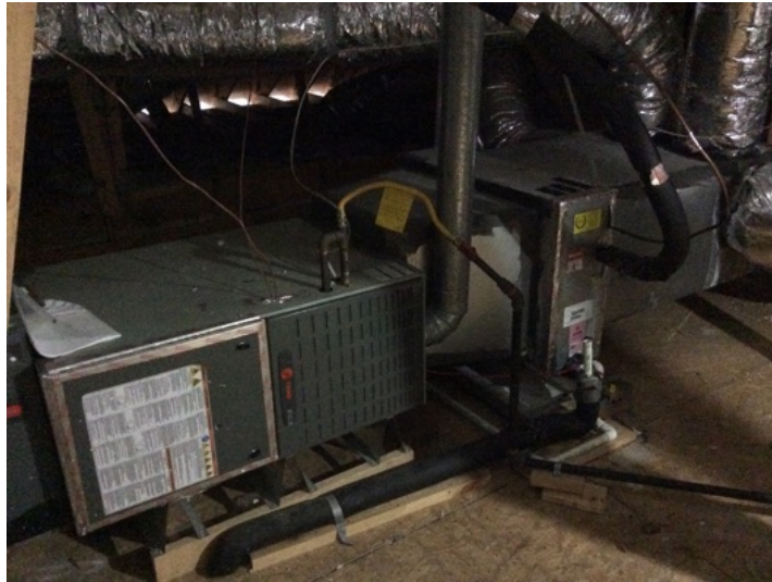
Upstairs furnace and air handling unit
