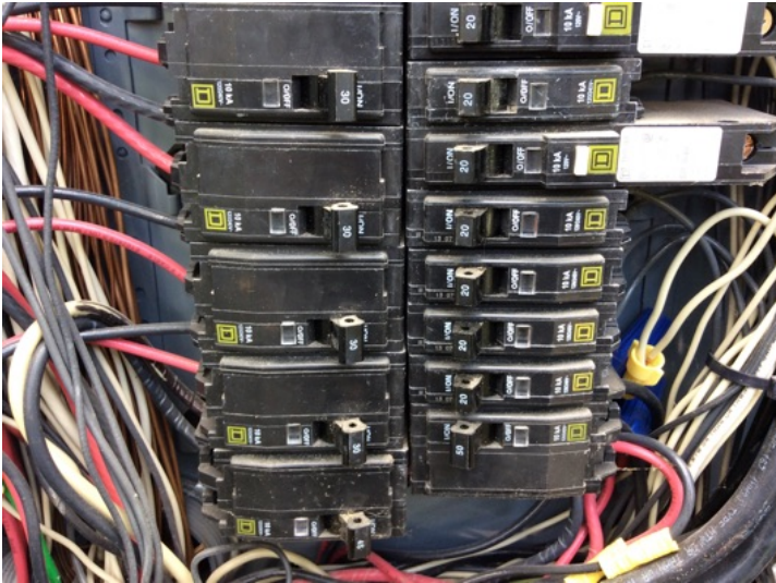
Square D, 200 amp, electric service panel
