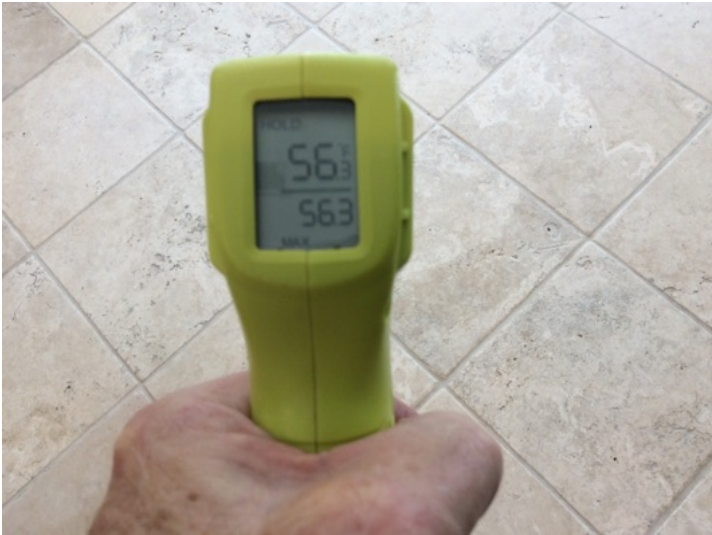
Downstairs cooling supply temperature 56°
