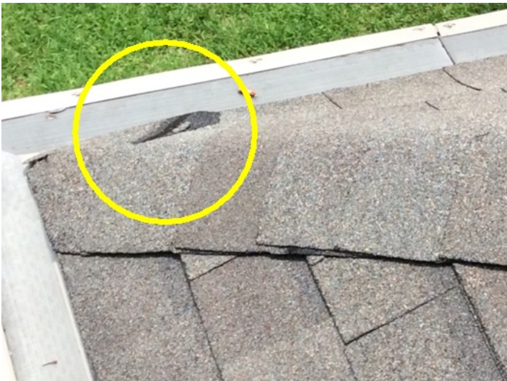
Damage to the roof
