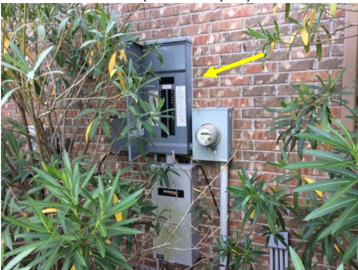
Electric service panel is located on the west exterior wall
