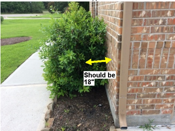
Vegetation and shrubbery is too close to the house
