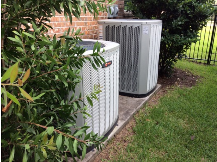
Twin air-conditioning systems
