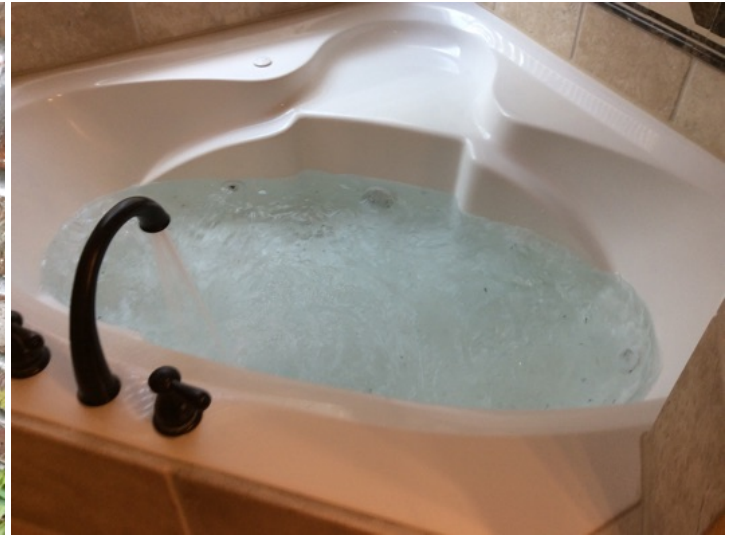
Jetted tub is operational
