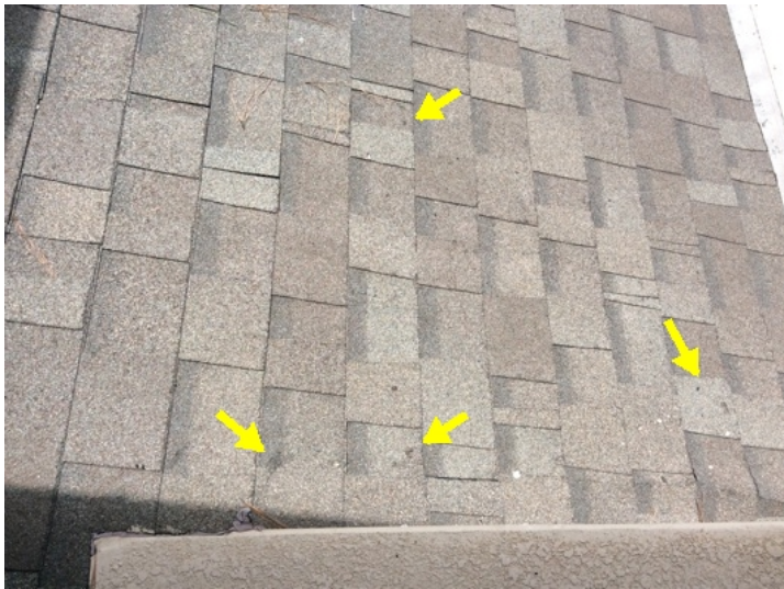
Apparent roof damage
