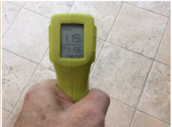
Downstairs heating supply temperature 119°
