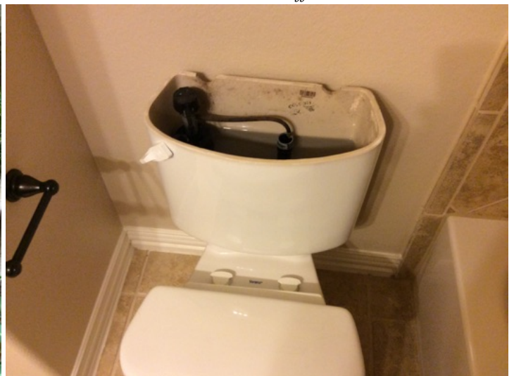
Upstairs hall bath toilet broken flush handle
