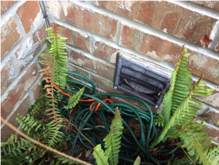
Broken exhaust vent from the equipment to the jetted tub
