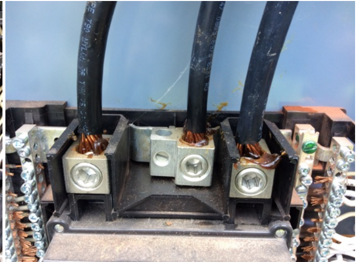
Copper service conductors, Square D, 200 amp, electric service panel
