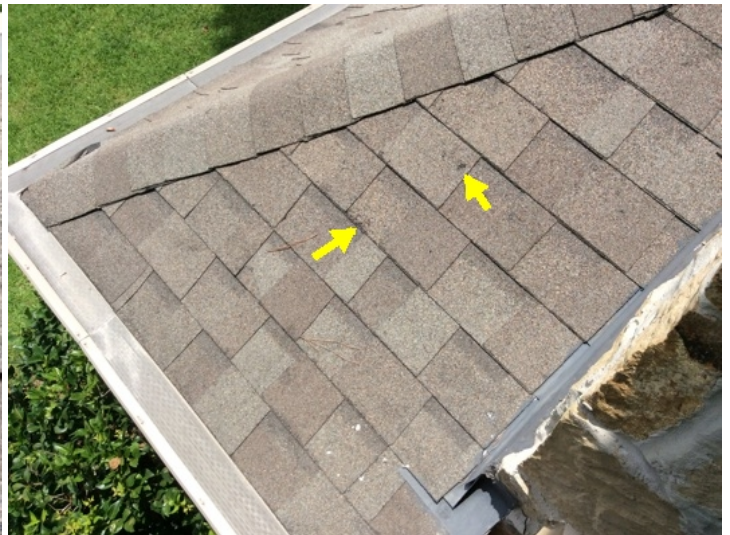
Apparent roof damage
