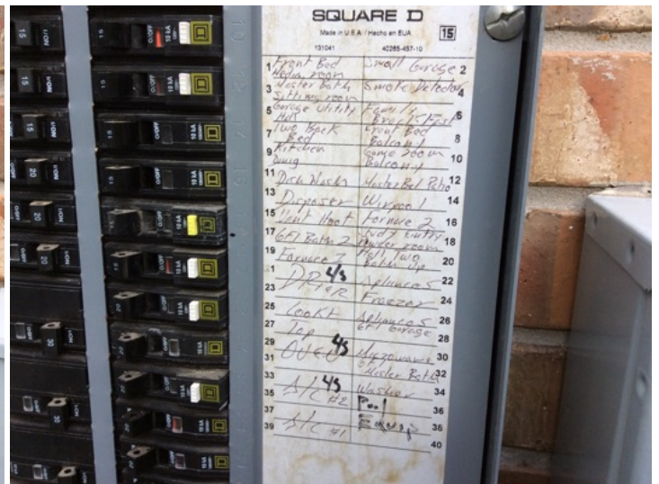
Noted the improper labeling in the electric service panel
