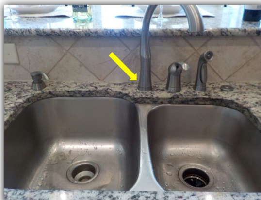
The bathtubs perimeters should be caulked.
