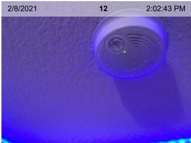
Wired Smoke Alarm (mfd 11/2005) | Smoke test: Passed | >10 yrs old
