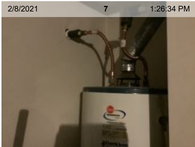
Gas Water Heater | >10 yrs old | Raheem | Water heater (with expansion tank if present)
