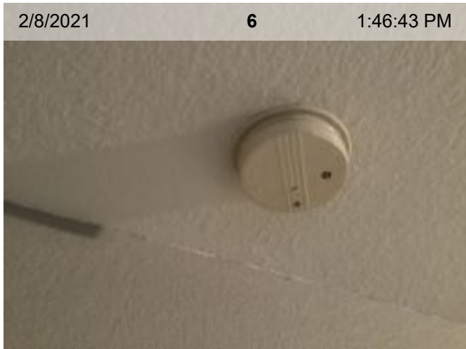
Wired Smoke Alarm (mfd 4/2005) | Smoke test: Passed | >10 yrs old | Alarm in place (on ceiling or wall)
