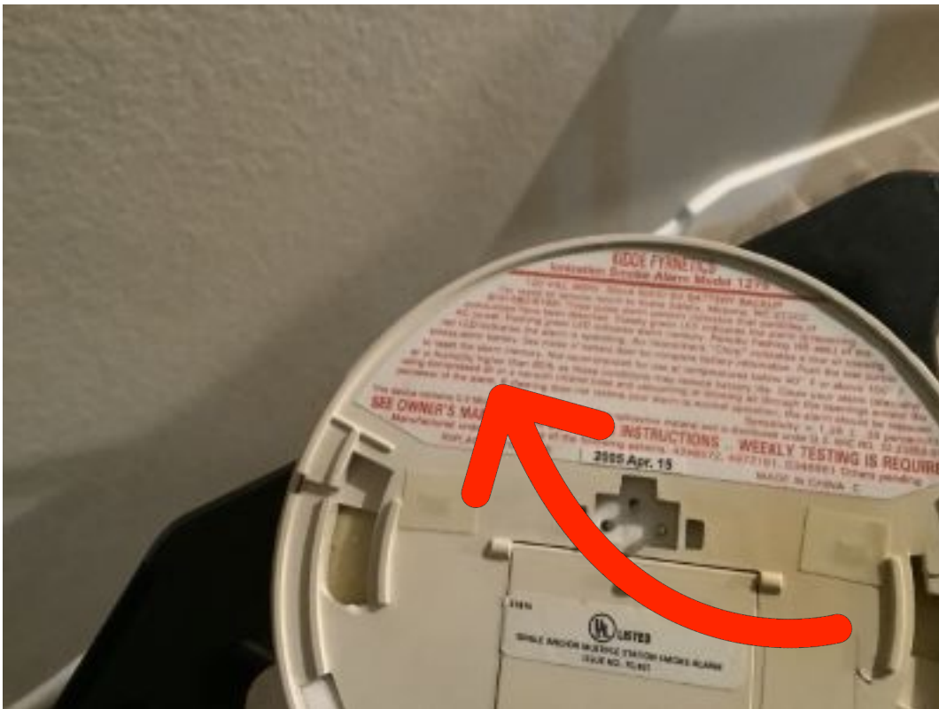
Hallway/Stairway Smoke Alarm Close-up of printed manufacture date (typically on back of alarm)
