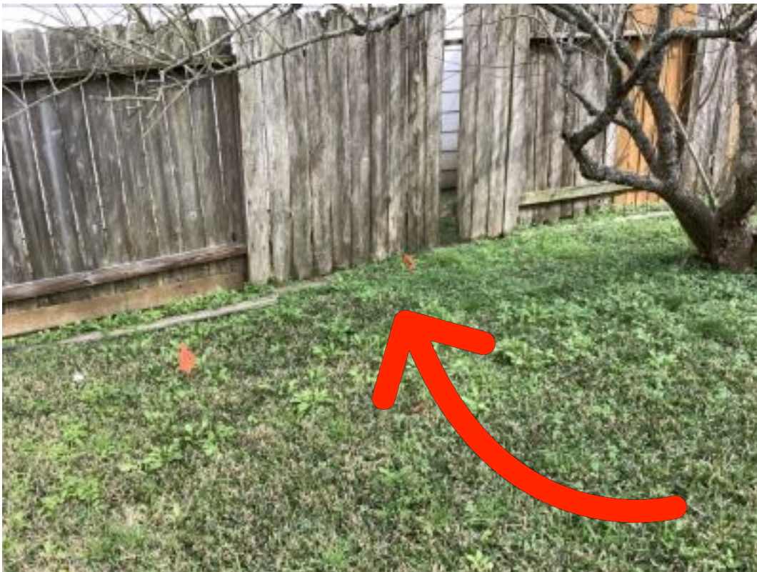
Rear Exterior Fence Damaged, rotten, or chipping fence materials; holes/gaps in fence; damaged clasps; gates that don't close securely
