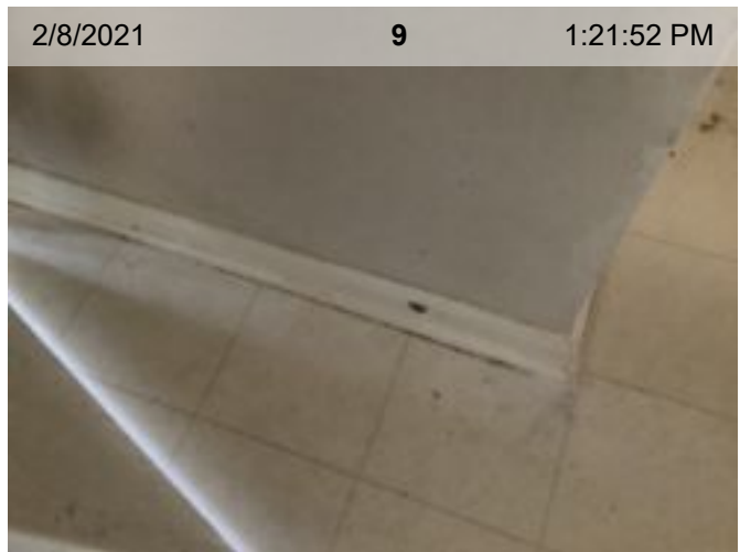
Door Stop | Door stop missing
