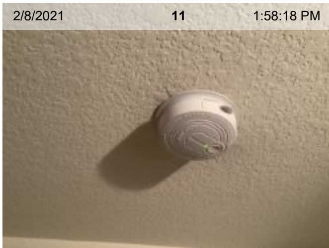
Wired Smoke Alarm (mfd 11/2006) | Smoke test: Passed | >10 yrs old
