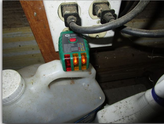
Loose outlet above kitchen counter.
