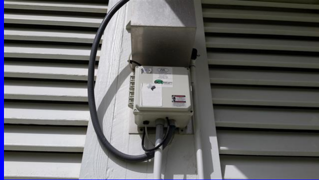
Aerobic septic system controls located on the left side of the home
