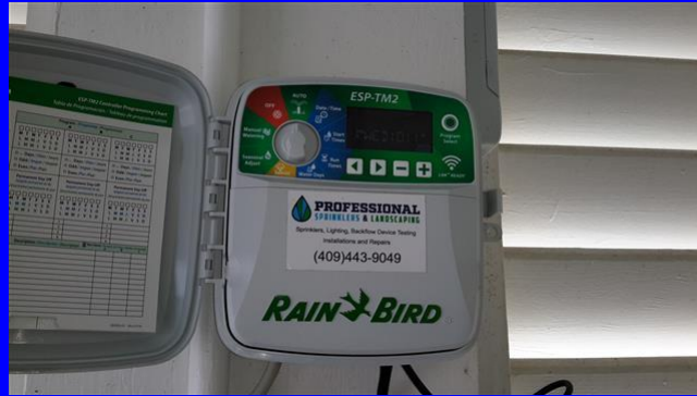
Sprinkler system controls located inside the garage on the left wall. 7 zones
