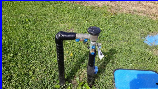
Sprinkler system backflow preventer and shut off valves located at the street on the right side
