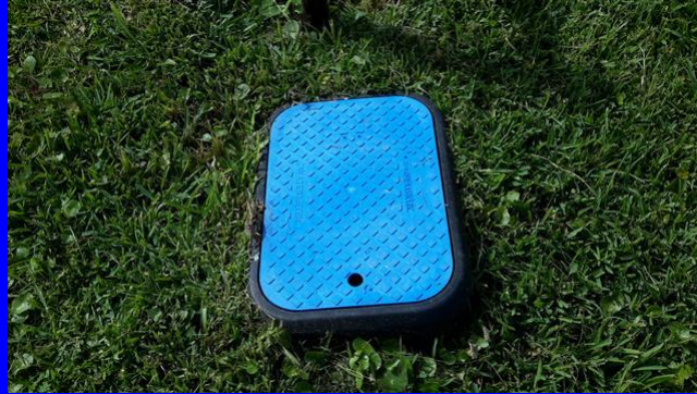
Water meter located at the street on the right side
