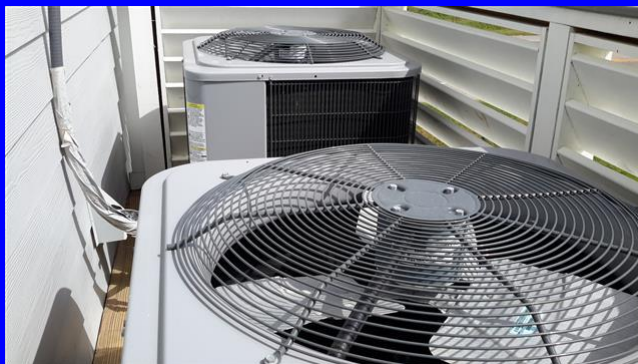
Two condensing units located on the left side of the home on elevated platform
