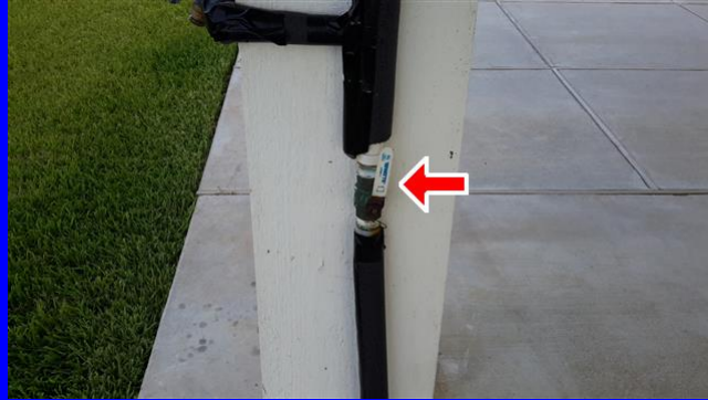
Main water shutoff valve located on the right side of the home
