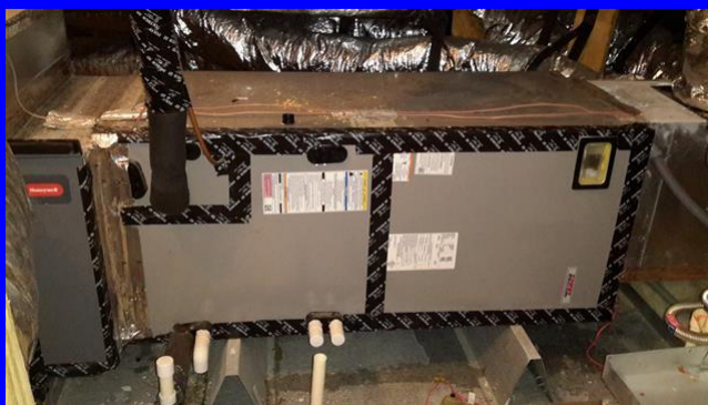
Heil electric furnace located on the left side of the attic
