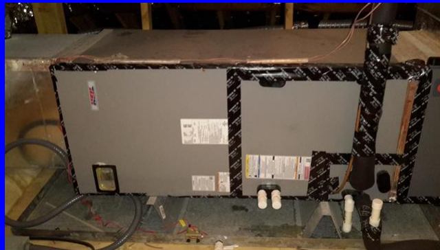
Heil electric furnace located on the right side of the attic
