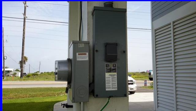
Underground electrical service entrance and main circuit breaker located on the right side of the home
