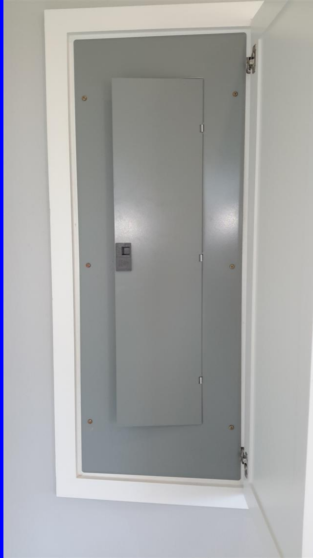
Electrical panel located inside the master bedroom on the left wall
