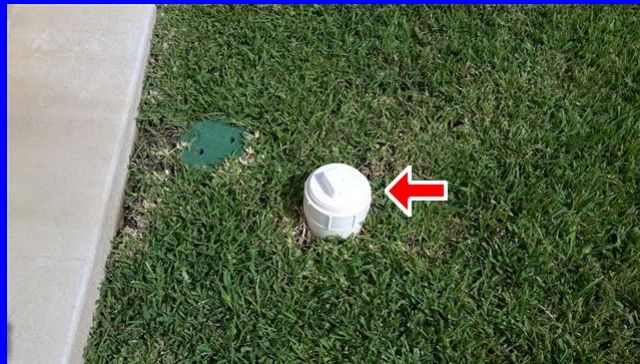
Septic clean out located on the left side of the home
