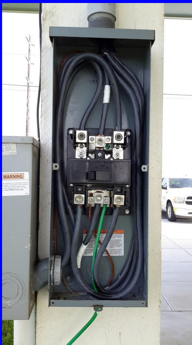
inside the main circuit breaker box
