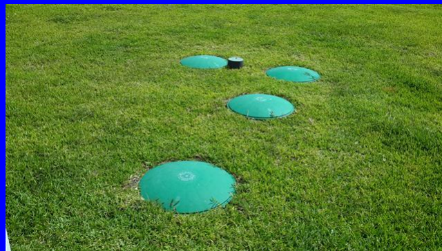
Septic tanks located on the left side of the home
