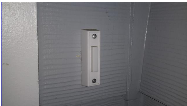
B. Item 2(Picture) doorbell is nonfunctional.
