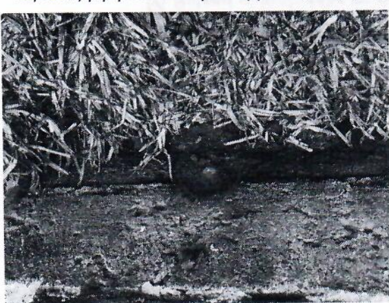
Post tension cable ends exposed right master
