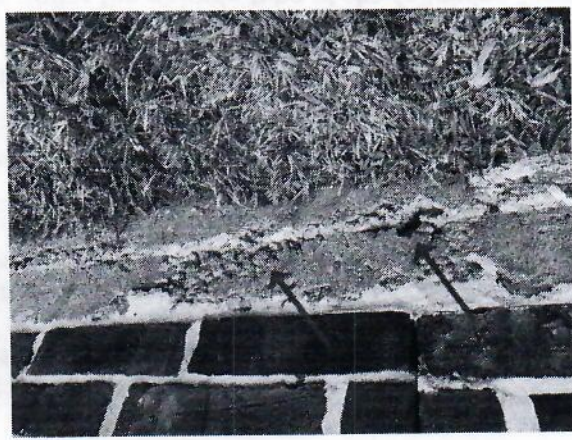
Honeycomb left perimeter slab
