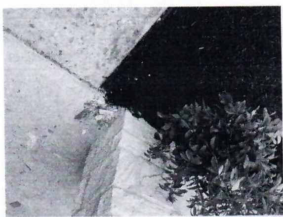
High soil levels front porch column
