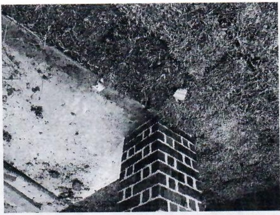
High soil levels rear patio column
