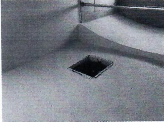
Exhaust fan vent cover missing upstairs bath
