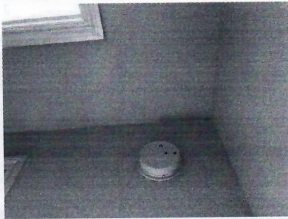
Upstairs hallway smoke detector not CO too
