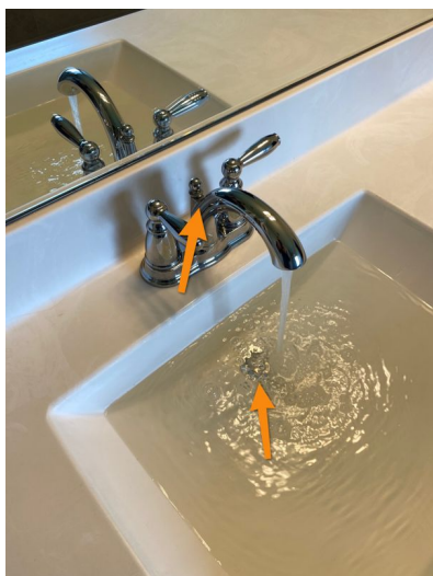
Master bathroom drain stop is not connected to each other
