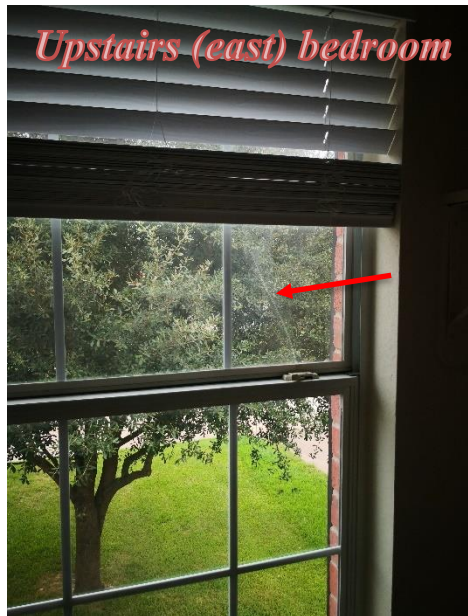
a. The inspector noted a cracked window pane (upstairs SE bedroom); recommend window replacement;
