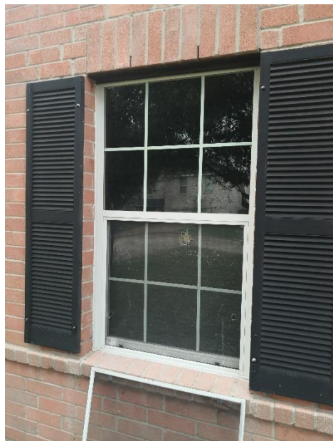
b. Certain windows (mostly in downstairs) closed by themselves when tested, this is possibly caused by loose/damaged window sash springs ; it is suggested that the client consult with a specialist for further evaluation; Also recommend installation of missing screens at all windows; Photo is representative of the issue and may not include all locations;
