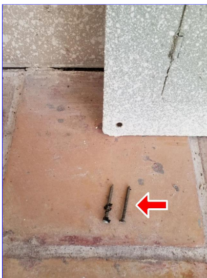
A. Item 5(Picture) Main service panel
