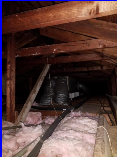
Electric furnace unit #2 (Right side of home)
