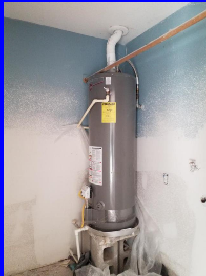
40 gallon gas water heater, located in the washer dryer room
