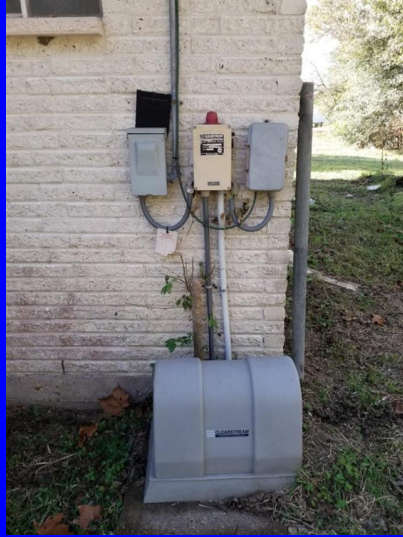
Septic system control panel, located rear of home
