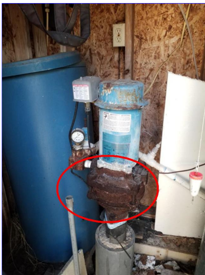
D. Item 3(Picture) Water well pump
