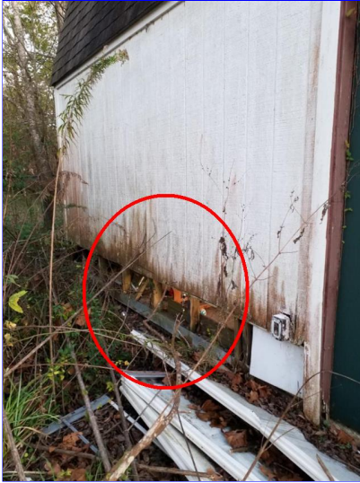
C. Item 1(Picture) Left side
