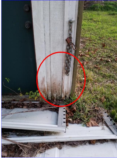
C. Item 2(Picture) Left side
