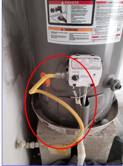
C. Item 2(Picture) Water heater
