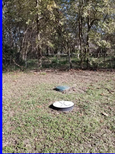
Septic system tanks, located rear of home
