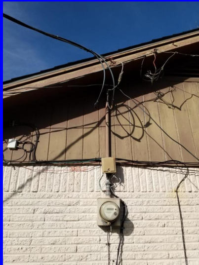
Overhead service, located front right side of home
