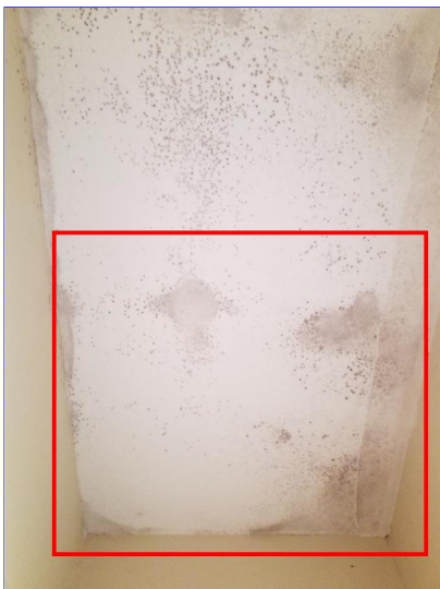
F. Item 5(Picture) Master bathroom shower
