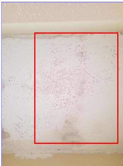
F. Item 4(Picture) Master bathroom shower
