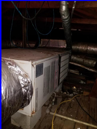
Gas furnace unit #1 (Left side of home)
