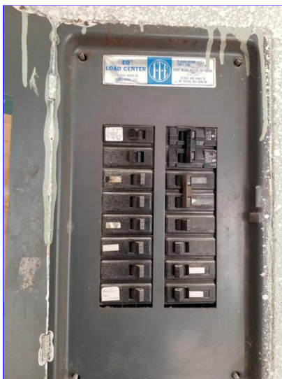
A. Item 3(Picture) Main service panel
