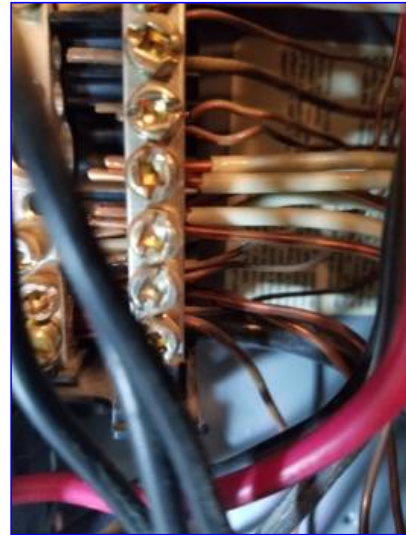
Observed multiple grounded (white) conductors terminated beneath a single lug on the neutral busbar. The conductor terminations were only rated for the termination of one conductor per lug. This causes an issue with the continuity of the homes electrical system when an attempt to isolate a single circuit is desired.
