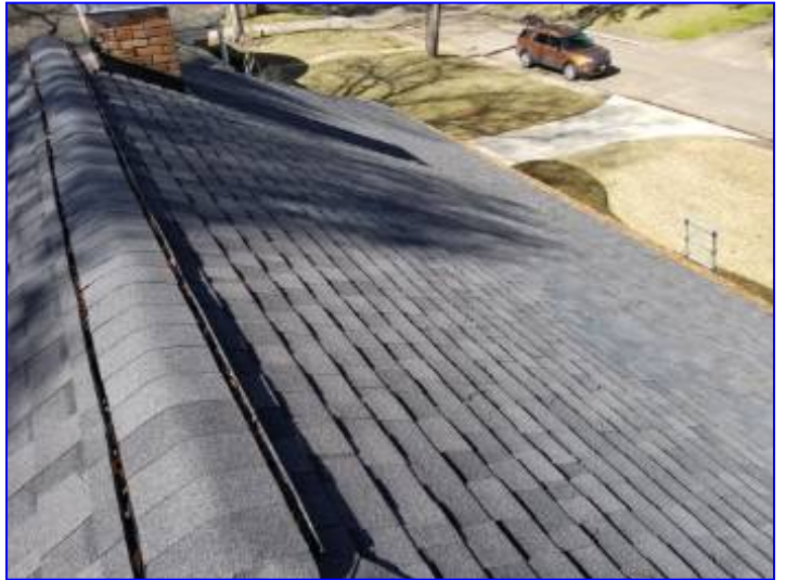
All visible roofing materials appeared to be properly installed at time of inspection.
