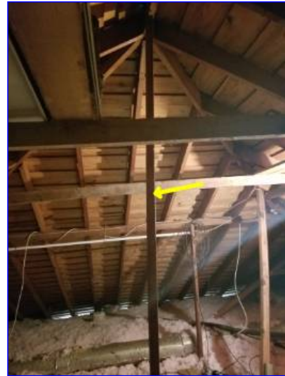
Braces that support the ridge that are longer than 8 feet long should be doubled in a Tee formation. Improvements are recommended to better support the ridge of the roof.
