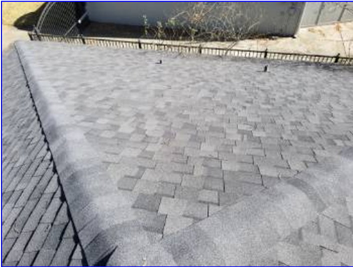
All visible roofing materials appeared to be properly installed at time of inspection.
