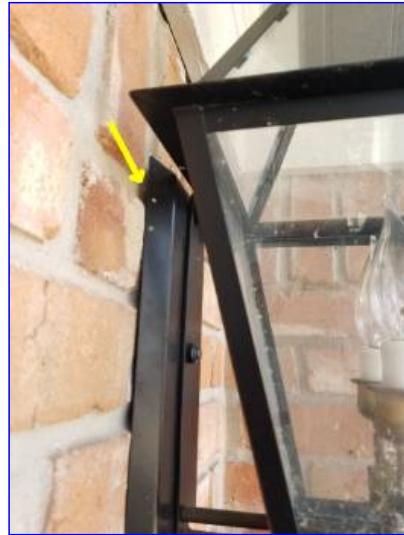
All exterior wall penetrations should be sealed. Failure to keep all penetrations properly sealed may lead to water intrusion to interior walls. This is a common maintenance item and all penetrations should be checked periodically.
