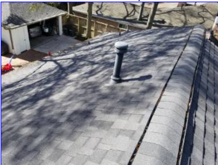
All visible roofing materials appeared to be properly installed at time of inspection.
