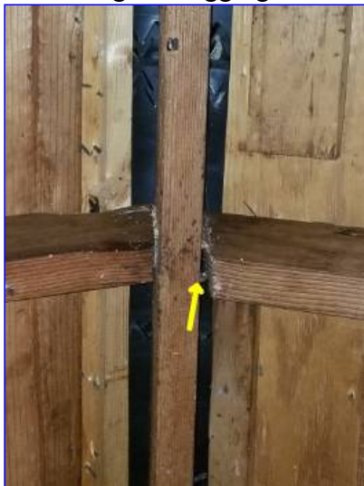
The rafters do not have adequate support at the ridge. Rafters that are cut improperly or do not fully bear should be repaired. This condition appears to be related to improper cuts during construction rather than to roof structure movement, as evident by the fact that they are scattered and not consistent.
