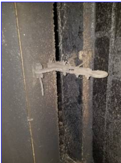
Creosote build-up was noted in the fireplace flue and/or firebox. Cleaning of these areas should be undertaken for improved safety.
