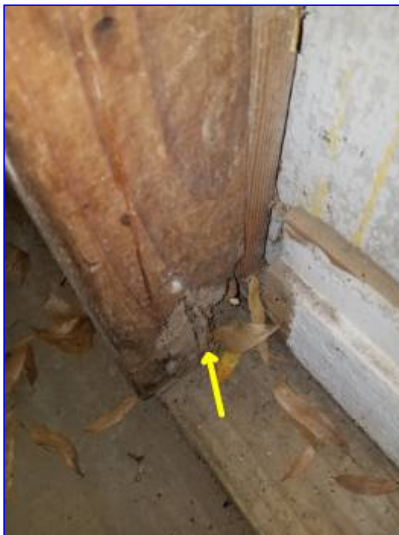
Observed evidence of wood destroying insects in the garage. Several wall studs are severely damaged. Further investigation by a wood destroying specialist is recommended. Repairs to the damaged wall studs are recommended.
