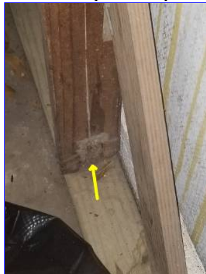
Observed evidence of wood destroying insects in the garage. Several wall studs are severely damaged. Further investigation by a wood destroying specialist is recommended. Repairs to the damaged wall studs are recommended.
