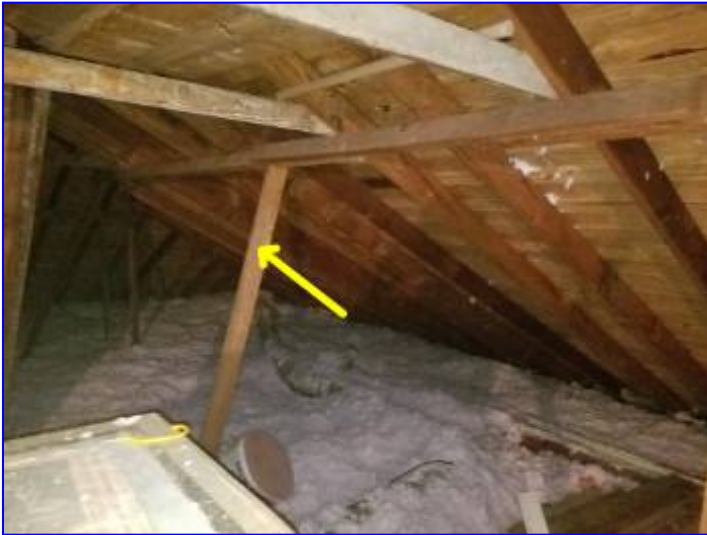
Today's building standards require purlin struts to be spaced no further than 4 feet on center. Additional supports are recommended if the roof begins to show sign of sagging.
