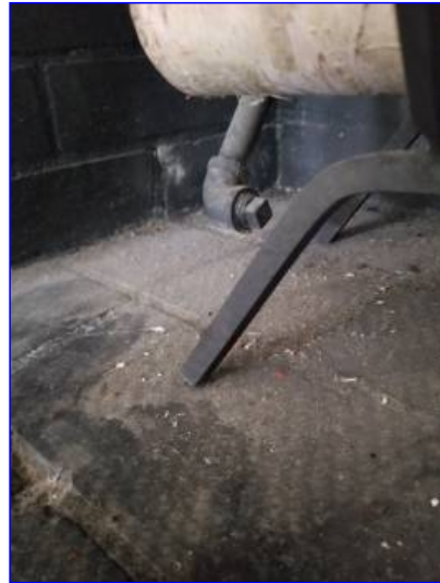
The gas log lighter has been capped off.
