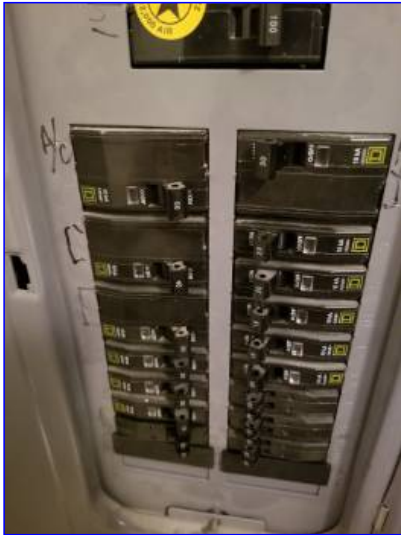
Current standards call for arc fault protection on outlets in living areas. No arc fault protection is supplied. Recommend updating to these standards.
