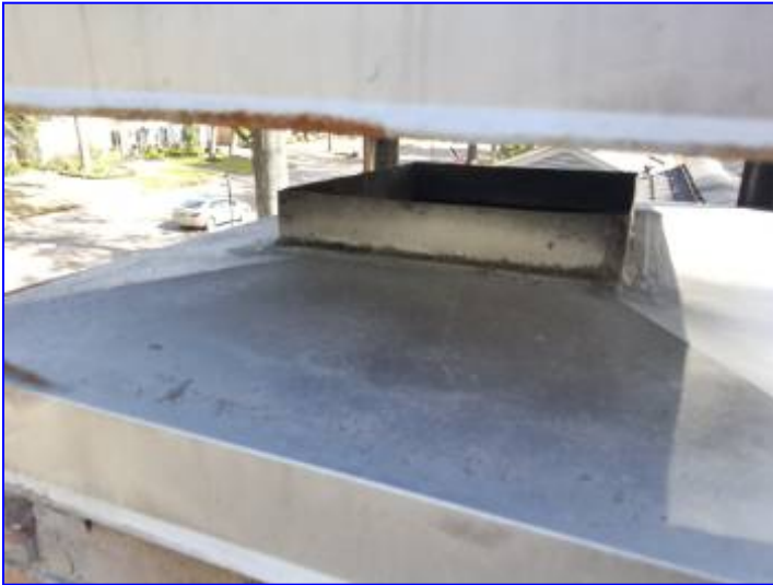
It is recommended that the chimney cap be screened to keep critters out.
