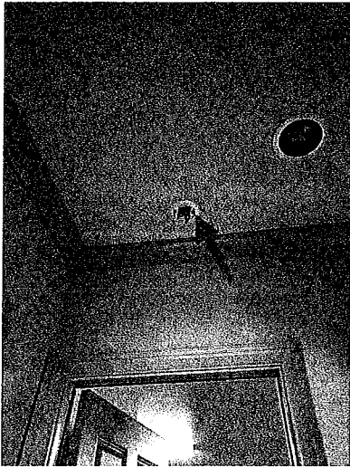
Missing smoke detector
