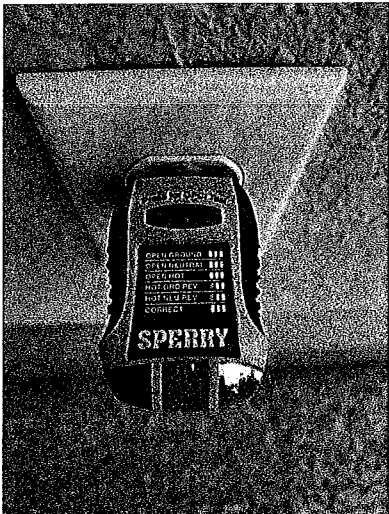
Upstairs bedroom was found to have an open neutral. The neutral provides a safe path for electricity back to the main panel.
