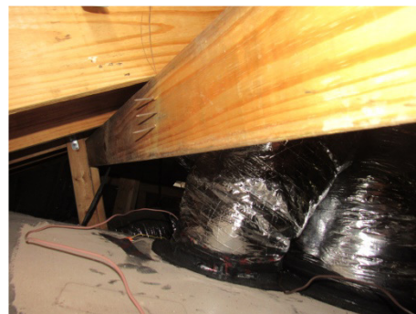
Missing roof brace
