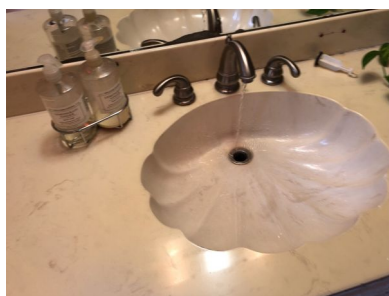
2nd Floor Bathroom Cold Water
