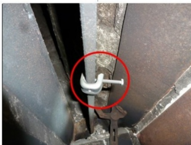
HEI file photo showing c-clamp in masonry fireplace
