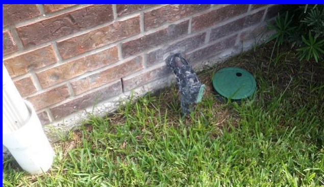
Main water shutoff
