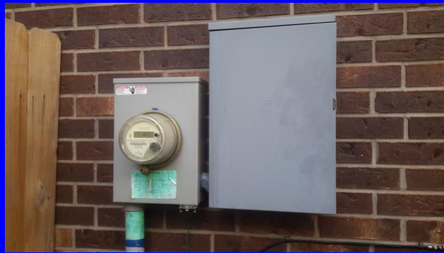
Electric meter and main panel
