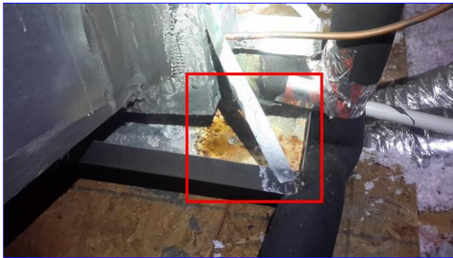
B. Item 1(Picture) Drain pan
