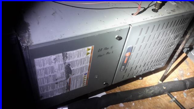
Trane furnace in attic
