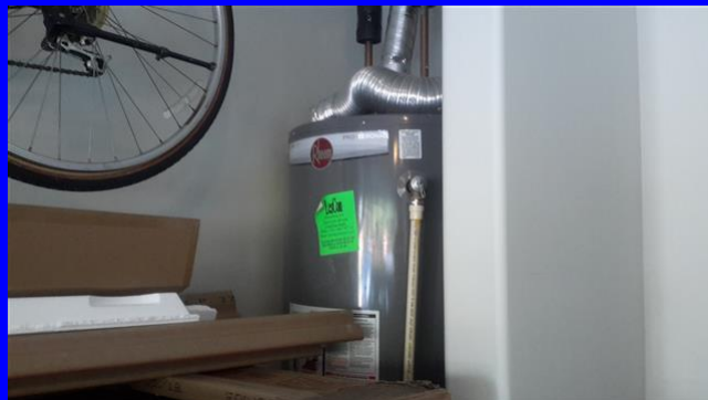
Water heater in garage
