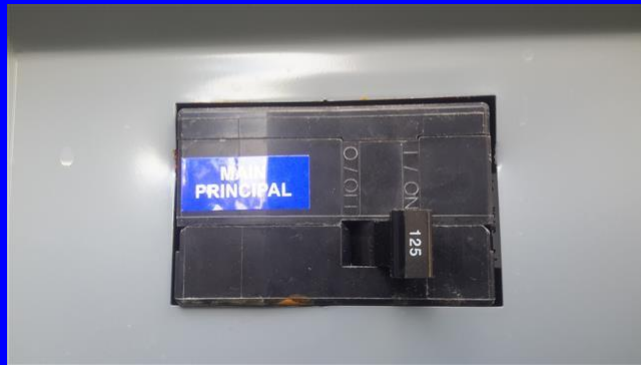
125 amp main service disconnect outside
