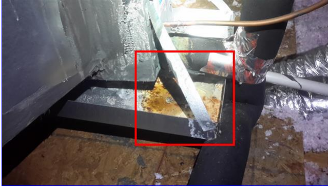
B. Item 1(Picture) Drain pan
