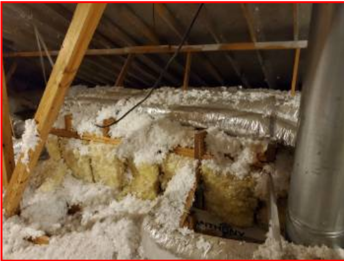
Ductwork should not be touching.
