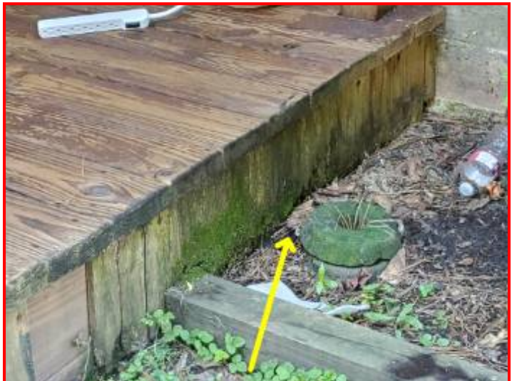
Boards need replaced
