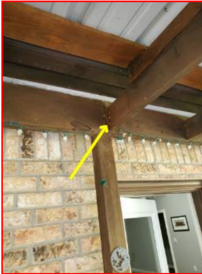
Ceiling joist hangers should be installed.
