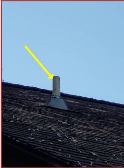
Vent pipes should be painted to protect them from UV rays.
