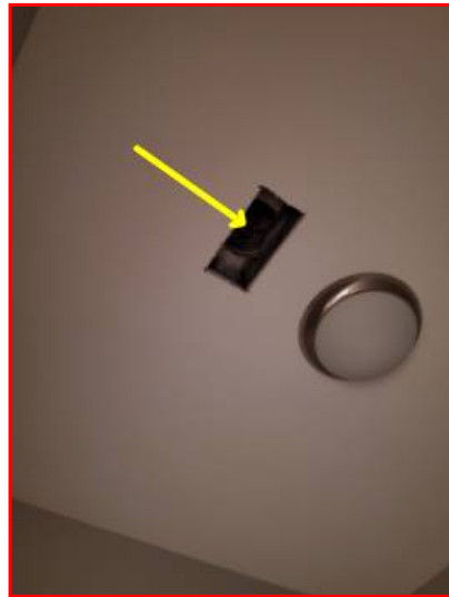
Register(s) was missing.
