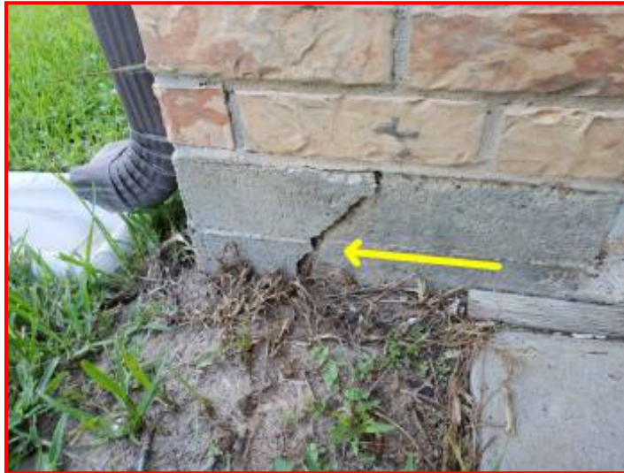
Corner cracks noticed. Not uncommon to see.
