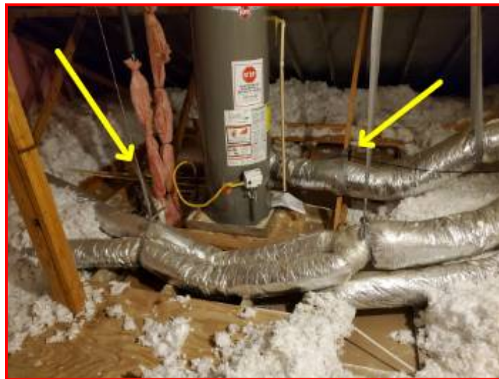
Insulation is missing in spots. Should be replaced.
