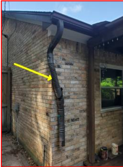
Gutter downspout not installed correctly.
