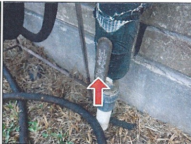
Main water shut off located left side of residence.
