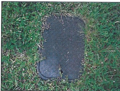
Main water meter located front left of residence.
