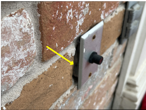
Recommend caulking all exterior penetrations to the house.
