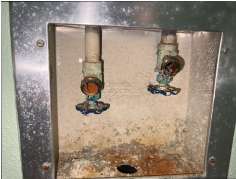
Corrosion observed on shut off valves to laundry connections.
