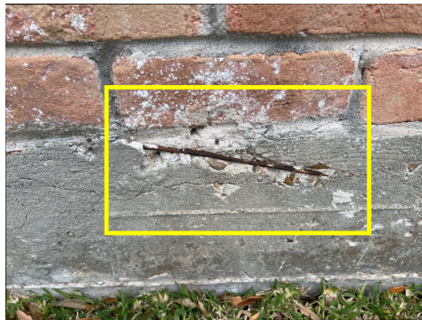
Exposed steel observed at west side of house.
