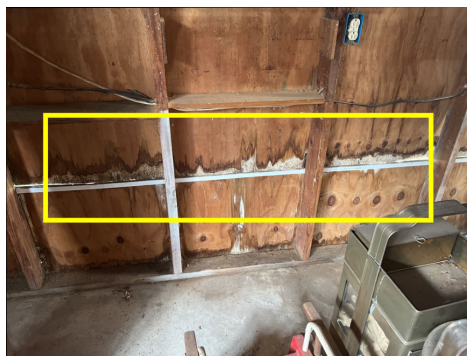
Water penetration observed at the interior wall garage.
