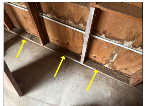
Sill plates are missing proper anchor bolts in the garage.
