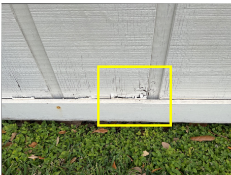
Wood rot observed at exterior west side wall of garage.
