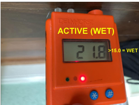
Moisture meter reading of floor in study (near front door).
