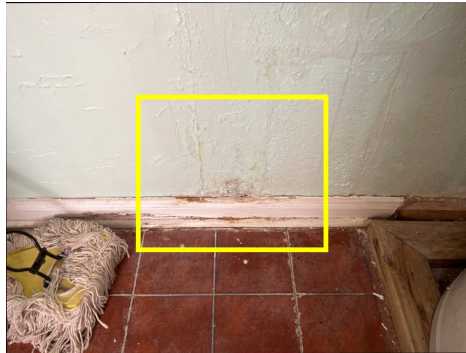
Water stains observed in utility room, moisture meter indicated that stains are not active (wet) at the time of inspection.
