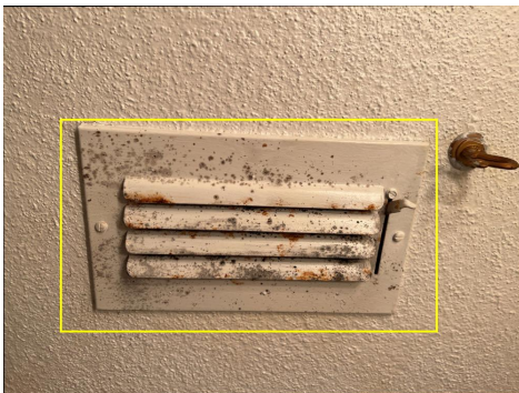
Microorganism growth on air supply grills / vents in upstairs hall bath which may be a concern due to increased awareness of environmental issues associated with molds. Recommend having an air quality/mold inspection done in the near future.
