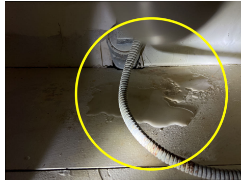
Water leaks under the kitchen sink.
