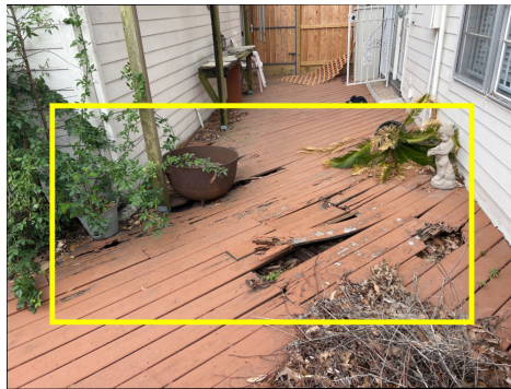
Multiple boards of wood decking are damaged due to wood rot recommend repair.
