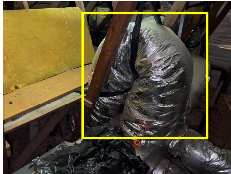
Flex ducts observed to be improperly routed with sharp bends and/or excess material in bends.
