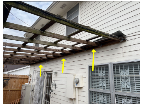
Patio cover does not appear to be properly secured - missing lag bolts to secure ledger board to structure.
