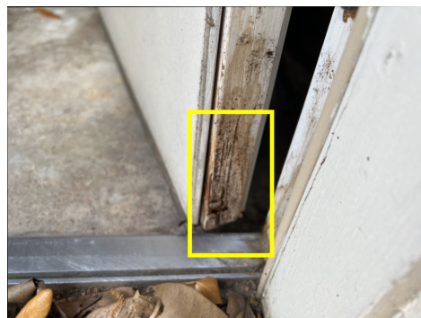
Wood rot observed at the bottom of the garage pedestrian door.
