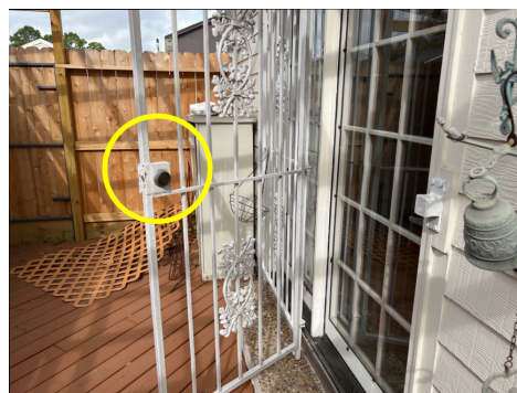
Exterior door with burglar bars, doors do not open without a key of locked.
