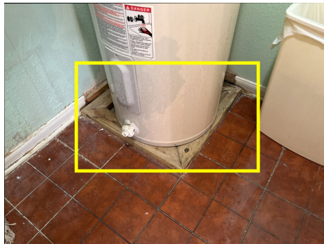
No drain pan under the water heater in utility room.
