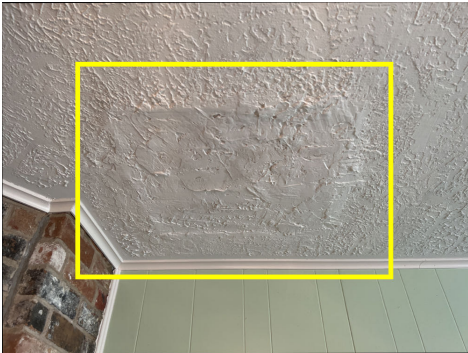
Observed patch repair to the ceiling in living room.
