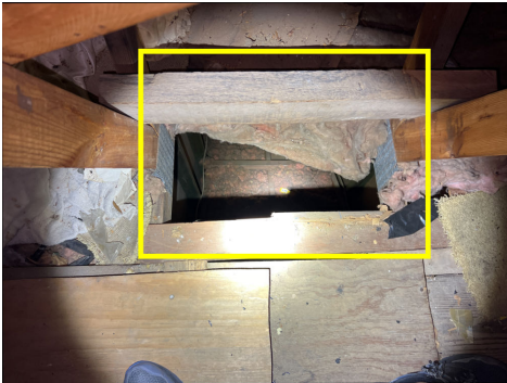
Observed open Chase an attic recommend it be sealed.
