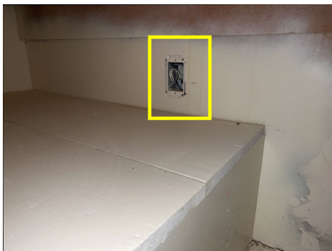
Wire splice missing cover left of kitchen sink under the cabinet.
