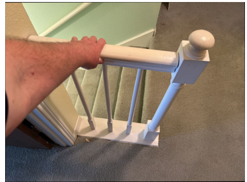
Railing at the upstairs landing is loose.
