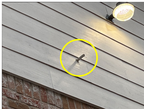
Observed an abandoned drain line at west side of house.
