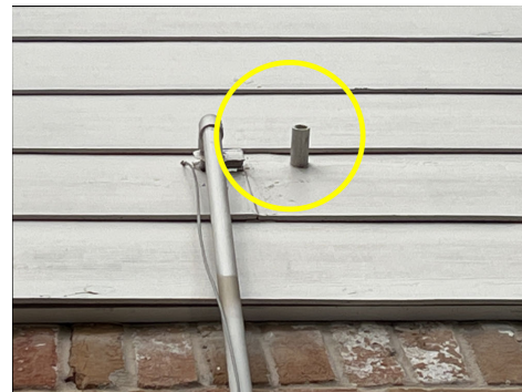
Missing 90 degree elbow fitting on end of emergency drain line at east exterior wall to prevent condensation dripping back onto the exterior wall.
