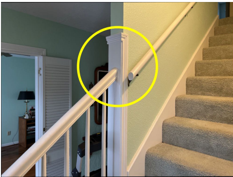
Hand railing is not continuous railing should be continuous the full length of the stairs.
