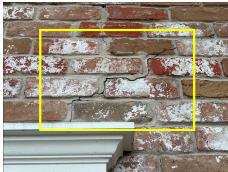
Brick crack observed over study window, north side of house.
