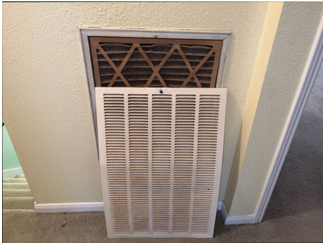
Return air chase grill was observed damaged and missing the screws which secured to the wall.
