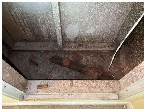
Return air chase is dirty, needs cleaning.
