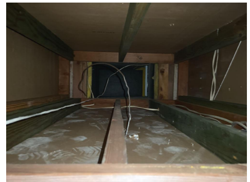
The return air chase is not properly sealed.
