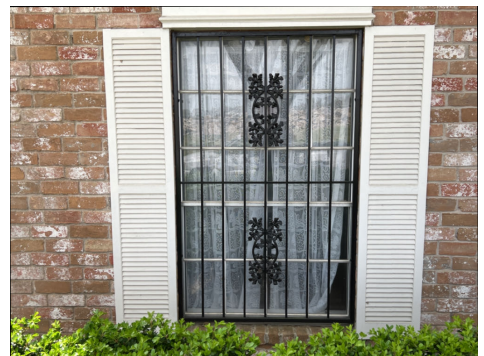
Burglar bars observed on study window and formal dining room window. Bars are affixed to the house and do not open.
