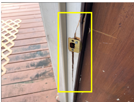
Damage door jam from forced entry at garage pedestrian door.
