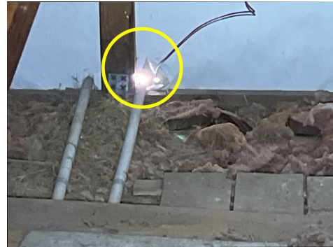
Daylight observed in the attic. Recommend sealing this area to prevent rodent entry.
