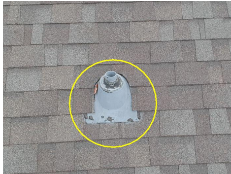
Drain waste vents should be a minimum of 6" above the roof line.
