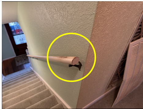
Hand railing should return to the walls as per current building code.
