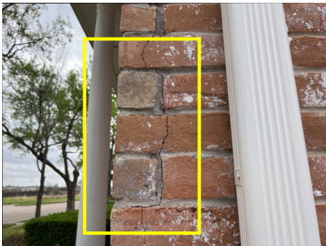
Brick crack observed at front northwest corner of house.
