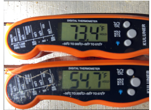
Temperature Split: 18.7 degrees (proper temperature split is between 16 to 24 degrees).
