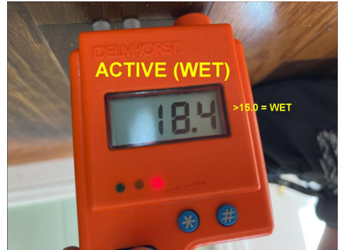
Moisture meter reading of floor in breakfast nook.
