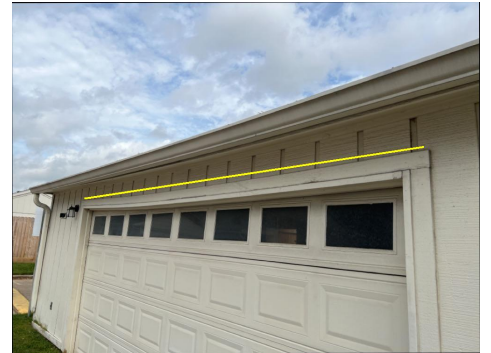
Observed sag in the double header over garage door, possible indication of improper/inadequate framing.
