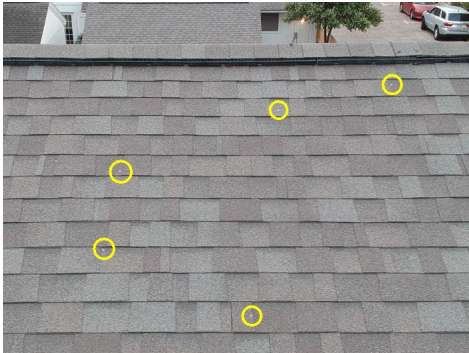
Multiple exposed nail heads observed on the roof.
