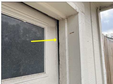
Observed gap at side of garage door.
