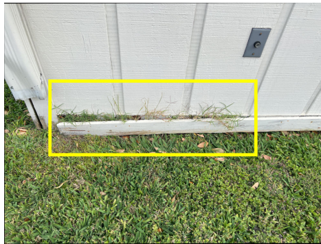
Trim / siding observed to be not secured in place; SW corner of garage.
