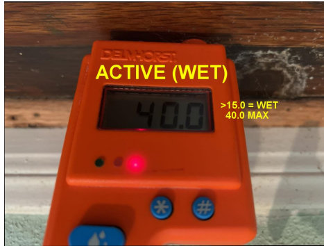
Moisture meter reading of floor in kitchen.
