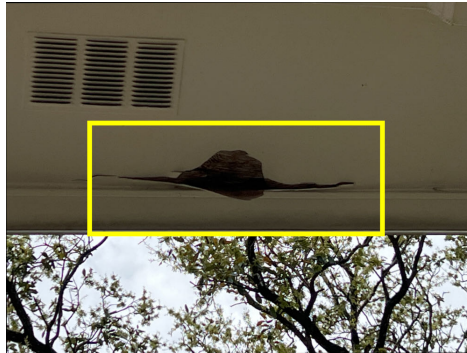
Area of wood rot observed at the soffit if the front porch.
