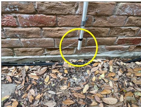
Primary drain line should not be allowed to discharge water right next to the foundation; east side of house.
