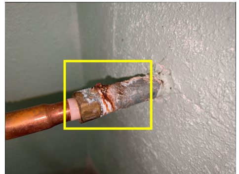
Corrosion observed on piping to water heater.
