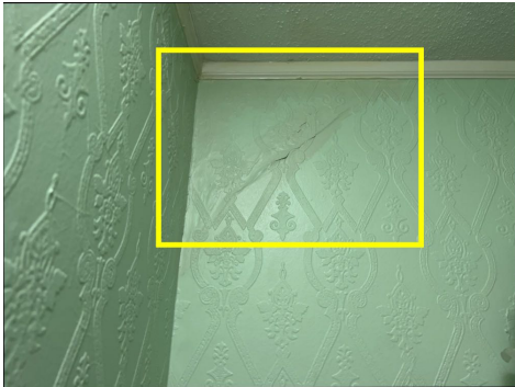
Water stains observed in half bath, moisture meter indicated that stains are not active (wet) at the time of inspection.
