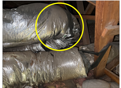
More flex ducts observed to be improperly routed with sharp bends.
