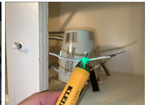
Wire improperly terminated above kitchen sink. Wired we're not hot (live) at time of inspection.
