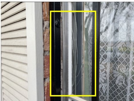
Cracked glass observed at front window of house in formal dining room.
