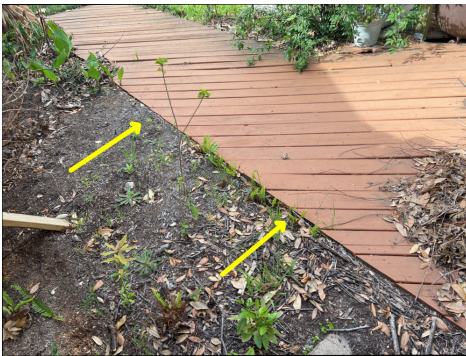
Patio decking is in contact with the ground which is kind do use it to wood rot.
