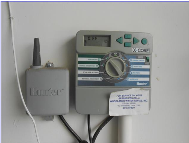
A. Item 2(Picture) View of sprinkler system controller
