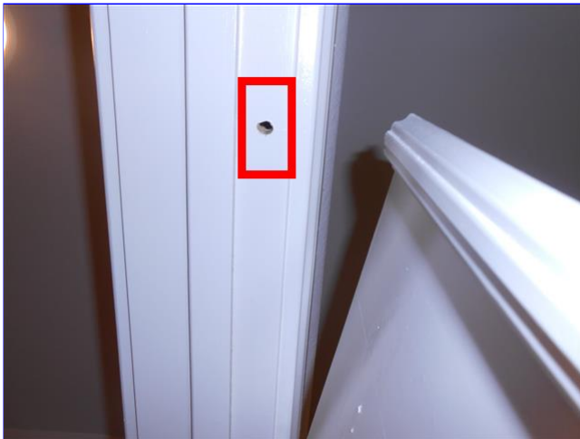
G. Item 1(Picture) Missing locking plate
