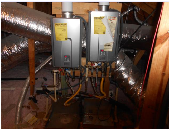
C. Item 1(Picture) View of the water heaters
