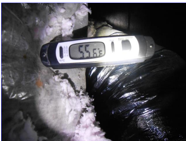
B. Item 5(Picture) View of the first floor cooling system measured exit air temperature at the evaporator.
