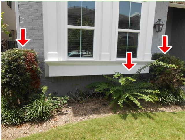
E. Item 2(Picture) Excess vegetation needs to be trimmed back
