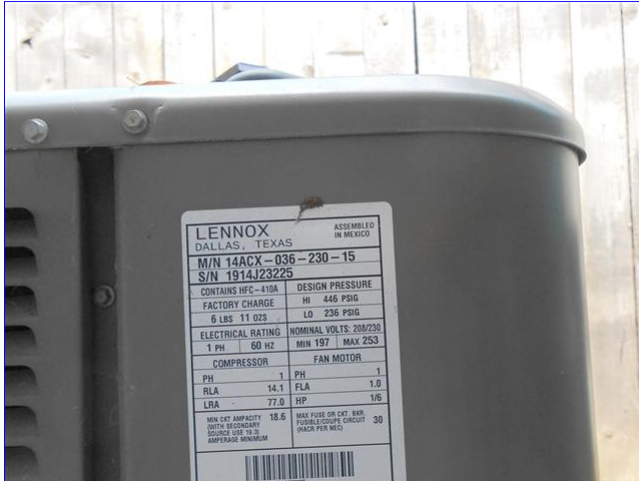
B. Item 1(Picture) View of the first floor cooling condenser information label
