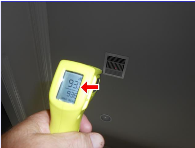
A. Item 4(Picture) View of the furnace temperature measured at a outlet register.
