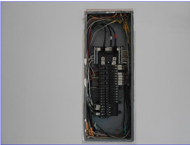
A. Item 2(Picture) View of the breaker panel open for inspection
