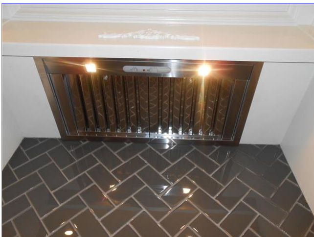
C. Item 1(Picture) View of the range exhaust vent.
