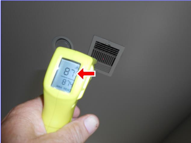
A. Item 3(Picture) View of the furnace temperature measured at a outlet register.
