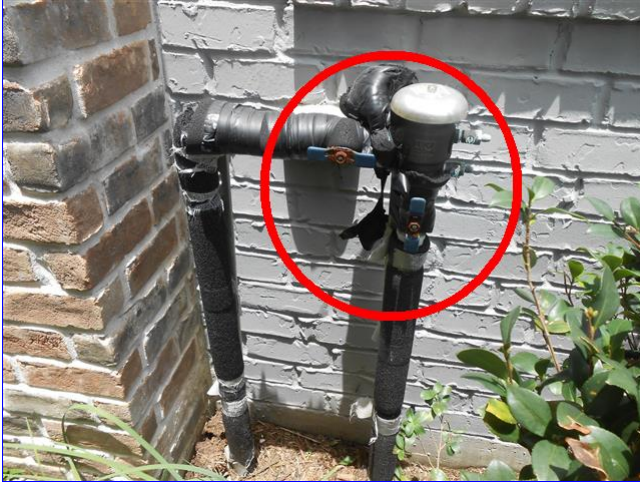
A. Item 1(Picture) View of the sprinkler system anti back flow device.
