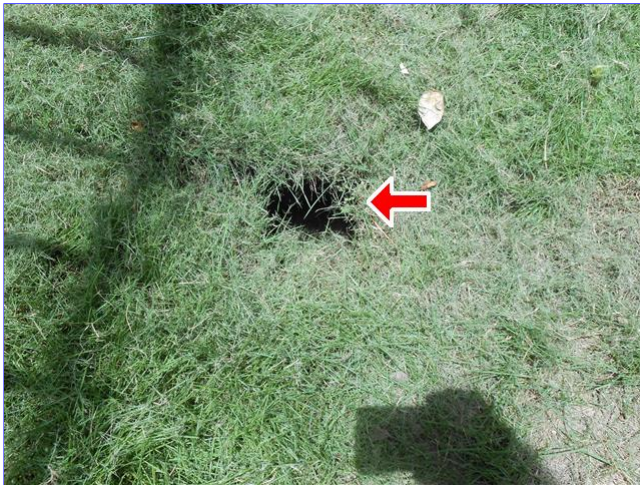
B. Item 1(Picture) Drain needs grate
