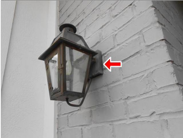
E. Item 1(Picture) This area needs to be sealed to the wall to prevent moisture and pest intrusion into the wall.
