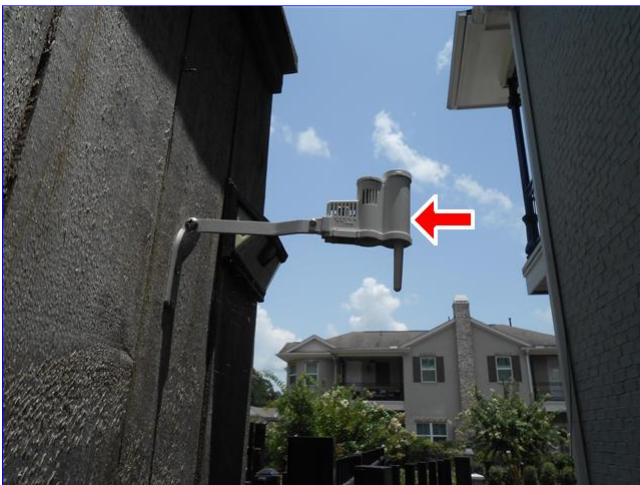
A. Item 3(Picture) View of the sprinkler system rain /moisture sensor.
