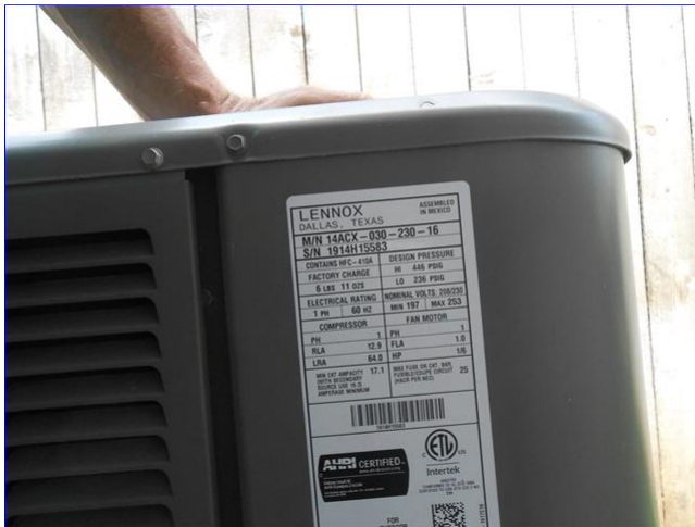
B. Item 2(Picture) View of the second floor cooling condenser information label
