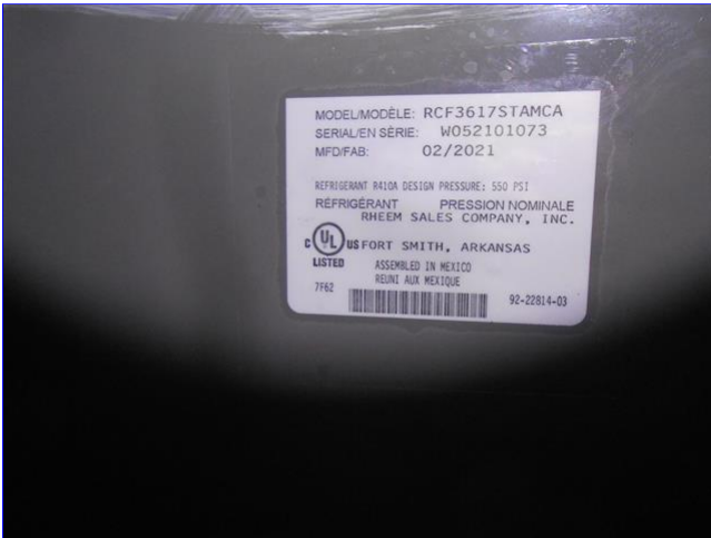
B. Item 8(Picture) View of the second floor cooling system evaporator information label
