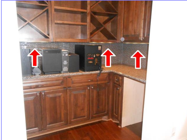
B. Item 1(Picture) No power at outlets
