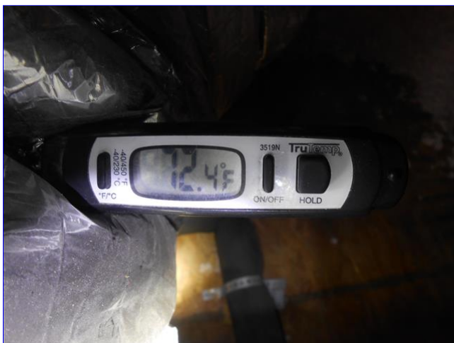
B. Item 6(Picture) View of the second floor cooling system measured return air temperature at the evaporator.
