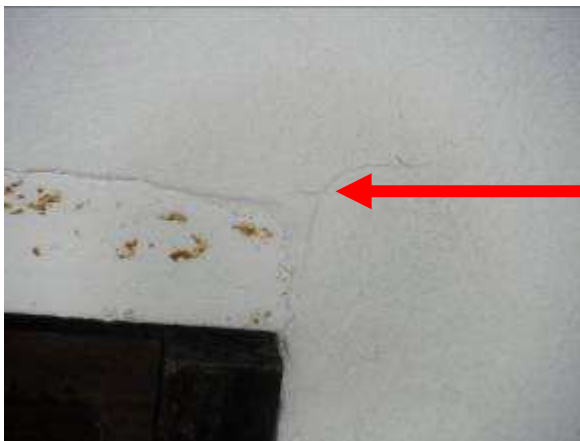
Crack and visible rust
