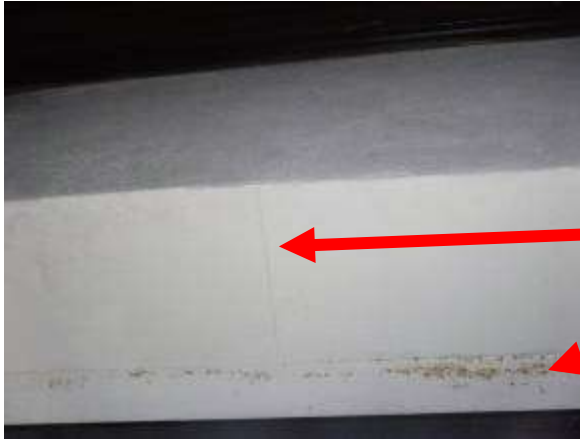
Crack and visible rust
