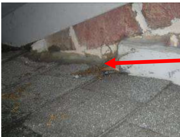
Roof section covered with caulk
