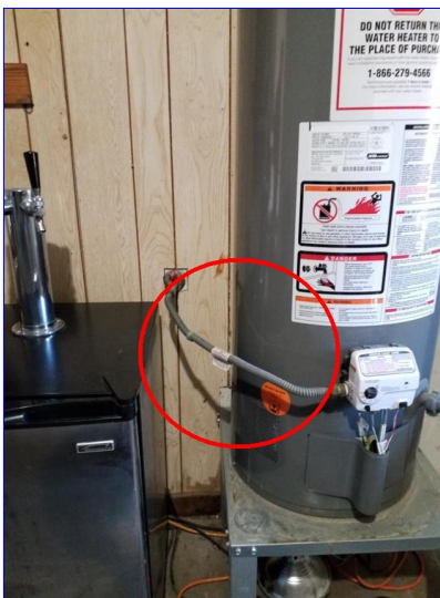
C. Item 2(Picture) Water heater
