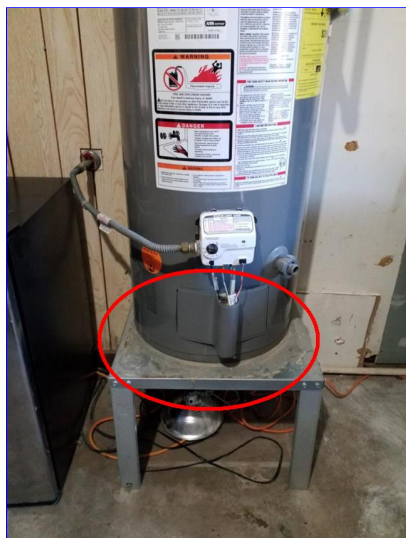
C. Item 3(Picture) Water heater
