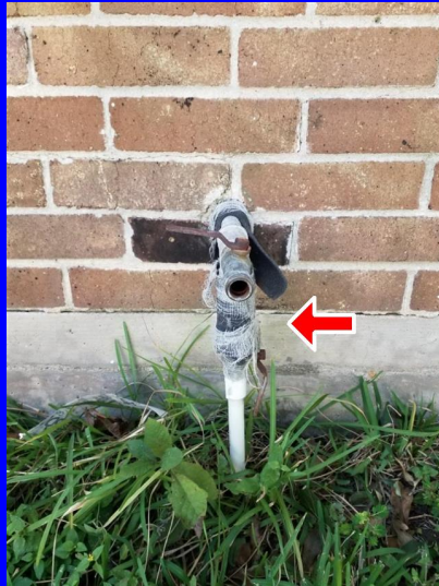
Water main shutoff, located front left side of home
