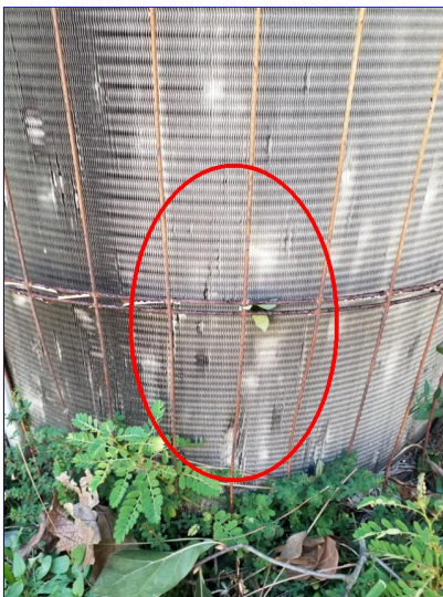
B. Item 4(Picture) HVAC condenser
