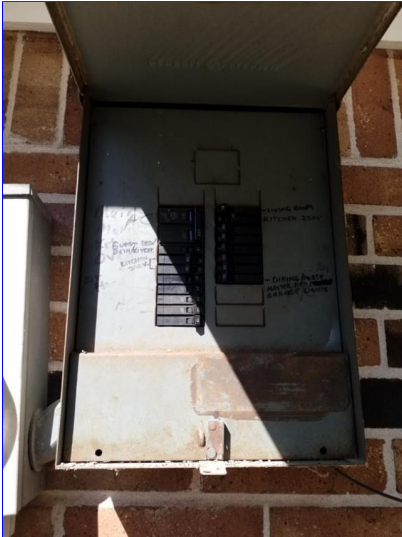
A. Item 1(Picture) Main service panel
