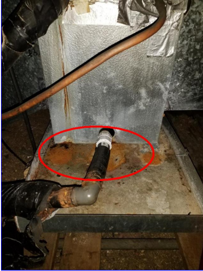
B. Item 7(Picture) Overflow drain pan
