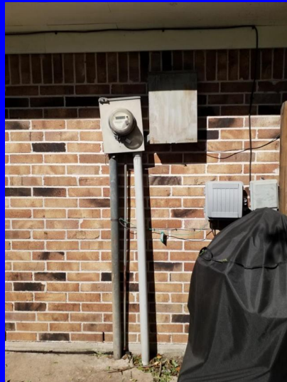
Underground service, located rear of home
