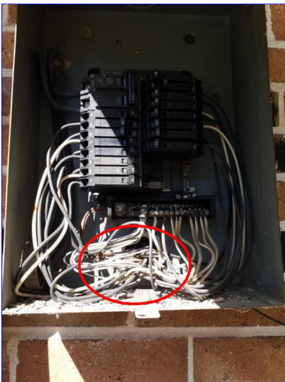
A. Item 2(Picture) Main service panel
