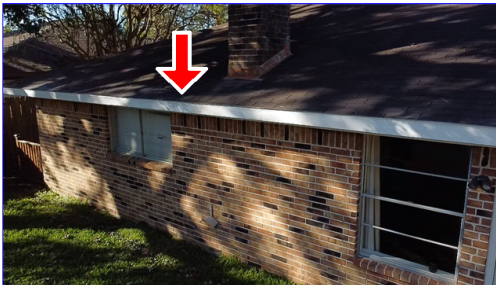
B. Item 2(Picture) Add gutters
