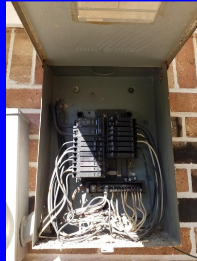
100 AMP main service panel, located outside, rear of home
