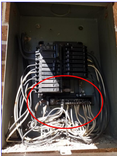
B. Item 2(Picture) Main service panel
