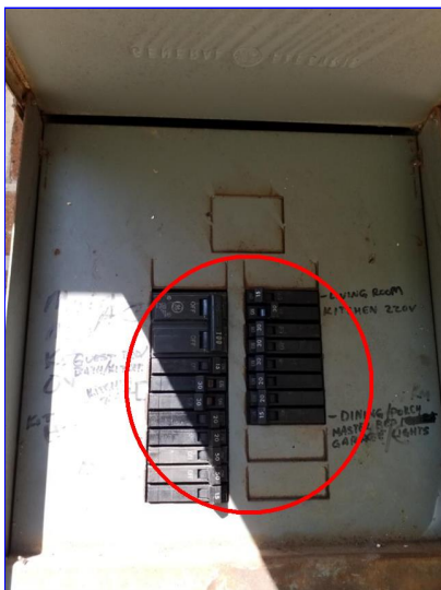
B. Item 1(Picture) Main service panel
