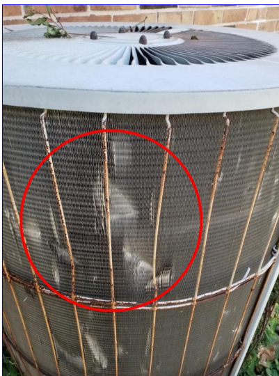
B. Item 6(Picture) HVAC condenser
