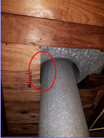
C. Item 1(Picture) Vent for gas furnace
