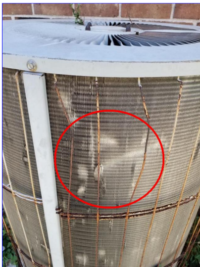
B. Item 5(Picture) HVAC condenser
