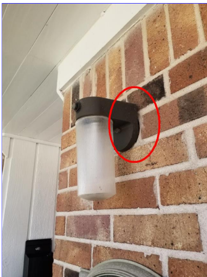
E. Item 1(Picture) Front of home
