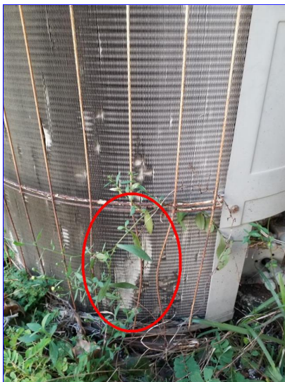
B. Item 3(Picture) HVAC condenser
