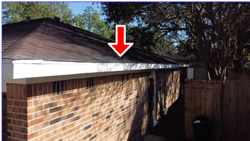
B. Item 1(Picture) Add gutters
