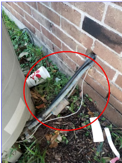
B. Item 2(Picture) Missing insulation
