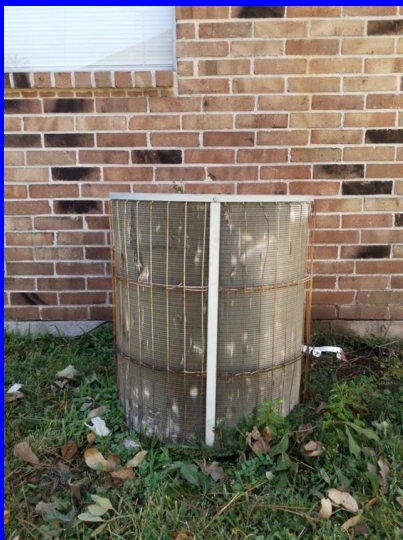
HVAC outside condenser
