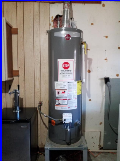
40 gallon gas water heater, located in the garage
