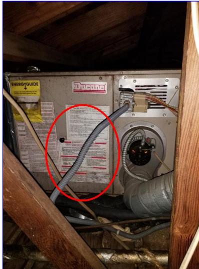
A. Item 3(Picture) Gas furnace
