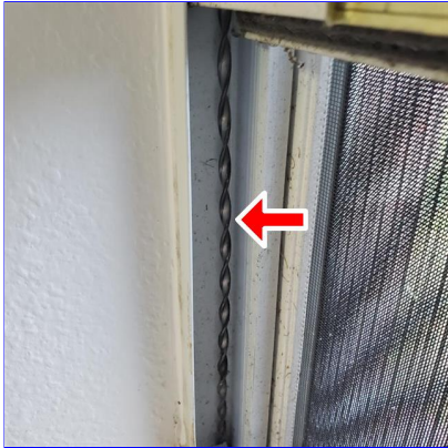
H. Item 1(Picture) Damaged spiral balances on the East breakfast nook window
