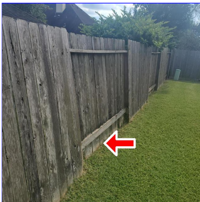
L. Item 3(Picture) The fence is leaning in the back yard and boards are starting to degrade and rot at the bottom of the fence in several areas
