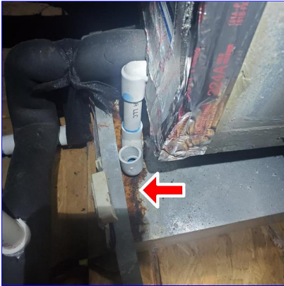
B. Item 3(Picture) Rust in the secondary drain pan at time of inspection
