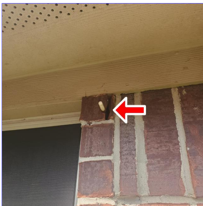
E. Item 5(Picture) Damaged brick at the top of the third window at the south side of the home
