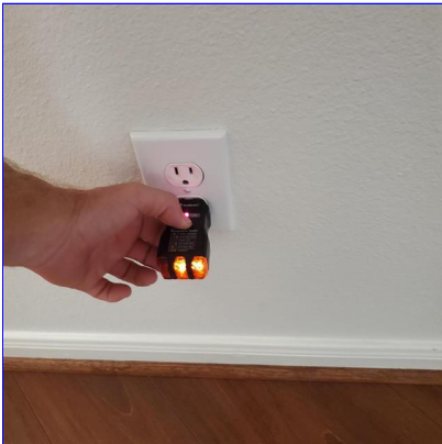
B. Item 3(Picture) Electrical receptacles within six feet of the kitchen sink on the back of the kitchen counter would not trip when tested and needs repair for safety
