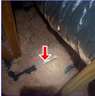
B. Item 4(Picture) Missing insulation on condensate line in the attic, approximately above the hallway bathroom, can cause line to condensate
