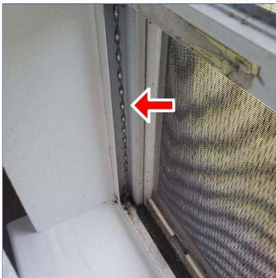
H. Item 3(Picture) Damaged spiral balance on North window on the East wall of the master bedroom
