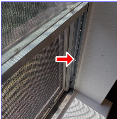
H. Item 4(Picture) Damaged spiral balance on window in the office/den area across in the hallway bathroom
