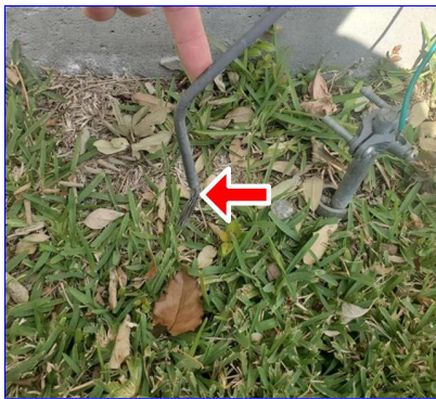
A. Item 1(Picture) Ground wire is loose from the grounding rod at the meter base and needs repair
