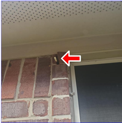
E. Item 3(Picture) Damaged brick at the top left corner of the first window at the south side of the home
