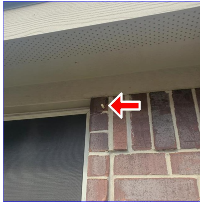
E. Item 4(Picture) Damaged brick above the second window at the south side of the home
