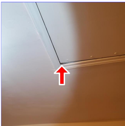
D. Item 1(Picture) Gap around the attic access in the garage be evaluated and repaired, as needed
