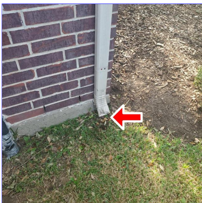
B. Item 7(Picture) Damaged gutter downspout and missing splash block at the northwest corner of the home
