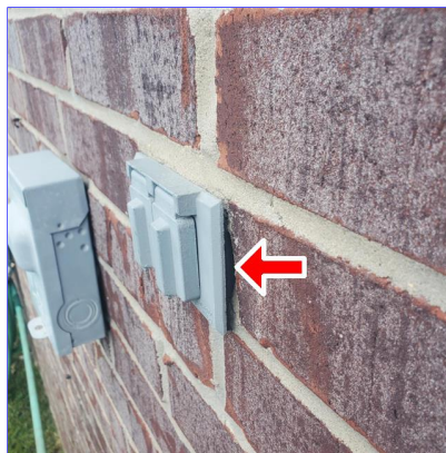
E. Item 6(Picture) Gap around electrical receptacle above the AC condenser should be sealed to help prevent water from entering this area
