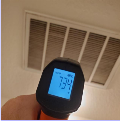
B. Item 1(Picture) Return air temperature was approximately 73 degrees. There should be a 14-22-degree drop between return and supply air temperature
