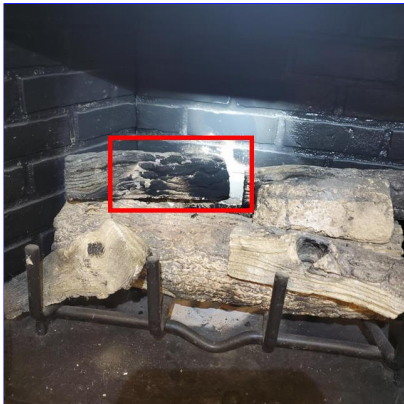
J. Item 1(Picture) Black soot on fire logs
