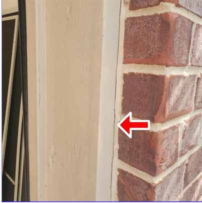
E. Item 1(Picture) Small gap in sealant around garage door trim
