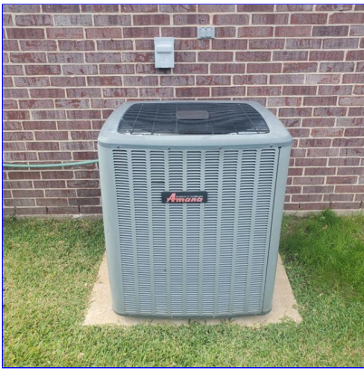
B. Item 5(Picture) General view of Amana AC
