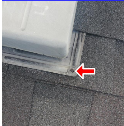
C. Item 2(Picture) Exposed nail on vent flashing on the left facet of the roof
