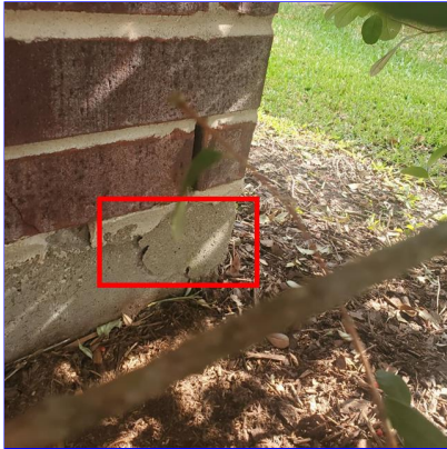
A. Item 1(Picture) Corner pop in the foundation at the South West corner of the home
