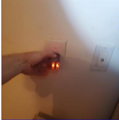
B. Item 6(Picture) Electrical receptacle on the South Wall of the garage is not GFCI protected and is not labeled as a non GFCI receptacle. This is a possible shock hazard
