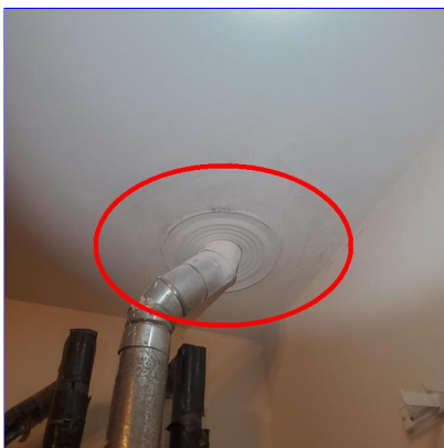
F. Item 3(Picture) Stain on the garage ceiling around the water heater flue pipe
