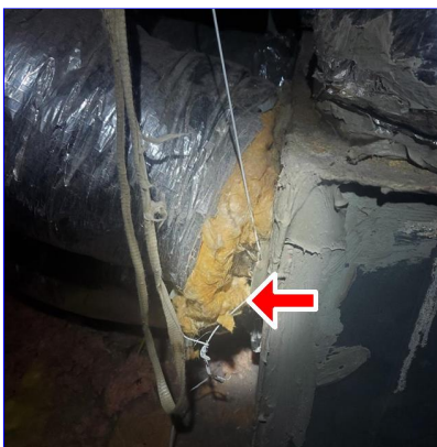
C. Item 2(Picture) Duct loose from the supply plenum
