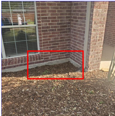
B. Item 6(Picture) rea for potential ponding water at the front of the home to the right of the front door
