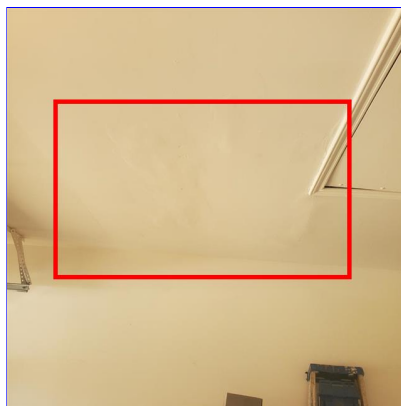
F. Item 4(Picture) Hairline crack and previous repair noted to ceiling in the garage
