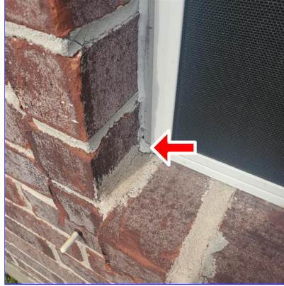
E. Item 2(Picture) Small gap in sealant at the bottom left corner of the first window at the south side of the home. This was noted that a few Windows around the home
