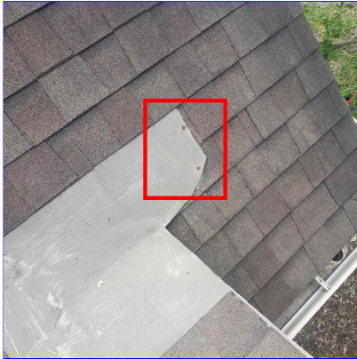
C. Item 1(Picture) Exposed nails on flashing at the front of the home
