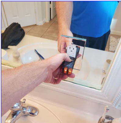
B. Item 4(Picture) None of the electrical receptacles in the master bathroom would trip when tested and need repair for safety
