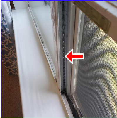
H. Item 2(Picture) Damaged spiral balance on the far south window on the East wall in the master bedroom
