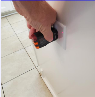
B. Item 2(Picture) Electrical receptacle on the kitchen island would not trip when tested and needs repair to help prevent possible shock hazard
