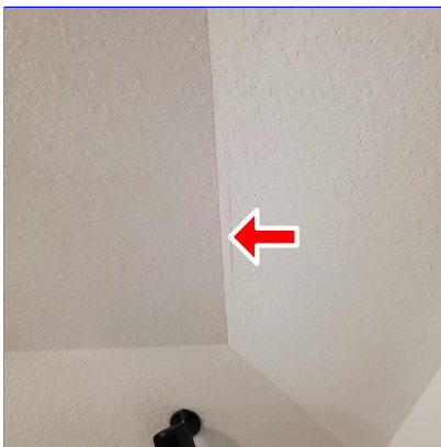
F. Item 1(Picture) Appears to be cosmetic damage to ceiling at the northeast corner of the living room
