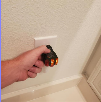
B. Item 5(Picture) Electrical receptacles in the hallway bathroom would not trip when tested
