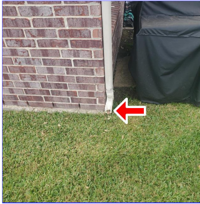
B. Item 2(Picture) Damaged elbow on downspout at the northeast corner of the home and missing splash block
