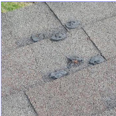
C. Item 3(Picture) Exposed lag bolts on back facet of roof appear to be from a satellite dish and are areas for potential roof leaks. There were two places this was noted at the back of the home.
