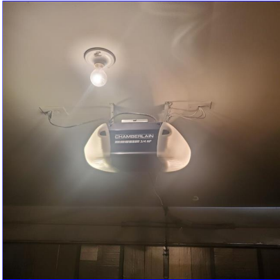
G. Item 1(Picture) General view of Chamberlain garage door operator
