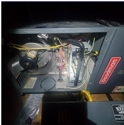
A. Item 3(Picture) General view of Goodman gas furnace.
