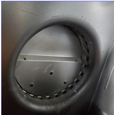
J. Item 2(Picture) Missing damper clamp on flue damper
