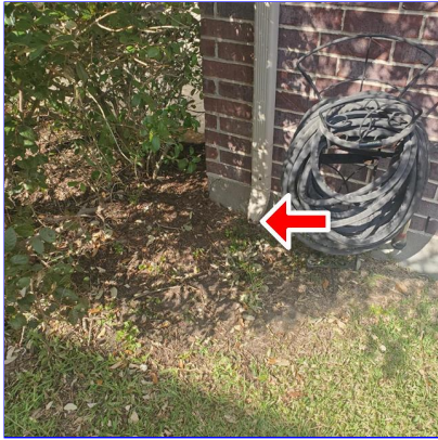
B. Item 1(Picture) Missing splash block at the southwest corner of the home
