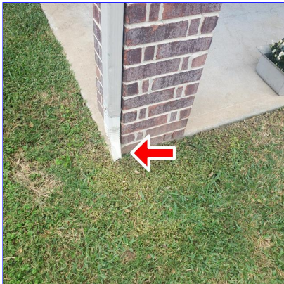
B. Item 5(Picture) Damaged gutter downspout and missing splash block at the back patio
