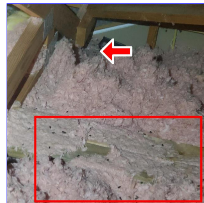
L. Item 2(Picture) Droppings and trails through insulation in the attic indicate possible critters or pests in the attic
