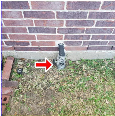
A. Item 1(Picture) Main water shut-off is at the left side of the home near the front of the home
