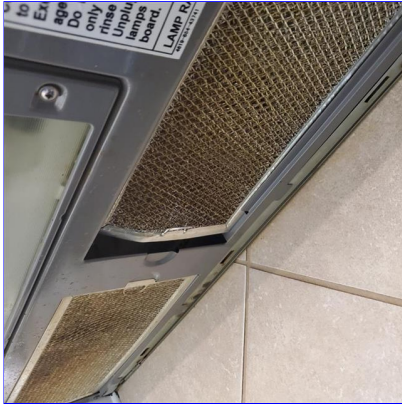
D. Item 1(Picture) Damaged filter on the range exhaust
