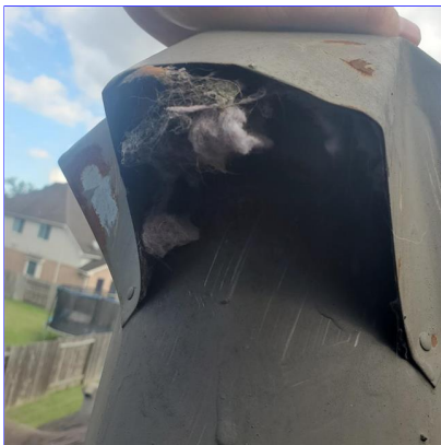
H. Item 3(Picture) Rooftop dryer exhaust vent is filled with debris
