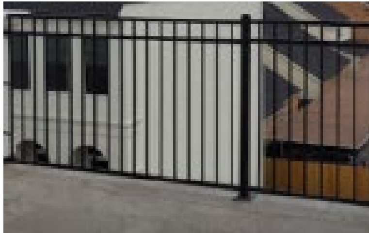
Balcony & Roof Deck Railing
