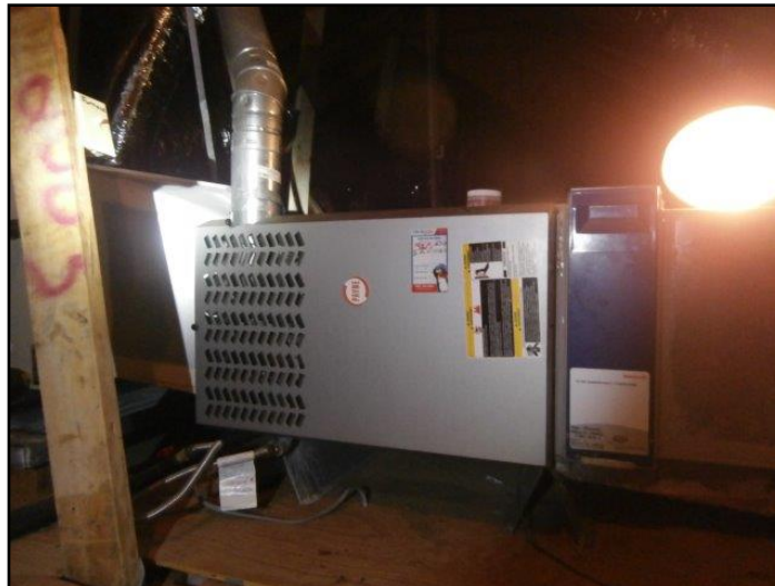
General view of heating system.
