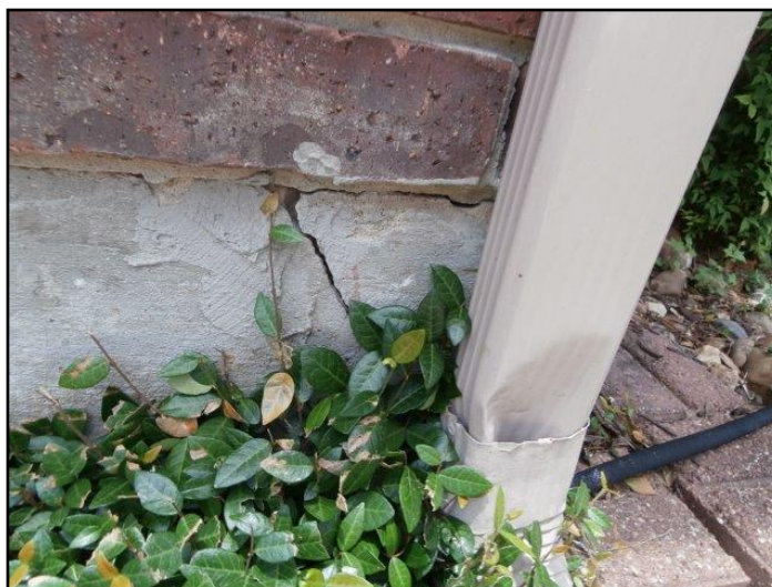
Note: Shear cracking ("corner pops")...
