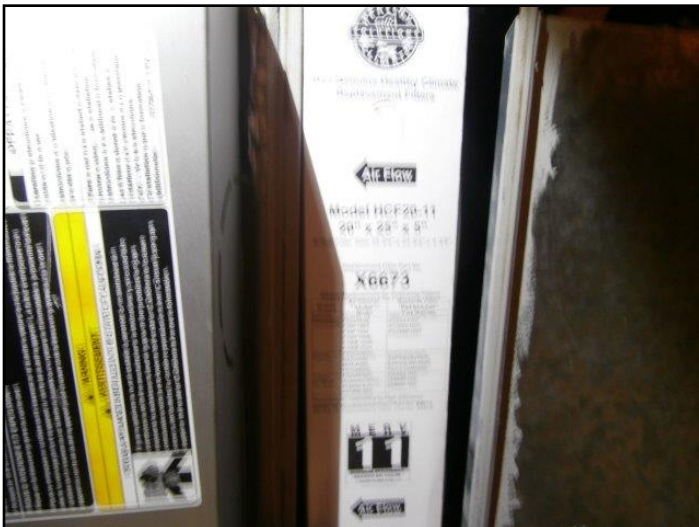
Note: Media filter is located at the HVAC...
