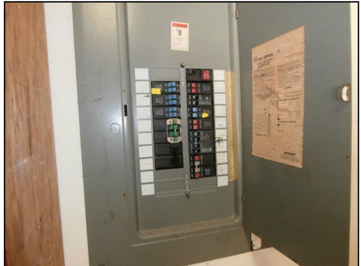
General view of electrical panel(s).
