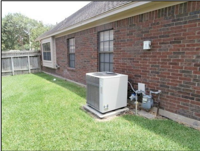
General view of air conditioning equipment
