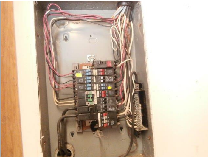
General view of electrical panel(s).
