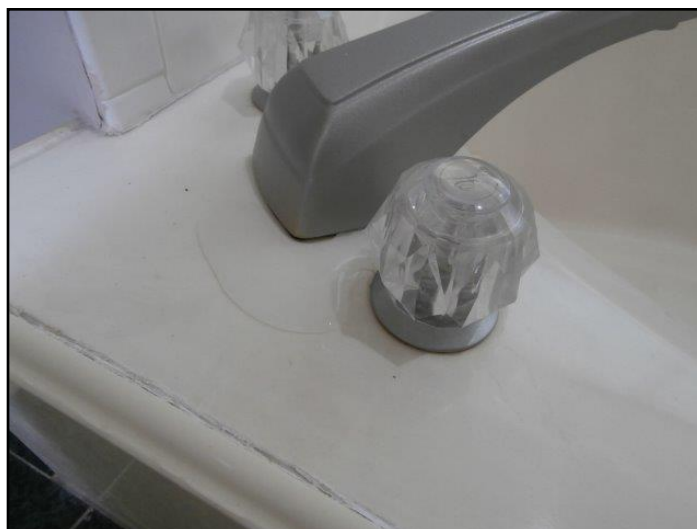
Leaking faucet stem
