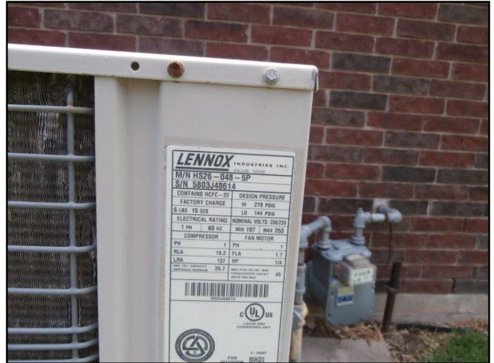
General view of air conditioning equipment
