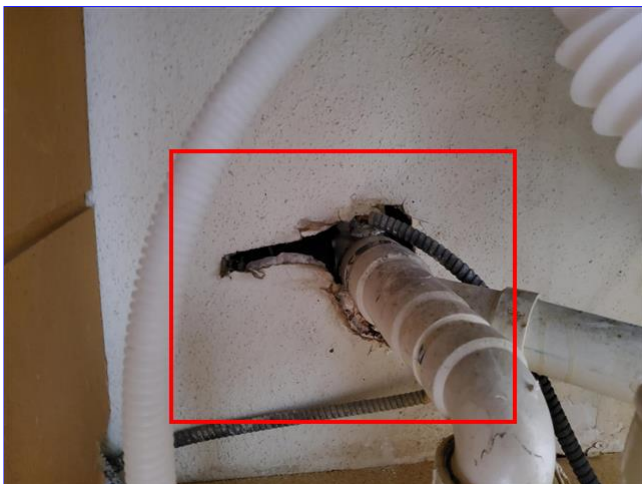
E. Item 1 (Picture) Under kitchen sink
