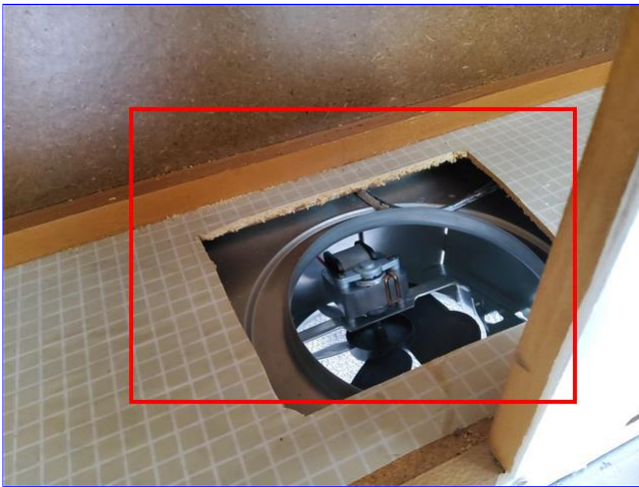
C. Item 1 (Picture) Vent discharges directly into cabinet.
