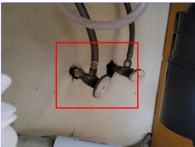
E. Item 2 (Picture) Under kitchen sink
