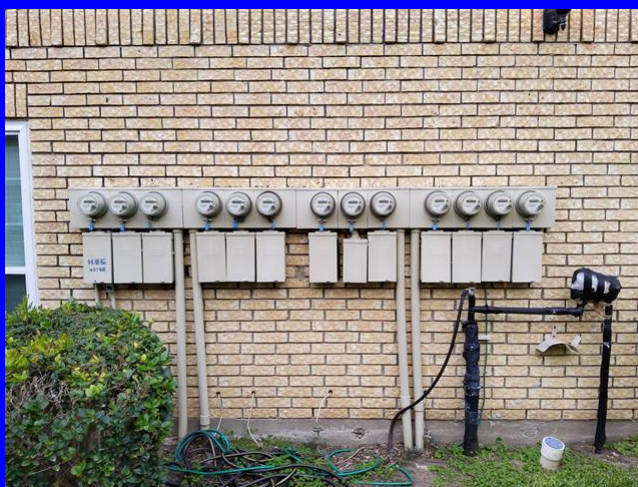
Unable to determine which main disconnect and electric meter are for the unit.
