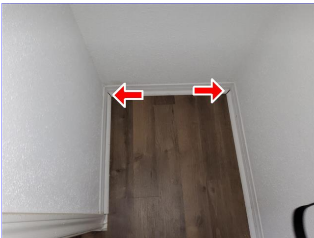
E. Item 5 (Picture) Trim installed unprofessionally throughout
