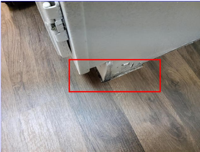
F. Item 6 (Picture) Gaps between flooring and cabinets
