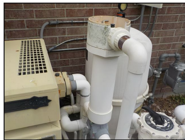
Chlorinator / Salt Cell
