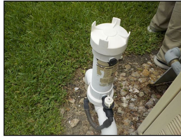
Chlorinator / Salt Cell
