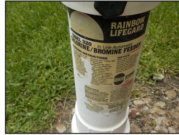
Chlorinator / Salt Cell data plate
