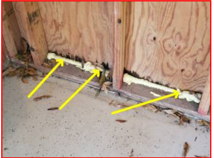
Stain noticed at the bottom of the garage walls.
