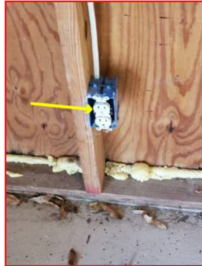
Outlet(s) cover missing or damaged.
