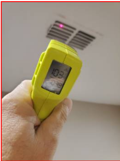
Heater supply temp 103 degrees.
