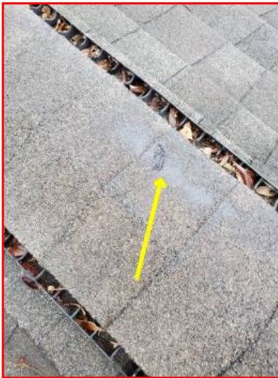
Damaged or missing shingles
