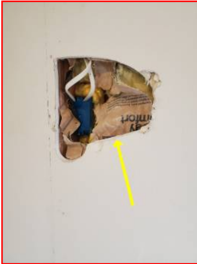
Damaged areas noted
