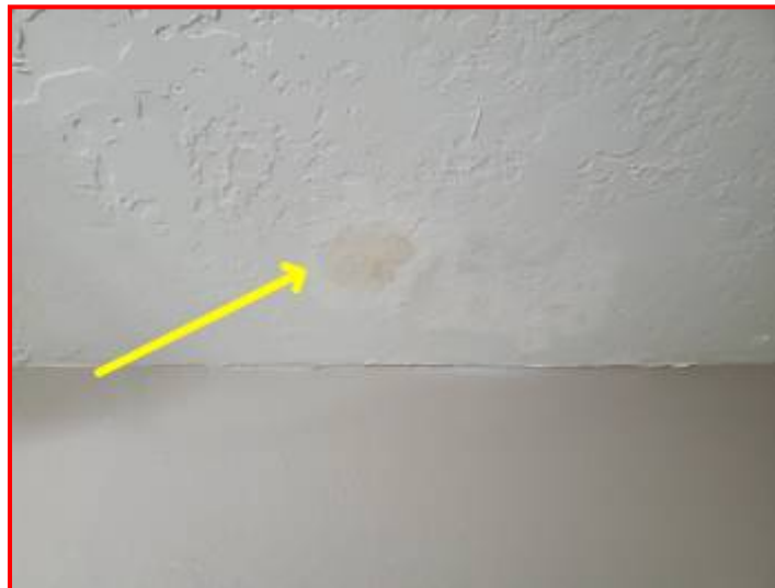
Water or liquid stain noted in one or more ares.
