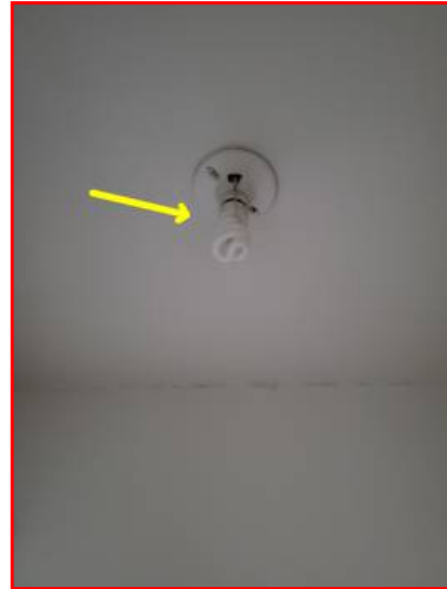
Pull cord missing. Couldn't check light.
