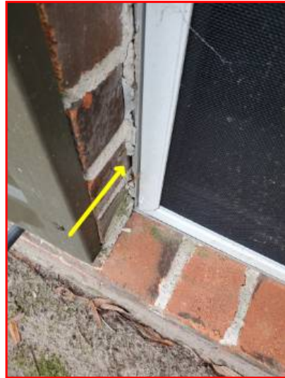
Windows need caulking.
