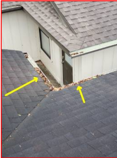
Gutter(s) need cleaning.
