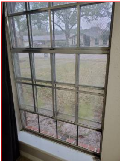
Window(s) would not fully open.
