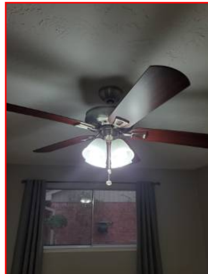
Ceiling fan(s) not working at time of the inspection
