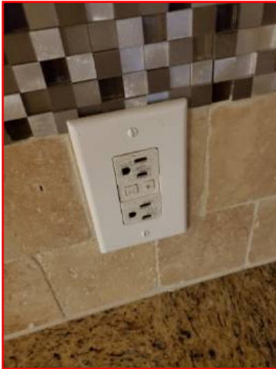
GFCI receptacles not working.
