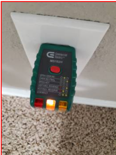
Open ground(s) noticed at one or more locations around the home.
