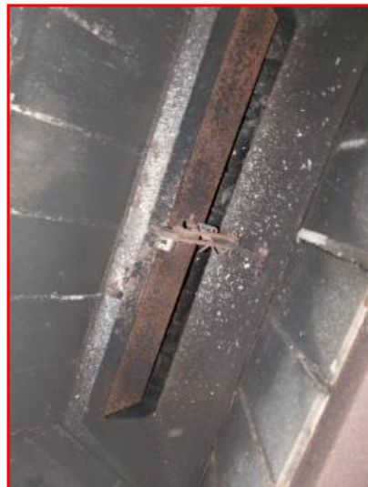
Damper doesn't work.
