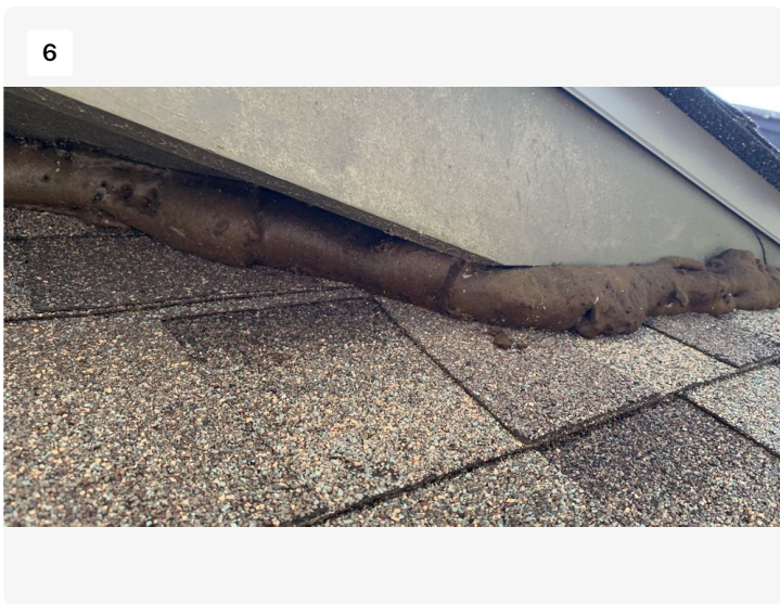
Foam and Wire mesh between soffit and shingle. We are assuming this was to keep an animal out of the attic.
