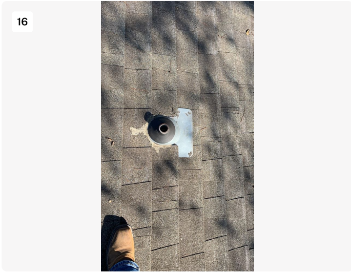
Plumbing Stack with Rubber Boot
