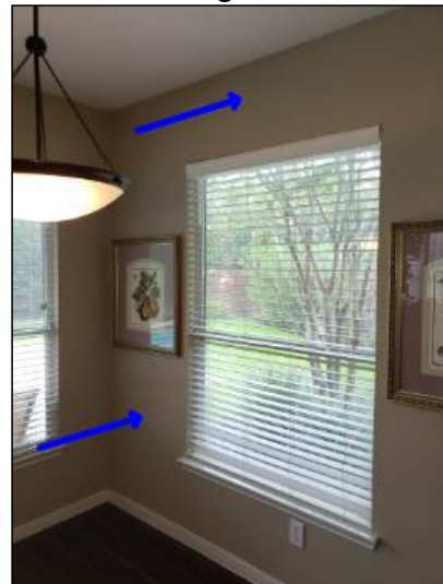
-Previous repairs were noted in the wall. Mainly at - breakfast nook
