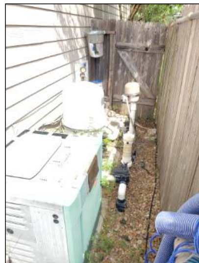
Overview of pool equipment
