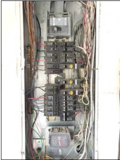
Overview of main electrical panel
