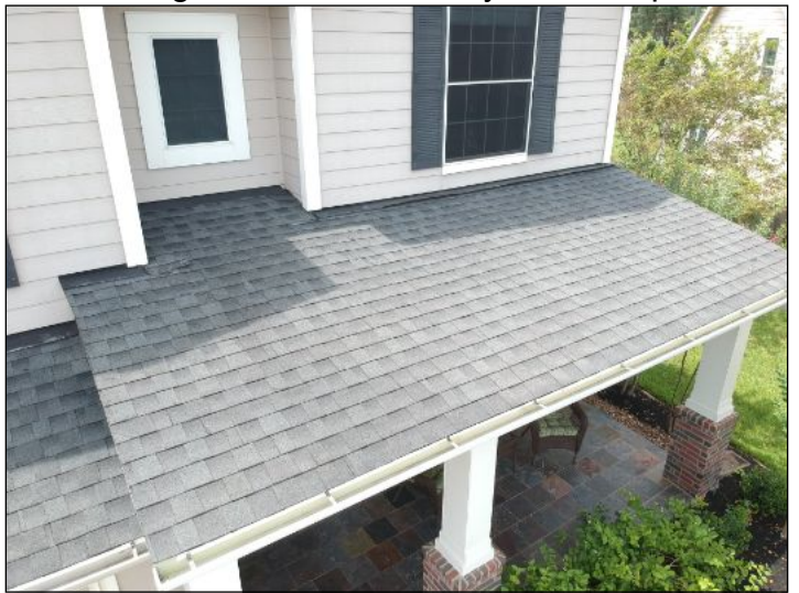
-The roof flashing is lifted. Recommend securing all loose or lifted flashing and sealing nails to help prevent water penetration. Mainly at - patio cover
