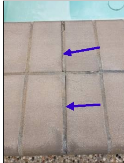
Minor cracks in the coping grout.
