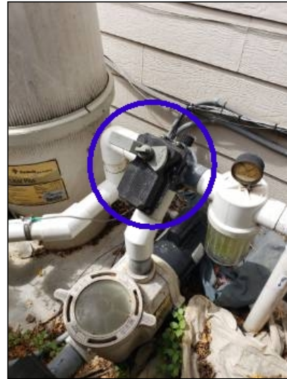
Automatic valve did not move. Its purpose is unknown.
