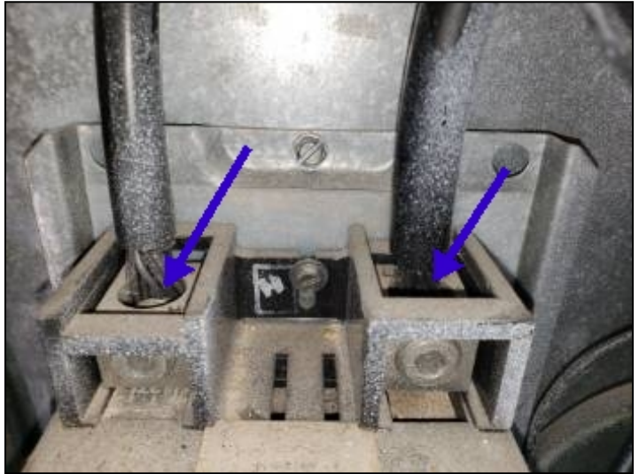
-There is no antioxidant on main aluminum feeds to the panel box. This should be used to help prevent overheating.
