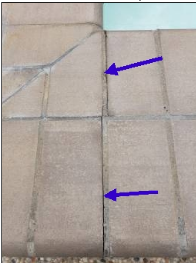
Minor cracks in the coping grout.
