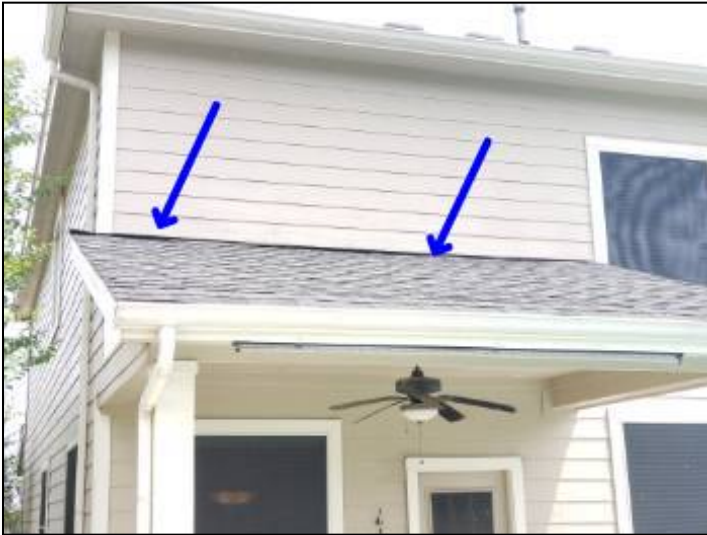
-The roof flashing is lifted. Recommend securing all loose or lifted flashing and sealing nails to help prevent water penetration. Mainly at - patio cover
