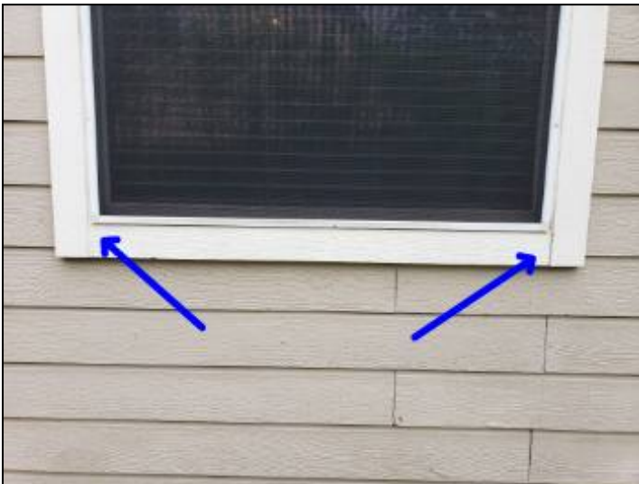
-Recommend sealing trim to help prevent water penetration. Mainly at - right
