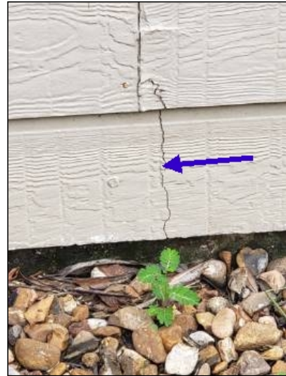
-There is some damage to the exterior siding, recommend repair or replacement to help prevent water penetration. Unable to determine the condition of the underlying materials. Mainly at - right
