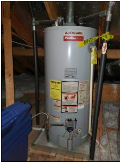
Overview of water heater(s)
