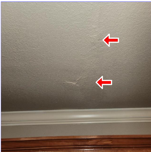
F. Item 5(Picture) Kitchen ceiling
